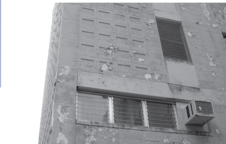
Hale Lulima exterior damage from water leak.
