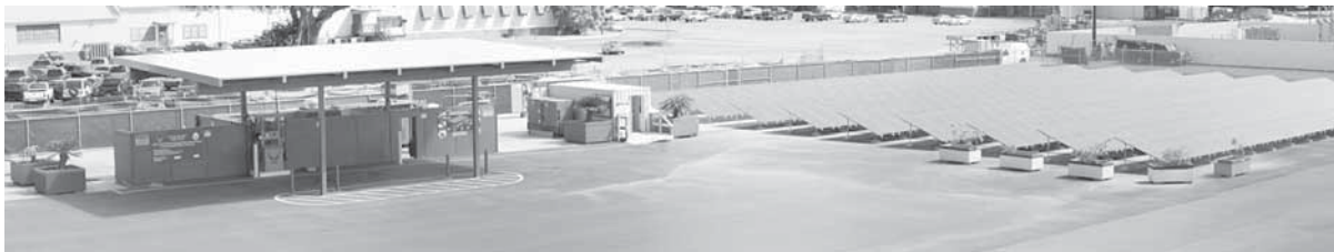
Hydrogen production and fueling station at Hickam AFB powered by 146kW photovoltaic array
