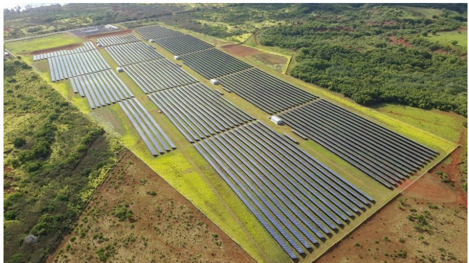
Anahola Solar Project (KIUC)
