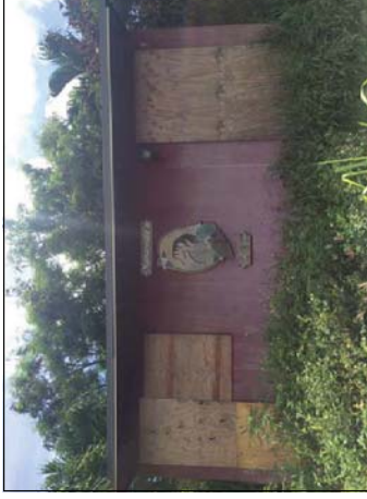
Photograph 25: View of storage shed located within the former Char Ranch tenant space.
