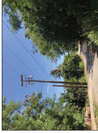
Photograph 38: View of HECO-owned pole-mounted transformers (Transformer Nos. 91805, 91808, 91895) located along Waikupanaha Street.
