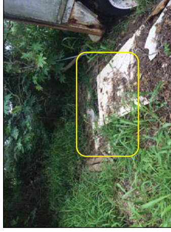
Photograph 17: View of on-site septic system located within the Cook's Ranch tenant space.
