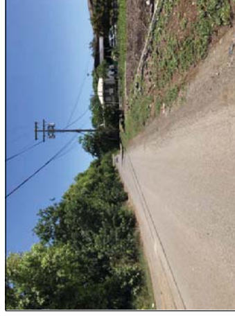
Photograph 39: View of HECO-owned pole-mounted transformers (Transformer Nos. 82645, 82646, 82878) located along Waikupanaha Street.
