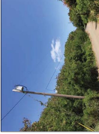
Photograph 37: View of HECO-owned pole-mounted transformer (Transformer No. 80182) located along Waikupanaha Street.
