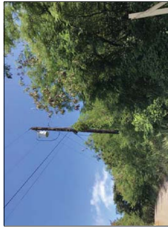
Photograph 36: View of HECO-owned pole-mounted transformer (Transformer No. 48428) located along Waikupanaha Street.
