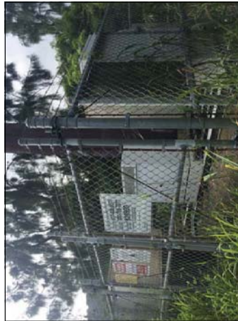
Photograph 9: View of cell phone tower located on the east portion of the Subject Property.
