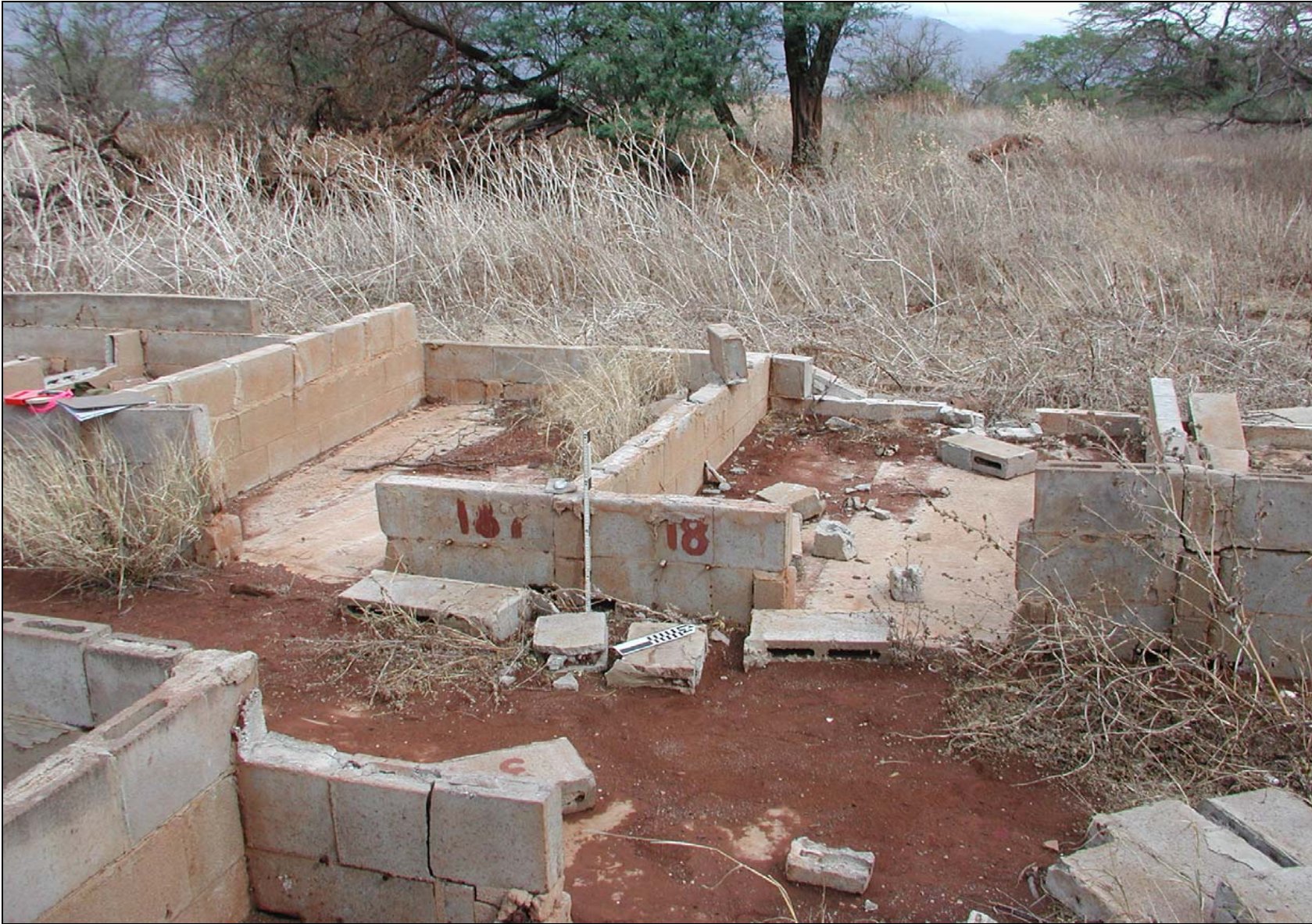
Figure 9: Photograph of SCS Site T-7 Piggery Structure with Rooms. View to Northwest.
