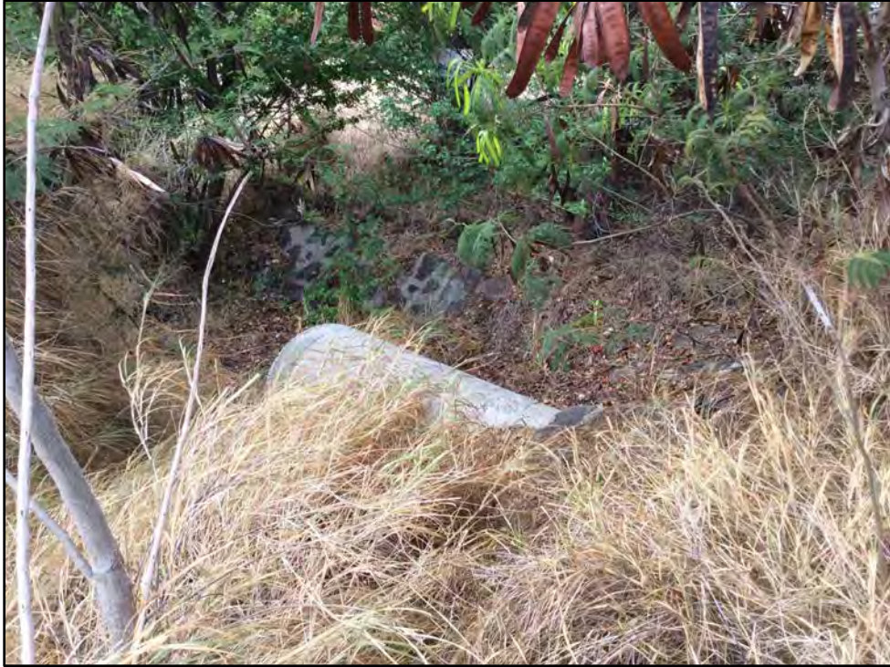
Figure 37. Concrete drainage pipe in concrete and mortared basalt drainage ditch southeast of Fort Barrette Road and Kapolei Parkway intersection, view to south
