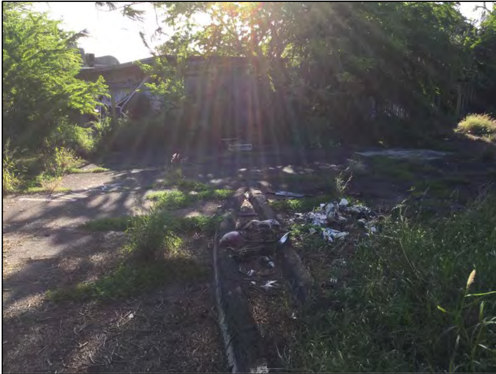
Figure 87. Asphalt surface and asphalt curbs along Wākea Street segment, view to east
