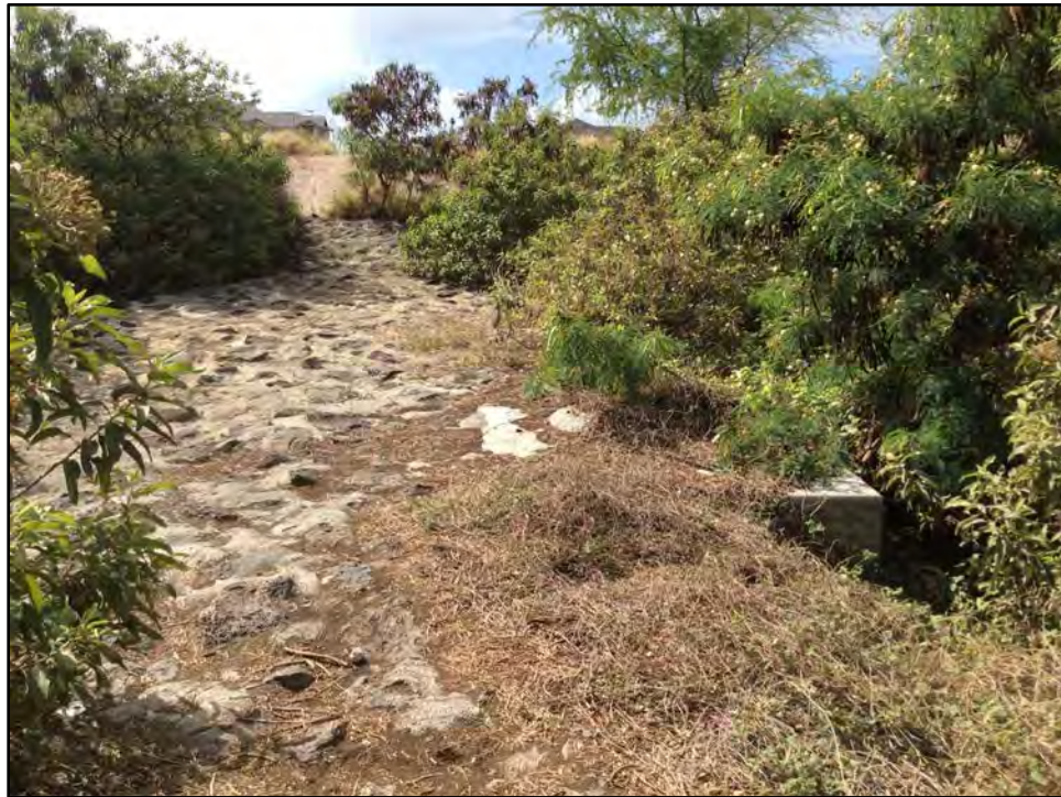
Figure 34. Concrete and mortared basalt drainage ditch with concrete block makai of Kapolei Parkway and Wākea Street intersection, view to south
