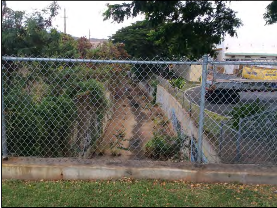
Figure 27. Concrete drainage canal mauka of Kapolei Parkway and east of Kalaeloa Boulevard, view to north
