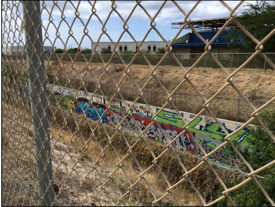
Figure 56. Canal west of unimproved road and fence, along West Perimeter Road segment view to southwest
