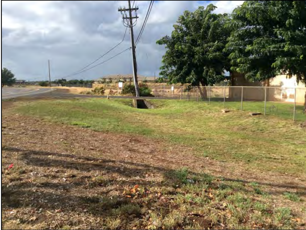
Figure 40. Concrete culvert underneath driveway makai and west of Fort Barrette Road and Kama‘aha Avenue intersection, view to south
