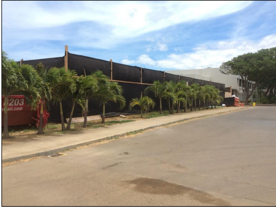
Figure 44. Overview of the construction area behind (west of) the Gym in the northwestern corner of the school campus, view to east
