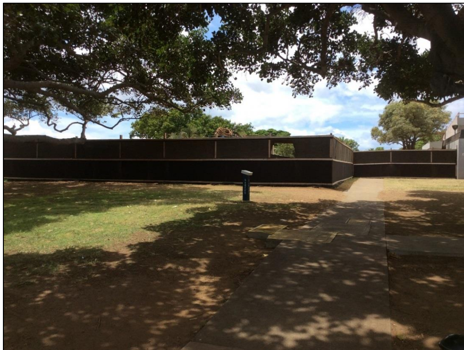
Figure 31. Construction area on the eastern side of the Building J Chorus Room, view to south
