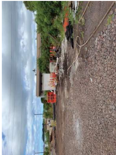
Figure 11. Construction laydown area southwest of the HART field office; orientation is to the southwest. Note the patch of invasive vegetation on the right.
