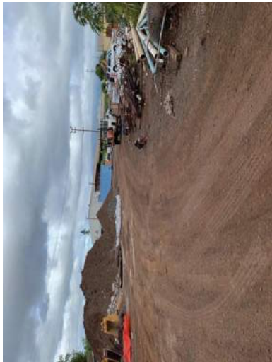
Figure 10. Area makai of the rail entry station, currently used for construction support; orientation is to the west.
