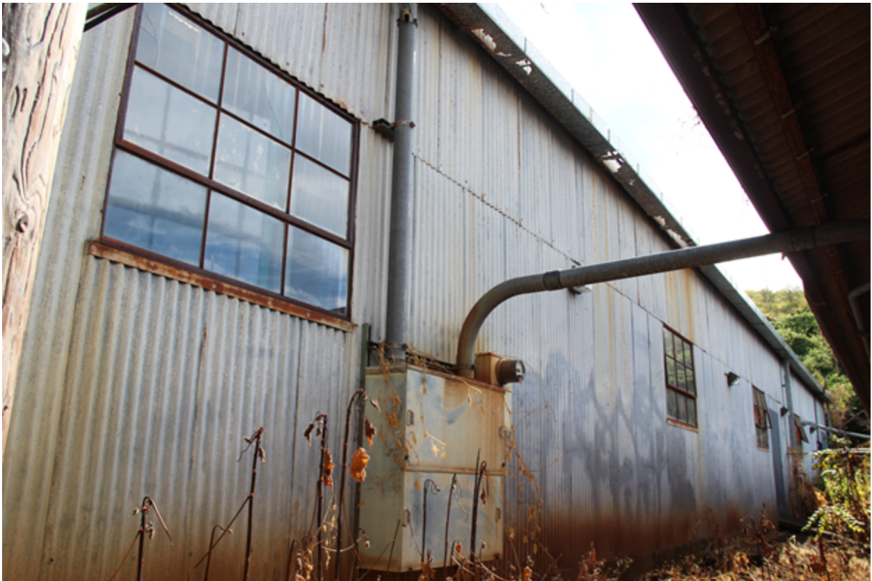
Annex II, south side, showing steel-frame windows and electrical connection to Annex I.
