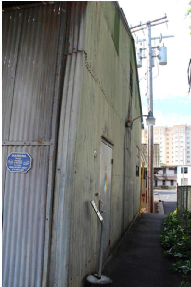
Annex II showing north side sliding vehicular doors with inset personnel door.
