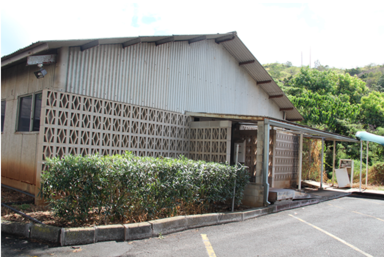
Annex I South end showing main entry with decorative breezeblock walls and entry porch.
