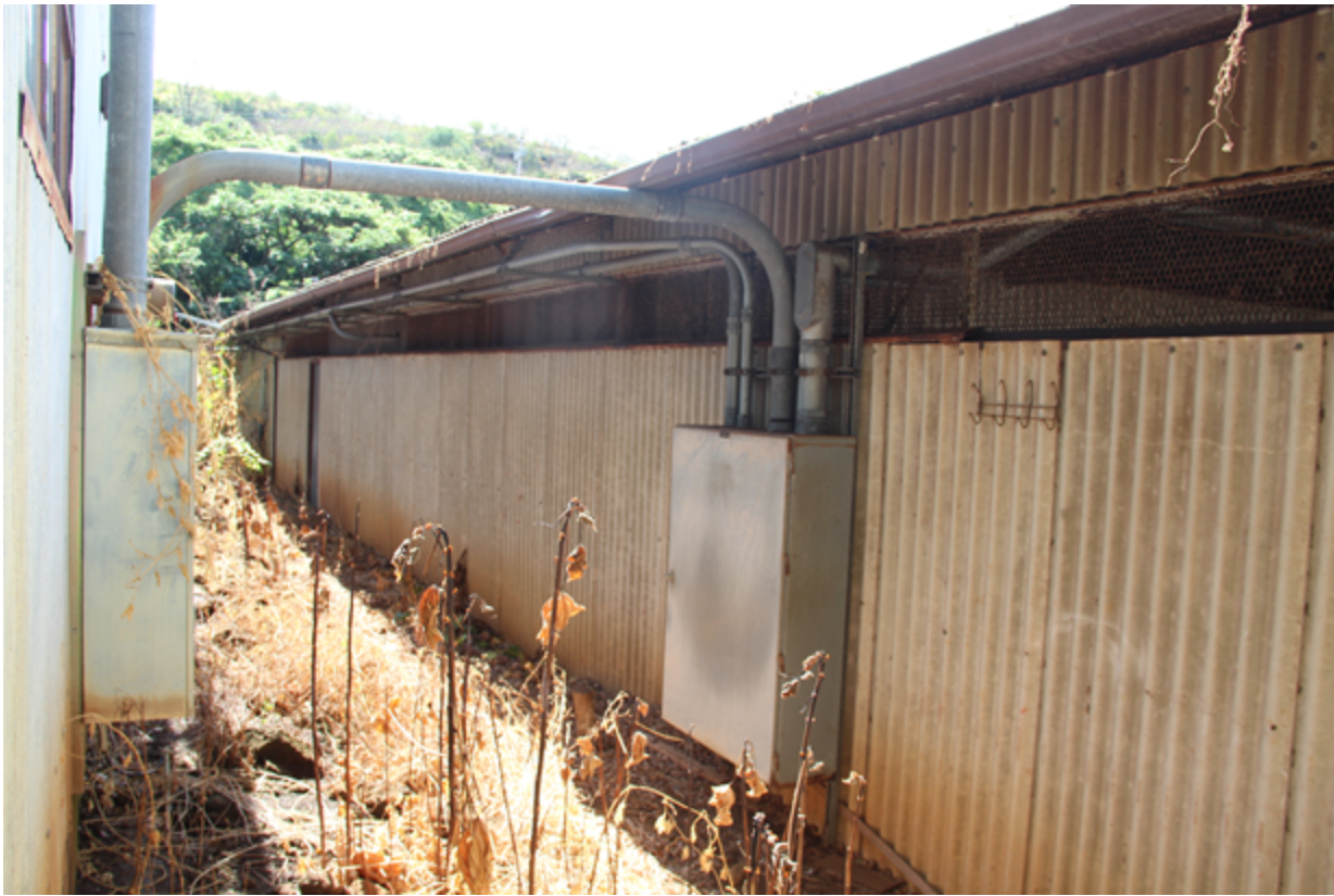
Annex I, north side showing corrugated cement wall panels and screened ventilation strip
