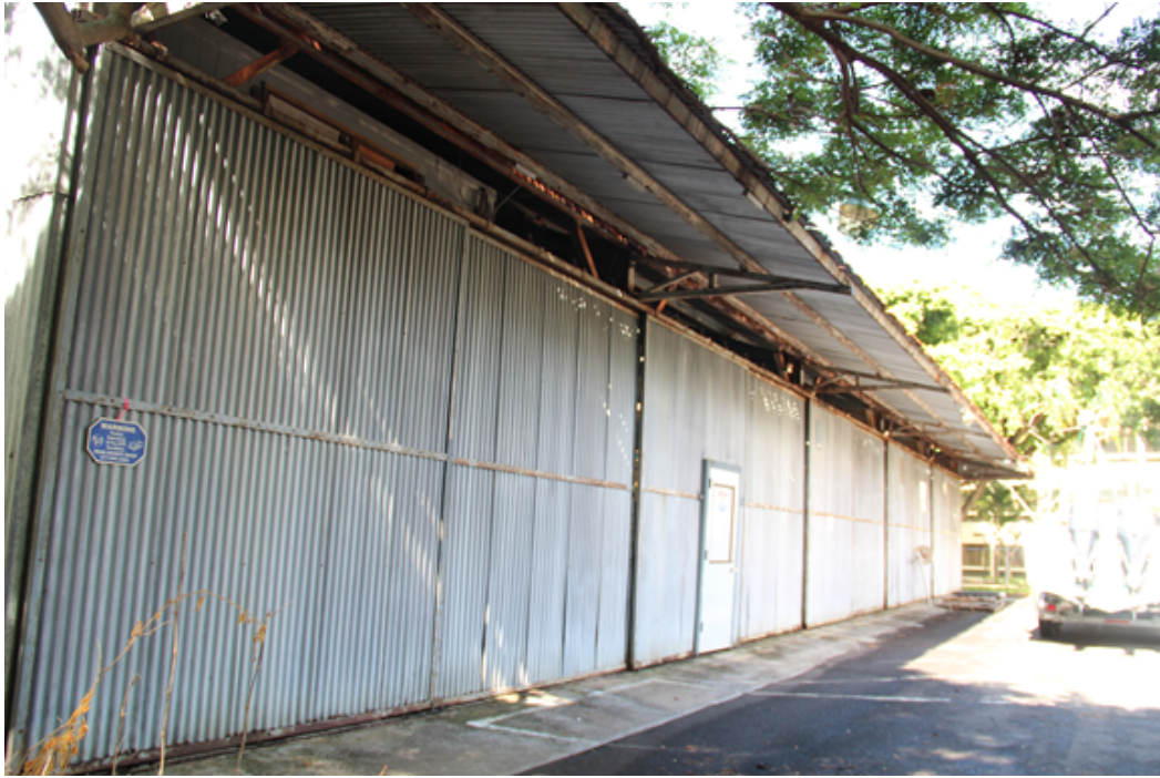
Annex II showing north side sliding vehicular doors with inset personnel door.
