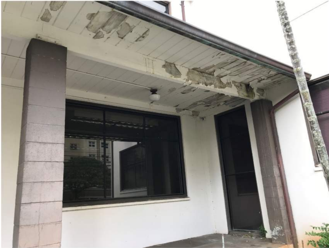
Covered walkway near front entrance with peeling paint. Source: MASON)
