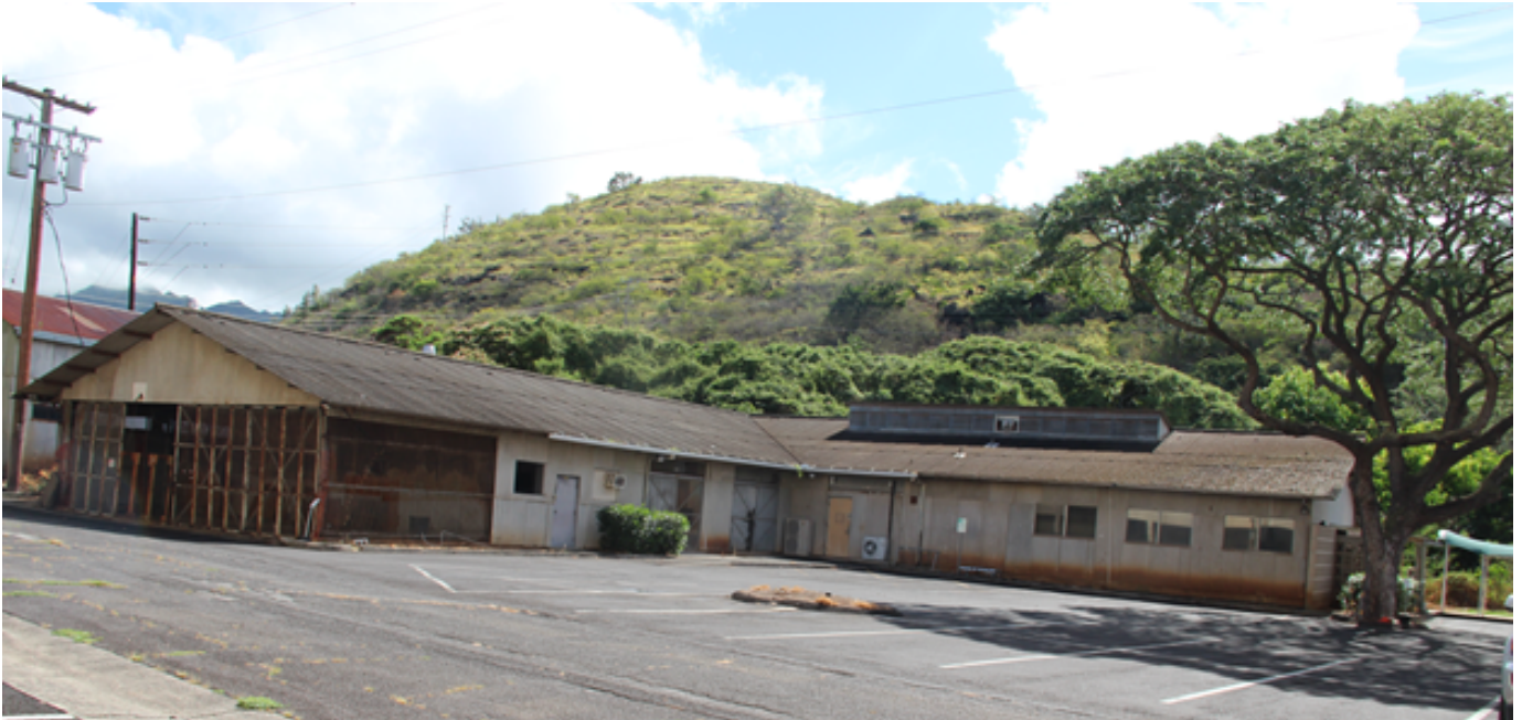
Annex I Southwest sides showing screened west end monitor vents and double screen doors
