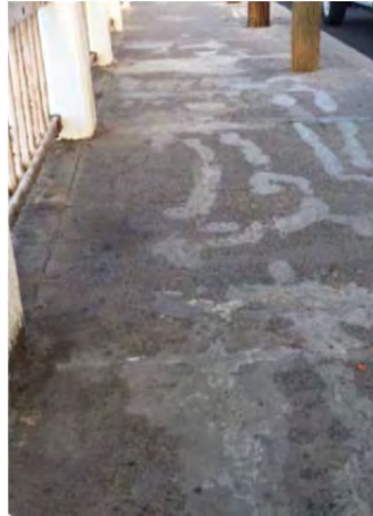
Sidewalk surface defects
