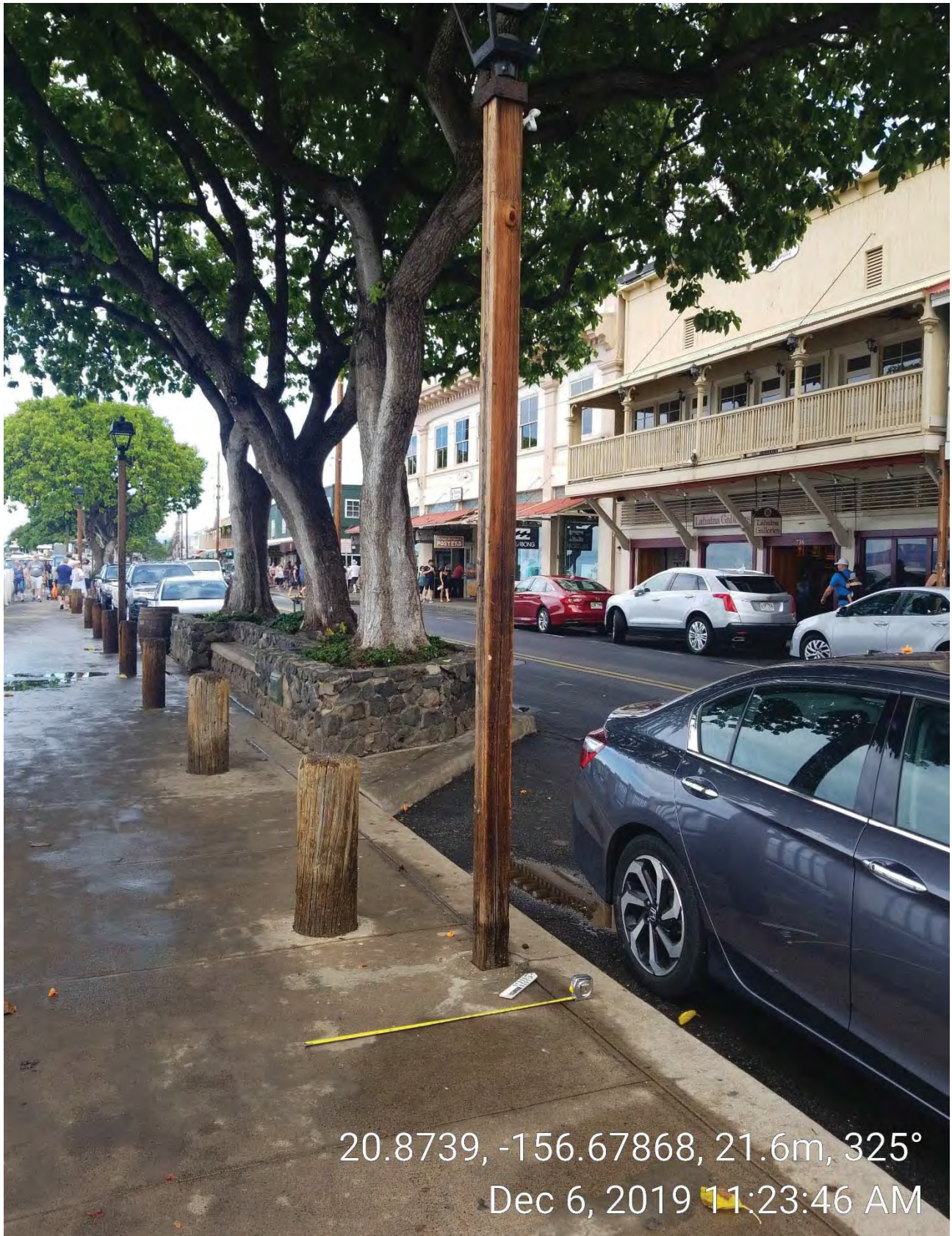
Figure 29: Photographic View of Existing Wood Bollard and Lamp Posts within Area 1. View to Northwest.
