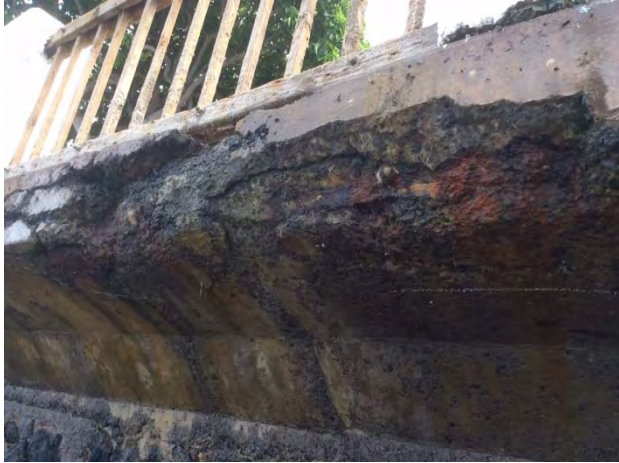
Spalls and corrosion on seawall wave deflector
