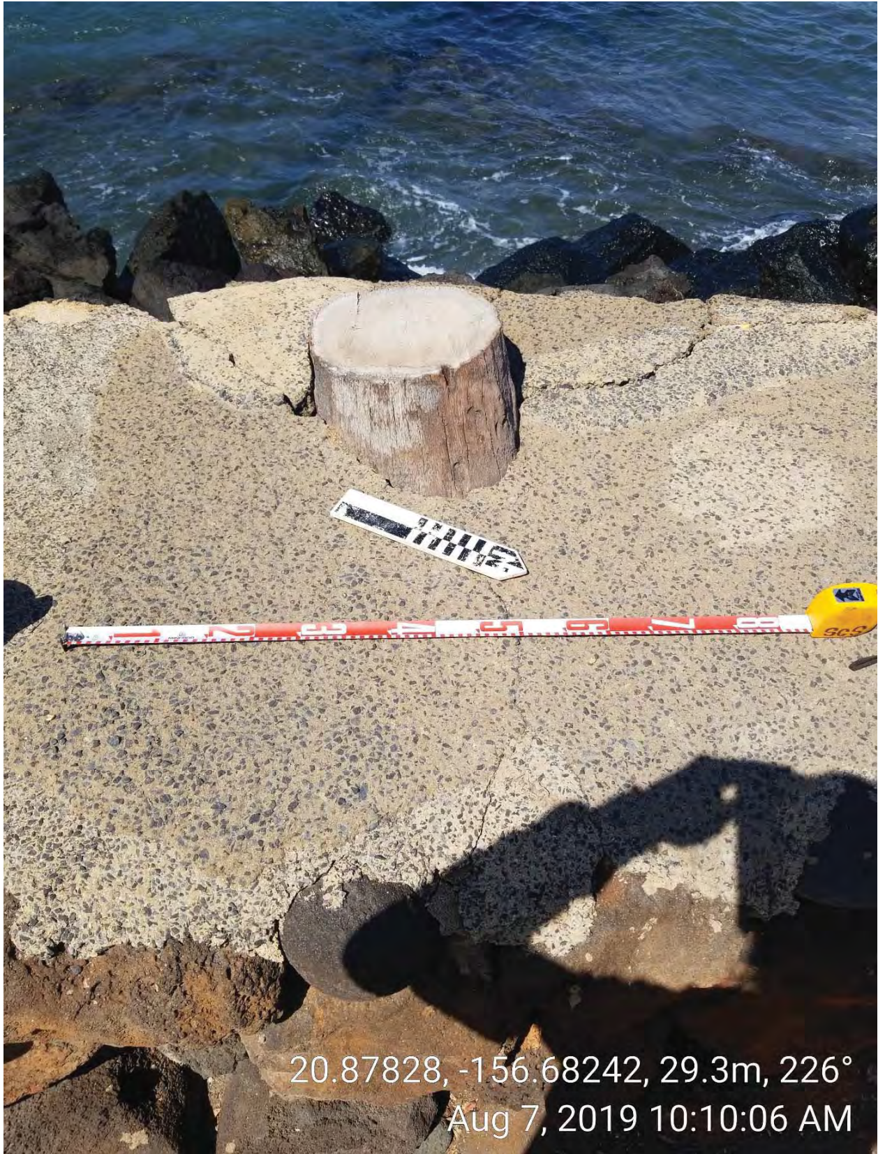
Figure 12: Photographic View of Damaged Wall Adjacent to Sidewalk in Area 2 and the Cut-Off Coconut Palm Tree Stump. View to Southwest.
