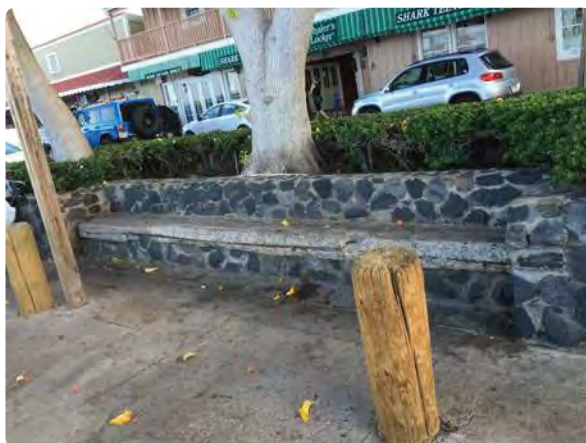
DAMAGED BENCHES & BOLLARDS
