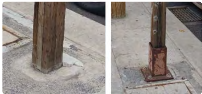
BASES OF WOODEN LIGHT POLES
