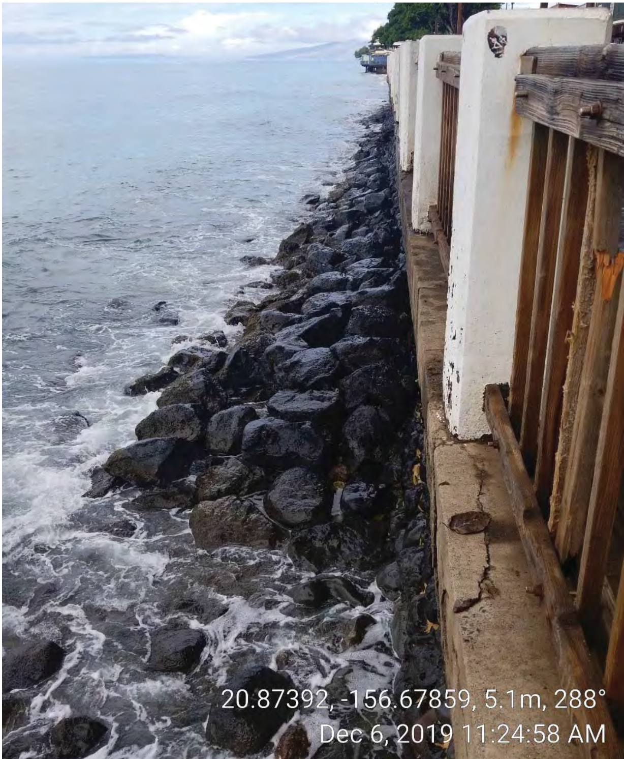
Figure 24: Photographic Overview of the Seawall and Railing within Area 1. View to Northwest.
