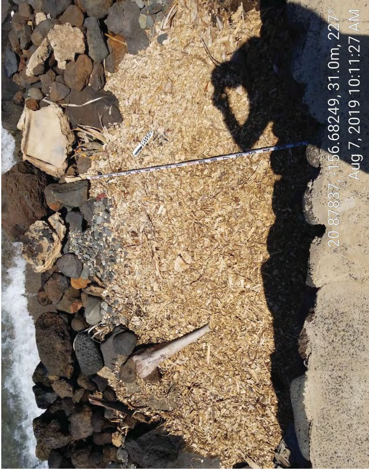
Figure 14: Photographic View of Area of Modifications to the Seawall in Area 2. View to West.
