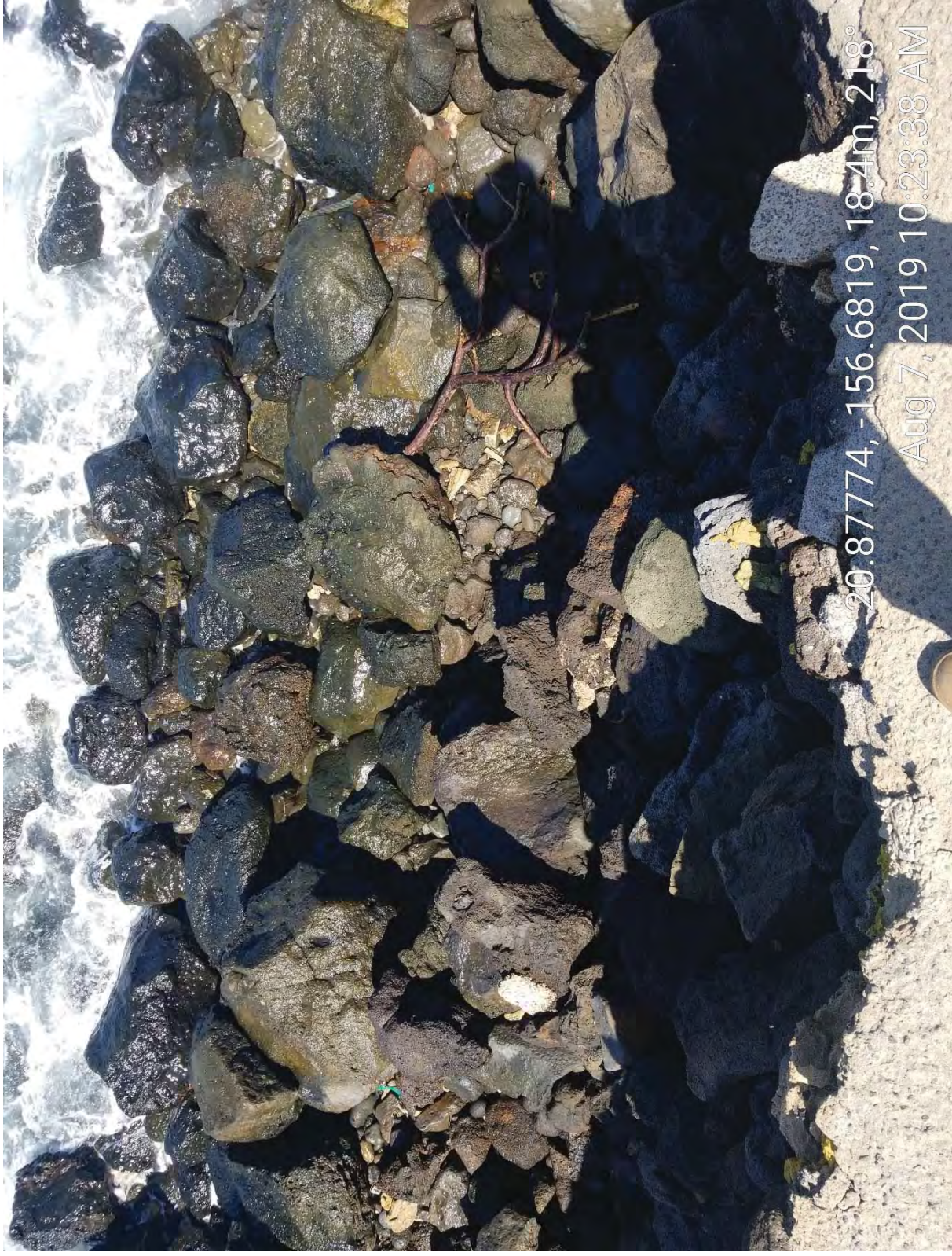
Figure 19: Photographic View of Dry-Laid and Stacked Basalt Rock Seawall to be Repaired in Area 2. View to South.
