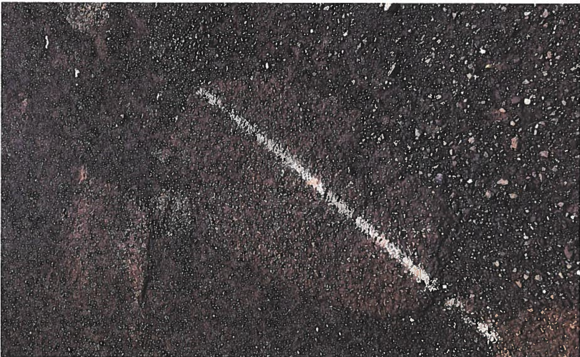
Photo 6. Existing degraded asphalt along Malio Street.
