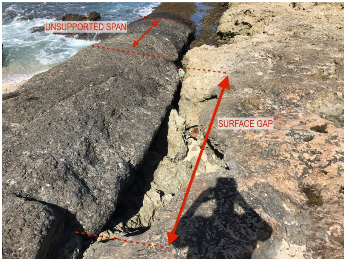
Figure 5-11. Surface gap and voids along north flank of pipeline near waterline/shoreline
