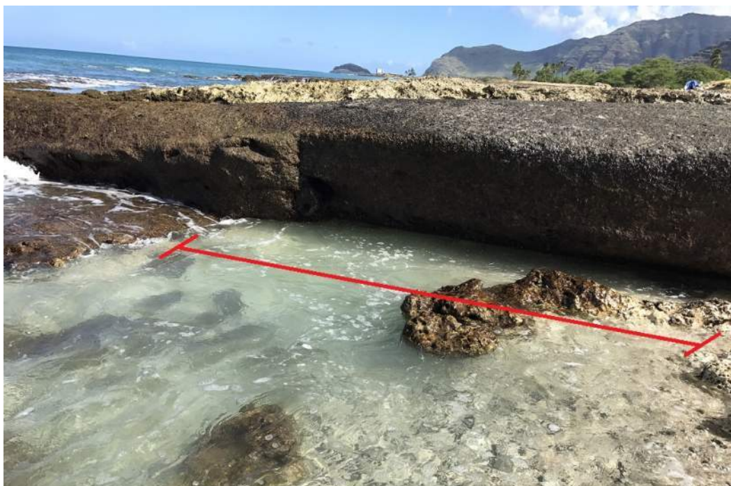
Figure 5-9. Section of unsupported pipe on southern flank of outfall, near the waterline
