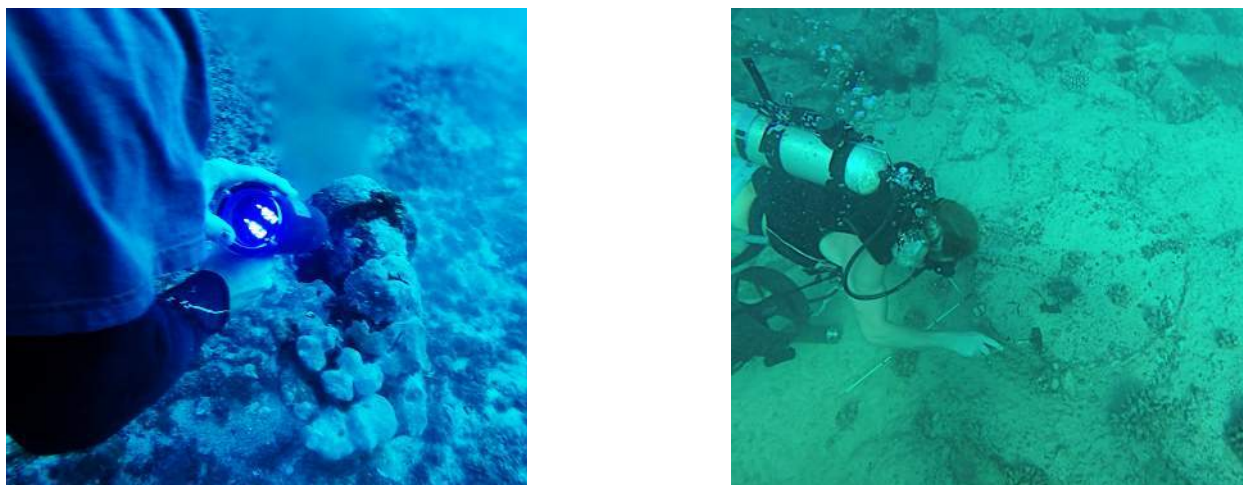
Figure 4-9. CP-gun measurements on monel diffuser bolts ( left ); surface cleaning, cast iron cover, MH3 ( right )
