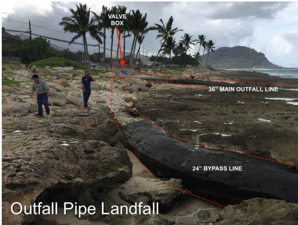
Figure 5-2. Outfall landing, with by-pass line (foreground) and main barrel (background) with MH 1 and valve box
