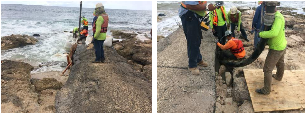
Figure 5-15. Concrete placement within formworks via boom truck ( left ); concrete pumped into gap ( right )
