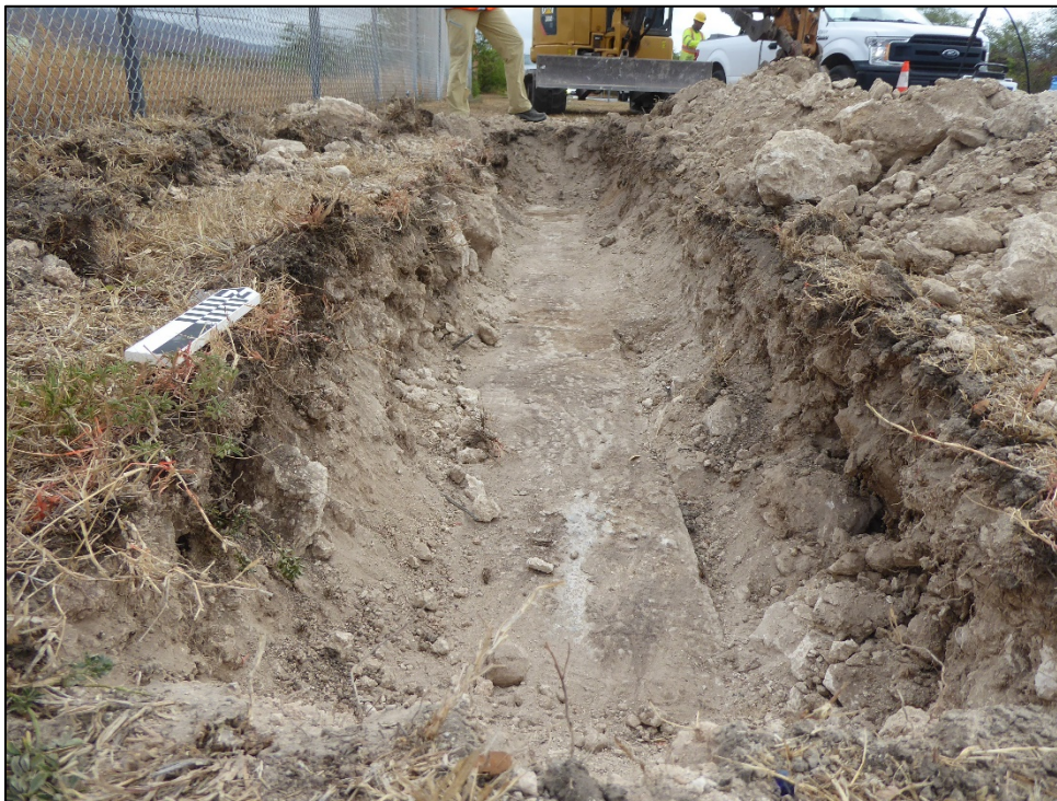
Figure 8. Trench 2, concrete utility jacket oriented north-south within the trench floor (view to north).
