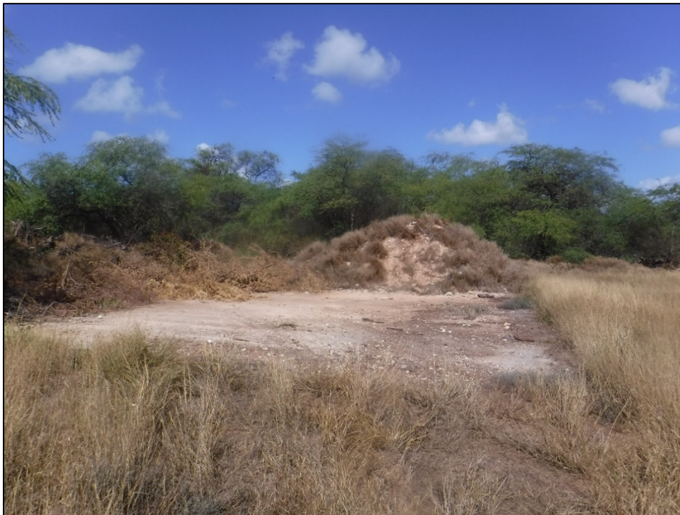
Figure 63. SIHP 50-80-12-XXXXX (T-02), Feature 19 likely Quonset hut concrete foundation (view to southwest).
