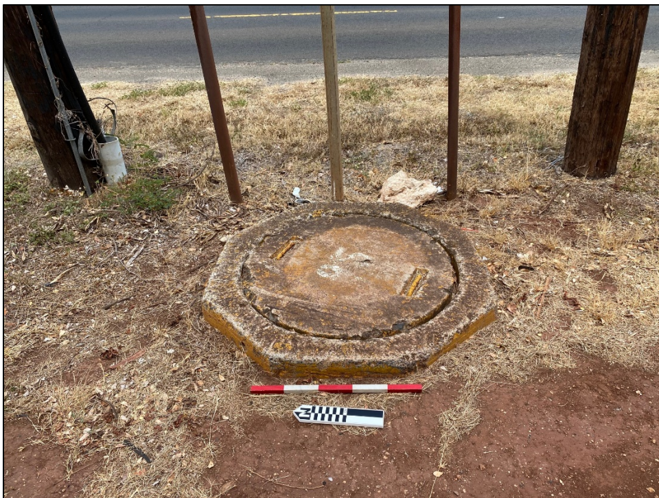
Figure 260. SIHP 50-80-12-XXXXX (T-09) Feature 4 concrete structure with pipes and poles (view to east).
