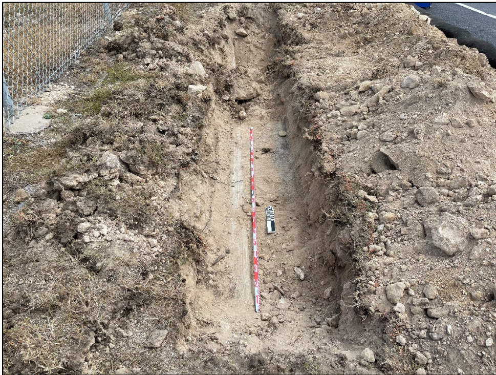
Figure 13. Trench 3, showing a concrete utility jacket oriented northwest-southeast within the trench floor (view to north).
