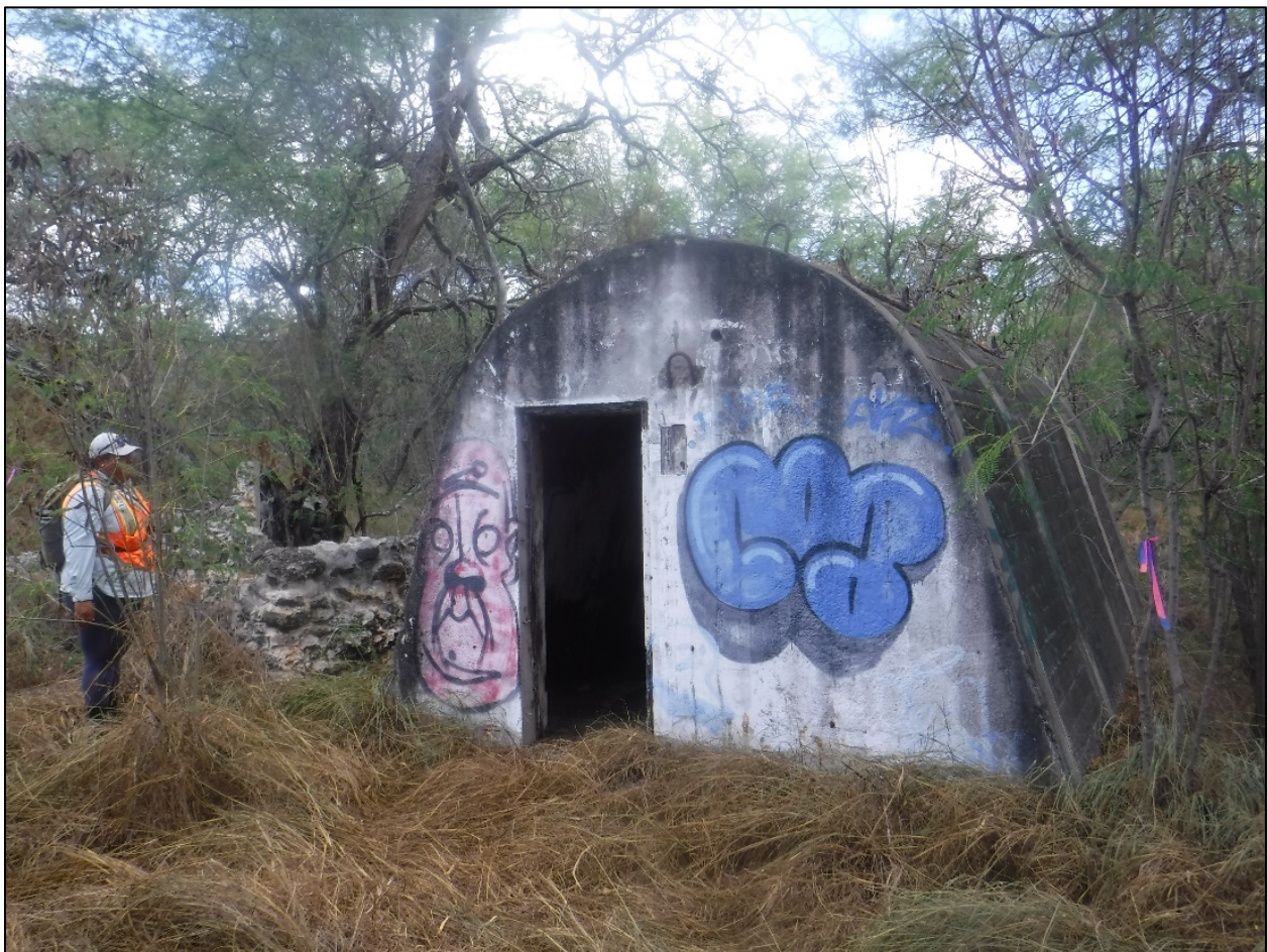
Figure 54. SIHP 50-80-12-XXXXX (T-02), Feature 35 air raid shelter with Feature 36 stone structure on left (view to north).
