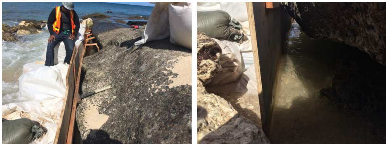
Figure 5-14. Sandbag caisson with plywood forms installation (left); close-up of void area within forms (right)
