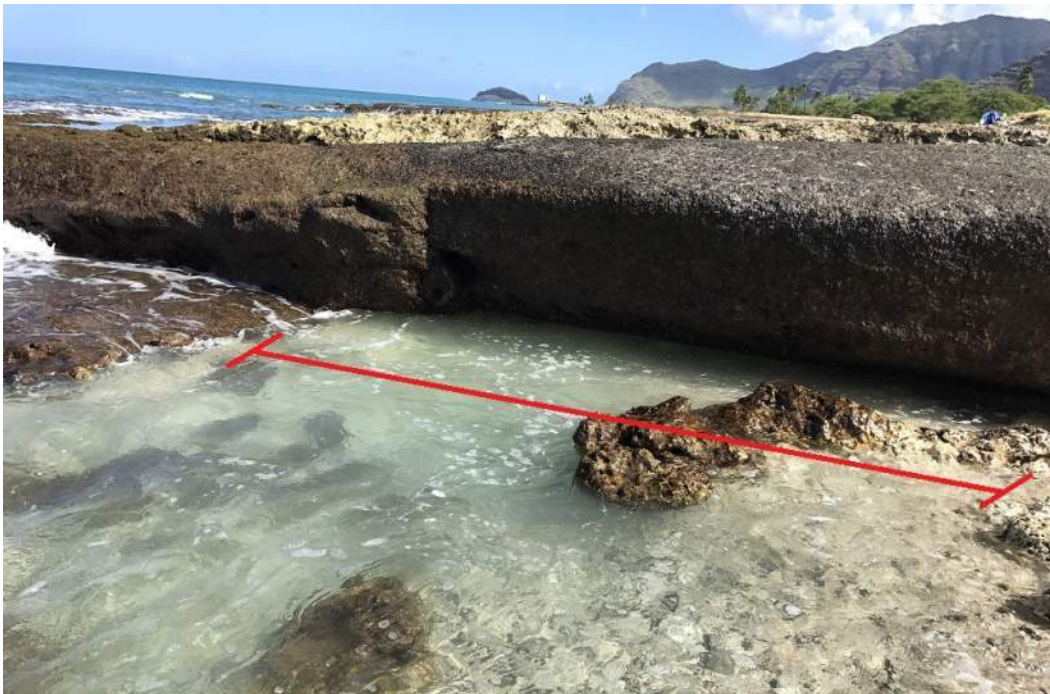
Figure 5-9. Section of unsupported pipe on southern flank of outfall, near the waterline
