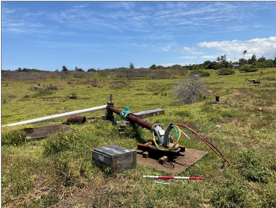
Figure 12. USGS Upolu Observation Well J-B (State Well ID 7451-02), view to the east.
