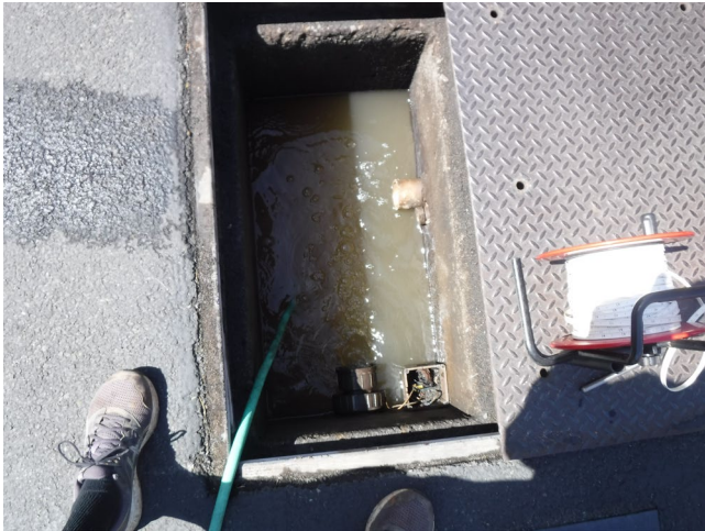
Photo 3: Overhead view of Well 2
