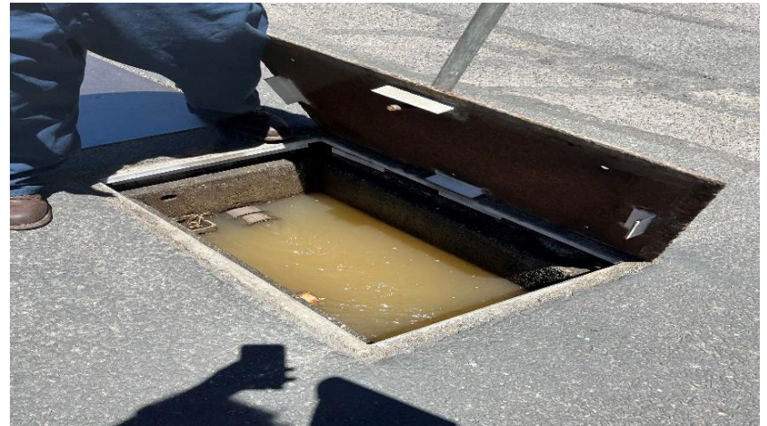
Photo 12: Interior of injection well #2.
