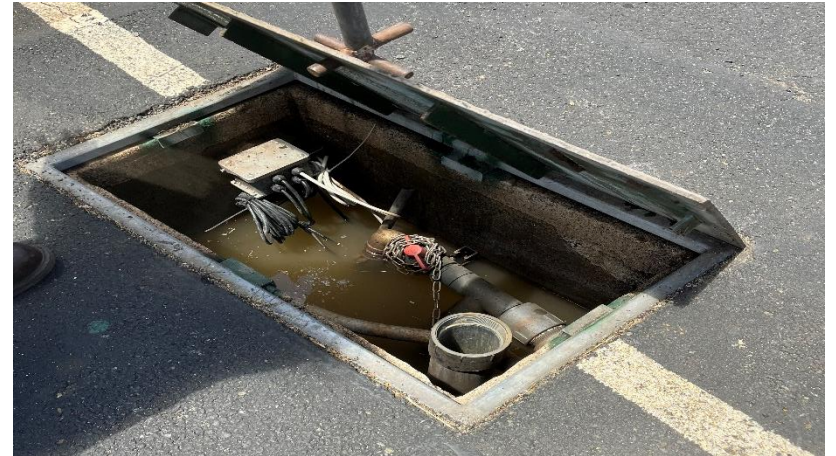
Photo 8: Pump station in parking lot.
