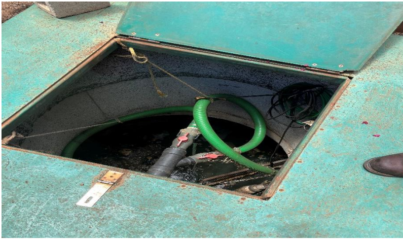
Photo 9: Interior of lift station.
