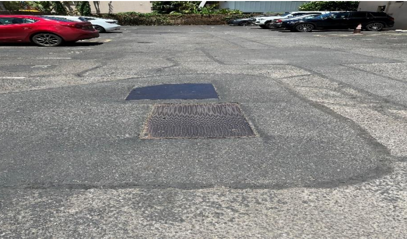
Photo 11: In parking lot, injection well #2 - facing north.
