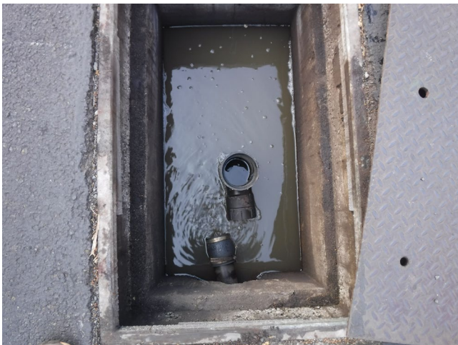
Photo 5: Overhead view of Well 3
