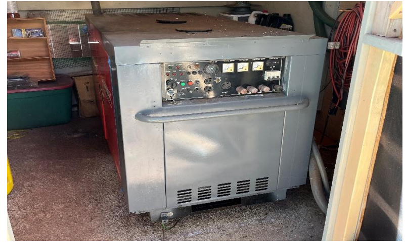
Photo 14: Emergency back-up generator.
