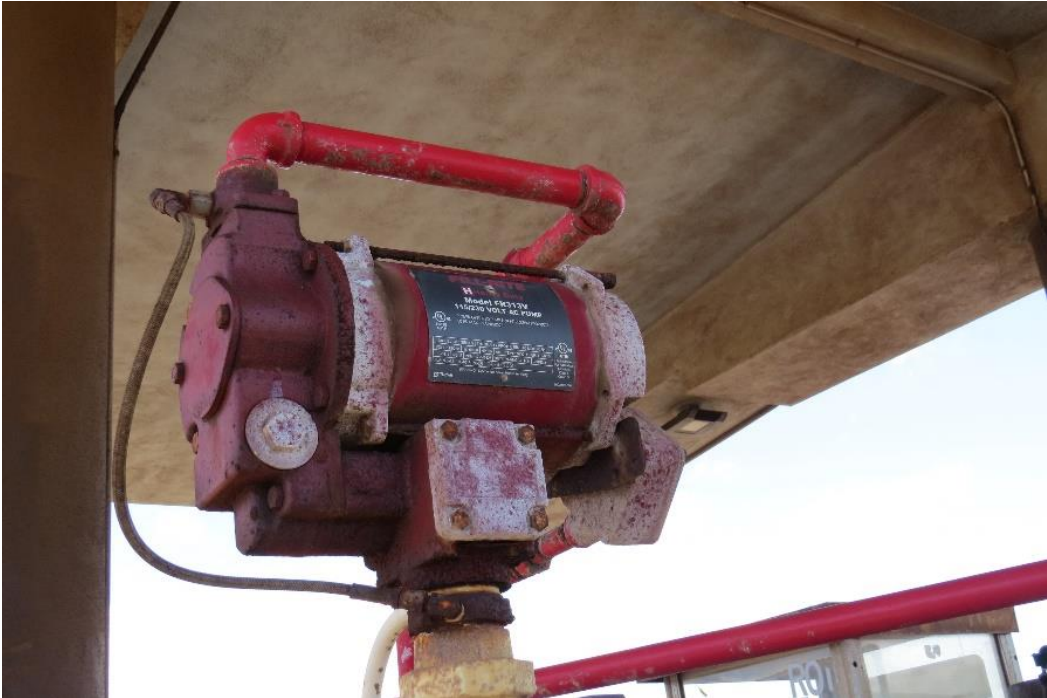
Photo 6: Existing corroded fuel pump.
