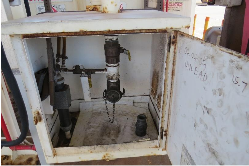
Photo 7: Tank remote fill connection.
