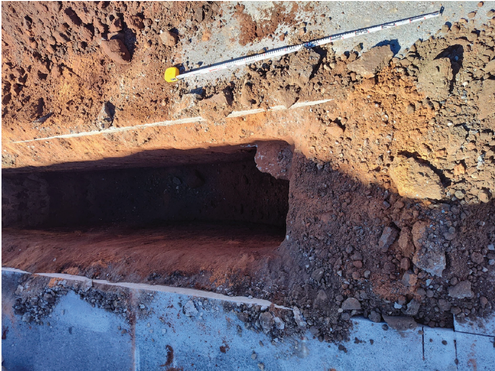
Figure 35: Plan view photograph of ST-8 taken on September 28, 2022 with the concrete kicker visible in the foreground
