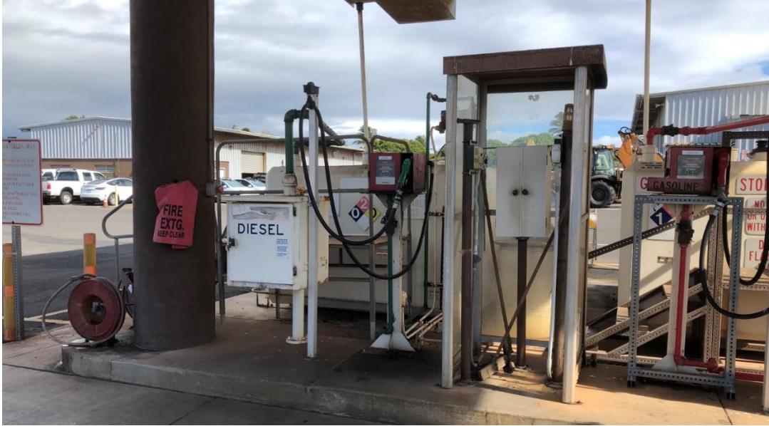
Photo 5: Fueling Station pumps.
