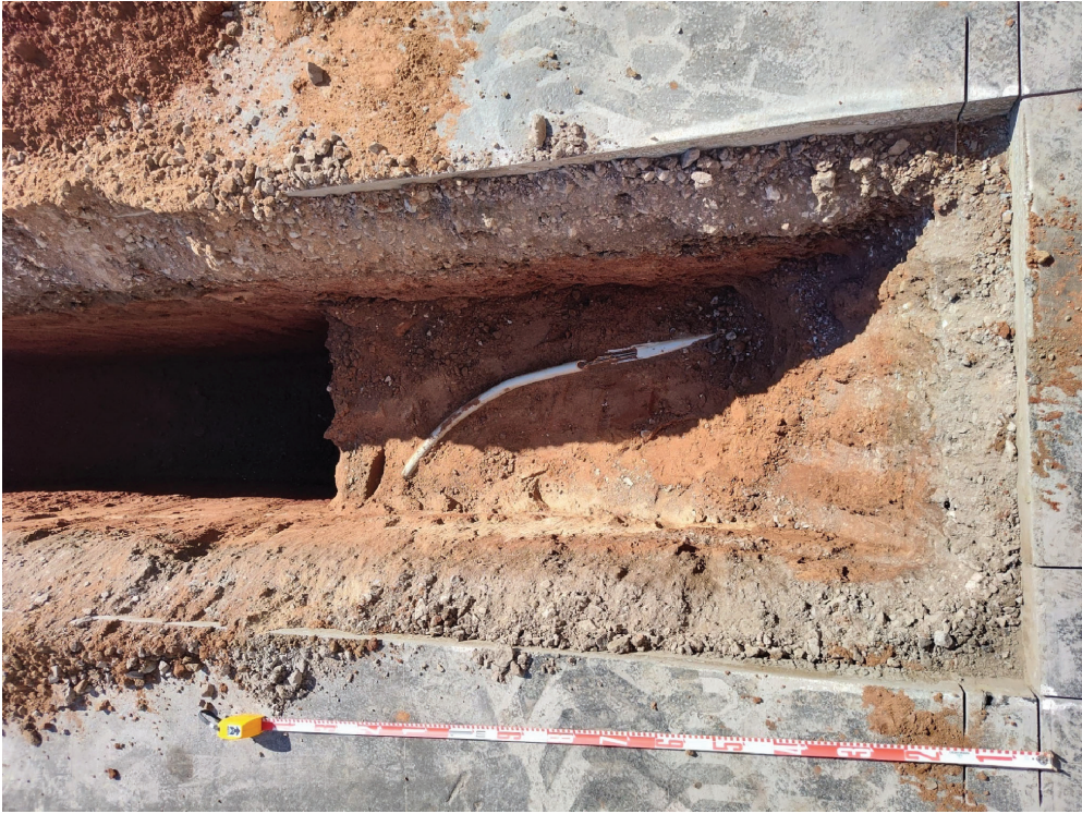
Figure 32: Plan view photograph of ST-7 taken on September 28, 2022 with the electric conduit visible in the foreground
