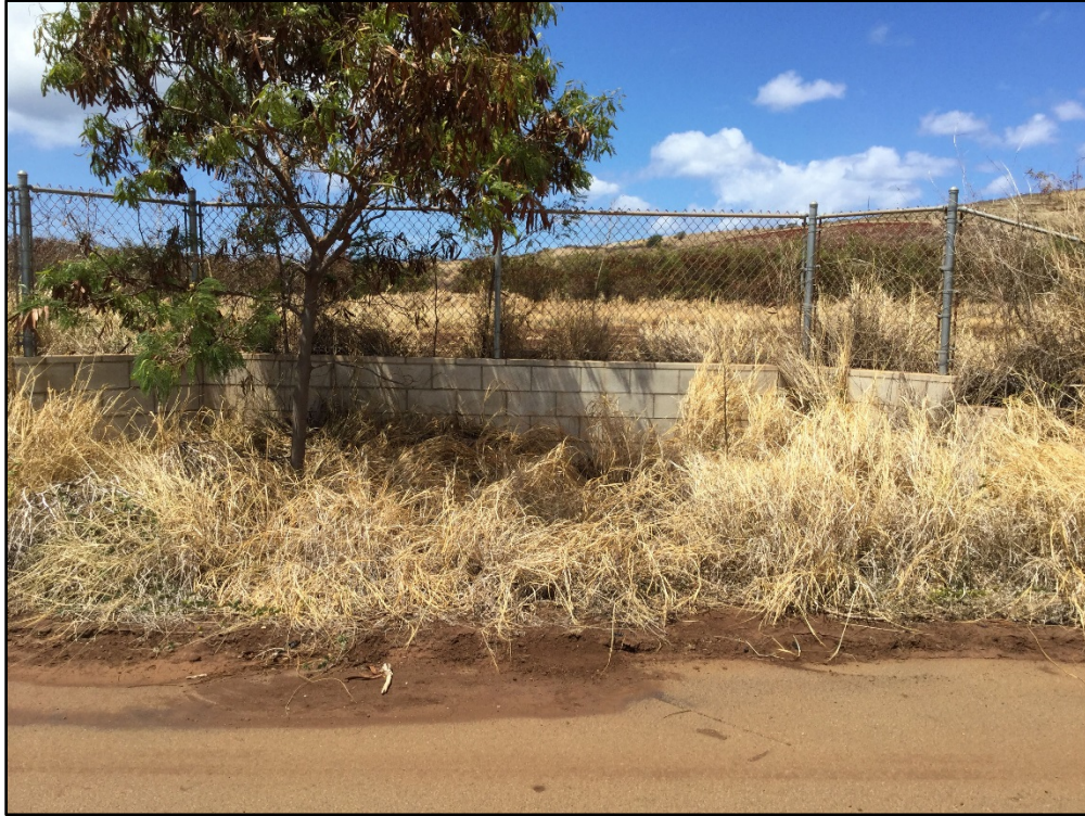
Figure 32. Modern cinder block retaining wall along BWS access road, view to southwest
