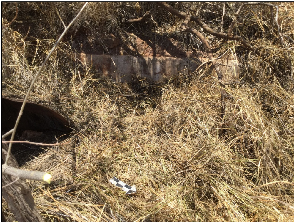
Figure 47. Exposed metal culvert with adjacent retaining wall visible, portions of CSH 1, view to southwest
