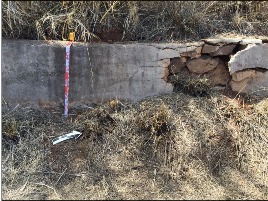
Figure 50. Disturbed section of retaining wall at northeastern end, highlighting construction style of stacked basalt with concrete covering, portion of CSH 1, view to northwest
