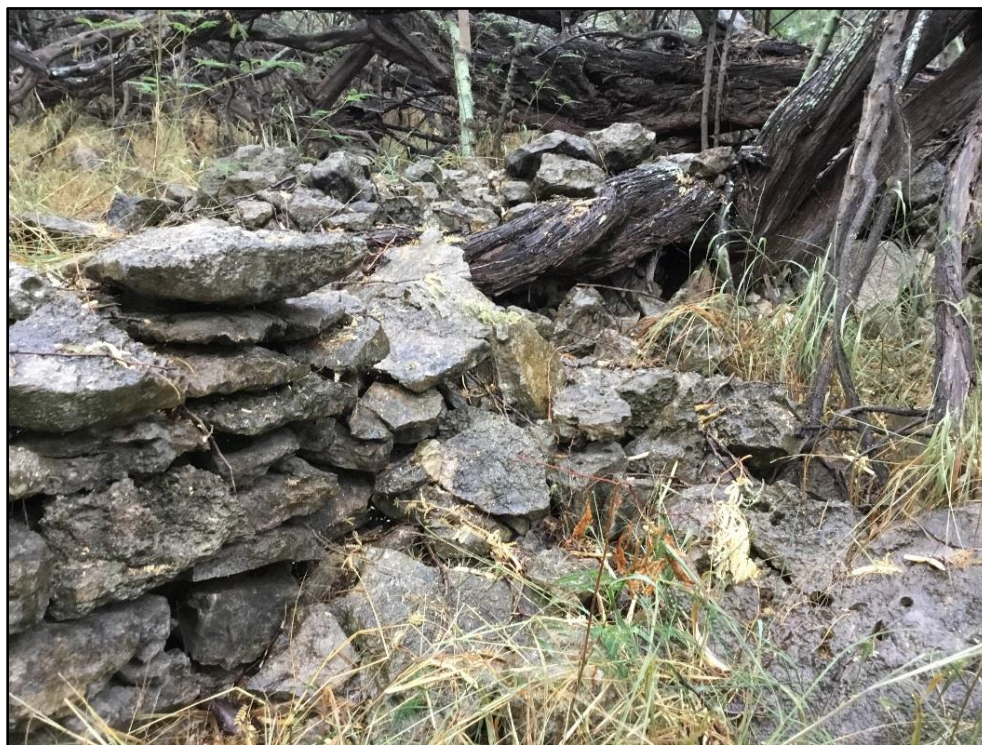
Figure 40. General view of portion of wall damaged by kiawe roots, within the Kalaeloa Heritage Park
