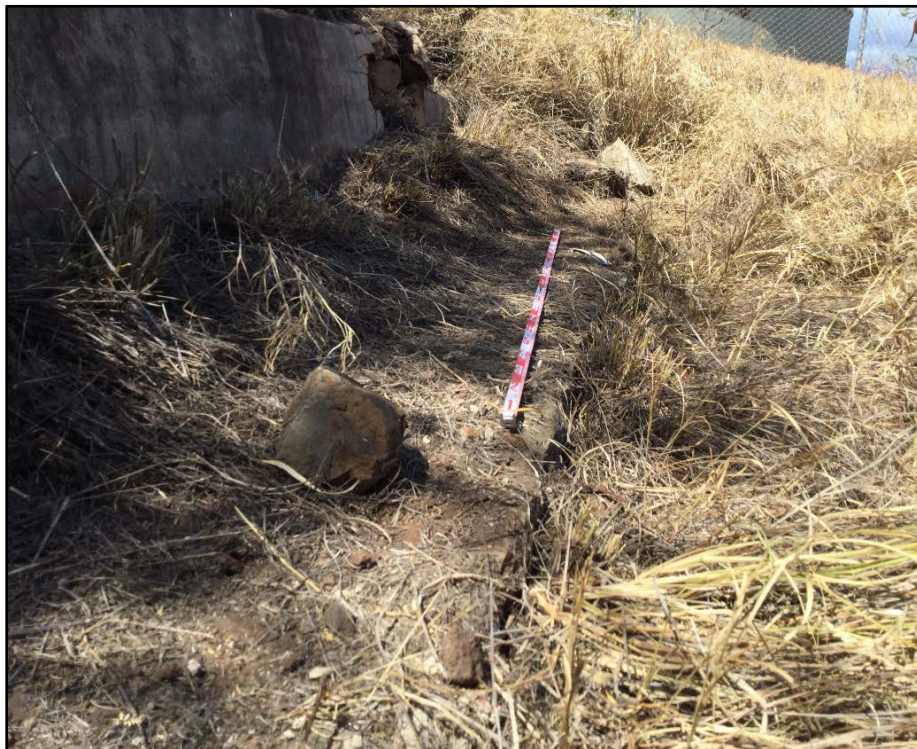
Figure 51. Exposed segment of concrete below retaining wall, portions of CSH 1, view to northeast
