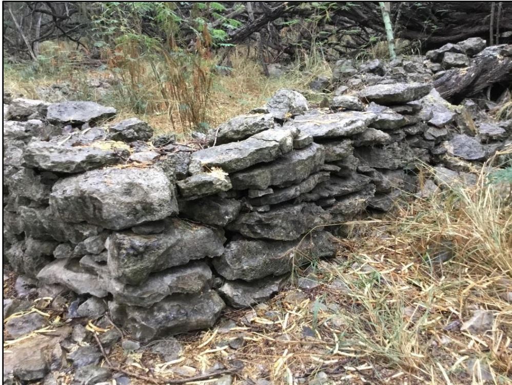
Figure 39. General view of intact portion of wall, within the Kalaeloa Heritage Park
