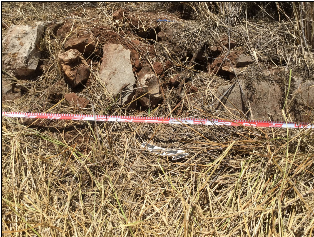
Figure 49. Disturbed middle section of retaining wall, portion of CSH 1, view to west
