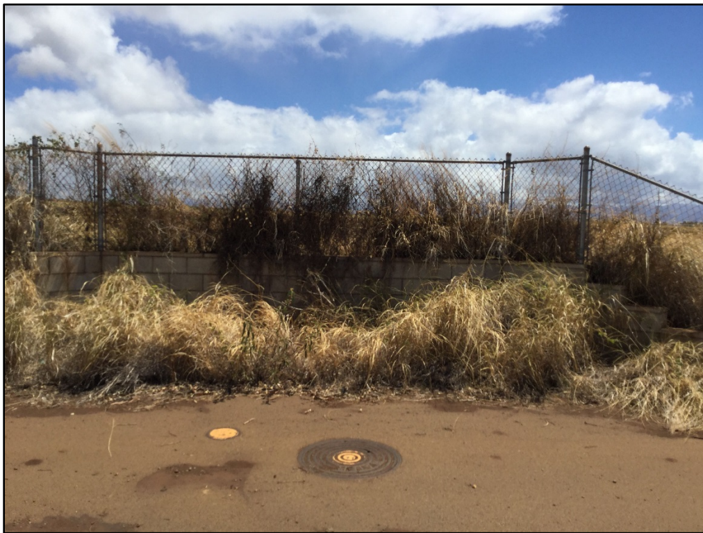
Figure 33. Modern cinder block retaining wall along BWS access road, view to northeast
