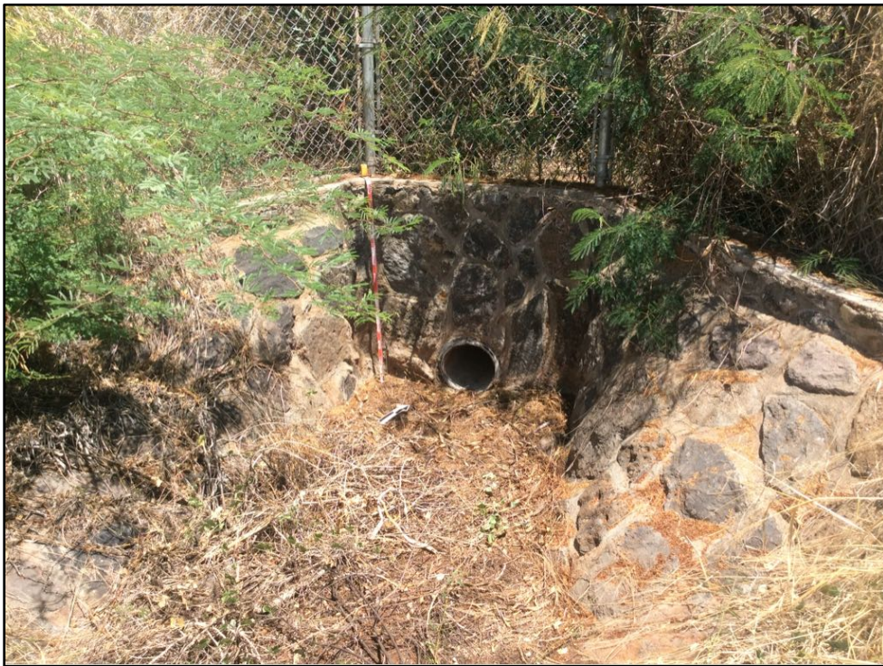
Figure 35. Modern mortared basalt culvert located makai of existing BWS reservoir, view to northwest
