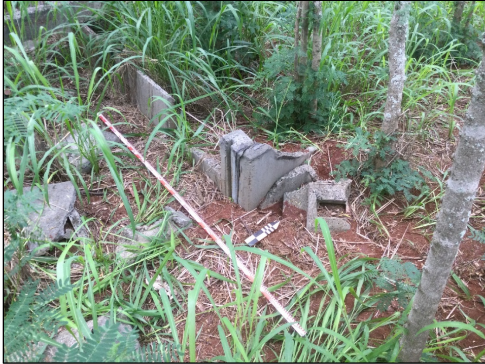
Figure 41. Photo G: PDU alignment 3, east end showing sluice gate, view to northwest
