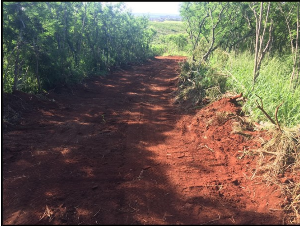
Figure 35. Photo A: Access route down a newly created access for the geotechnical testing drill rig to the proposed reservoir project area, view to south
