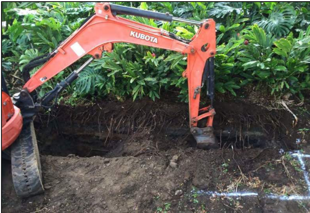
Figure 108. Excavated location of T-8 in relation to planned location (outlined in white), which was backfilled and abandoned shortly after excavation began due to the presence of a water line, view to northeast
