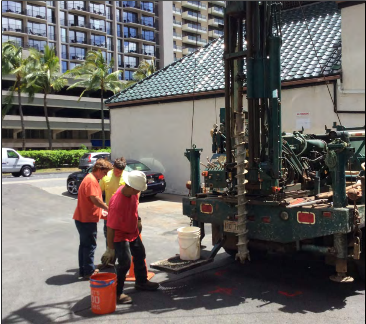
Figure 139. B-2 location, view to north; Kobe Steakhouse building (right) and Ala Moana Boulevard (left) in background
