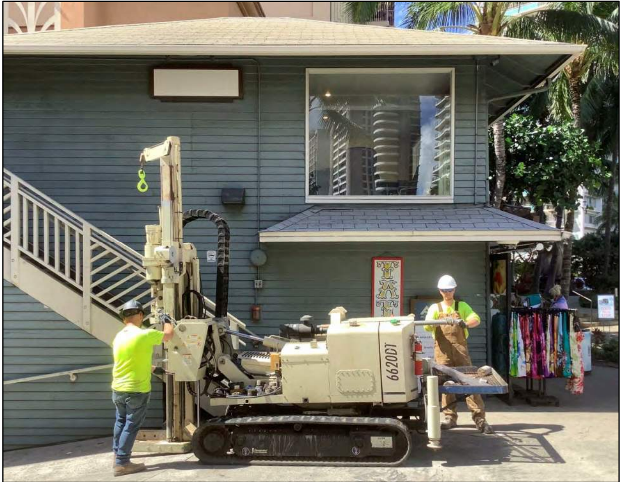
Figure 51. Boring at T-3, view to southwest; ABC store in background, Ala Moana Boulevard on right
