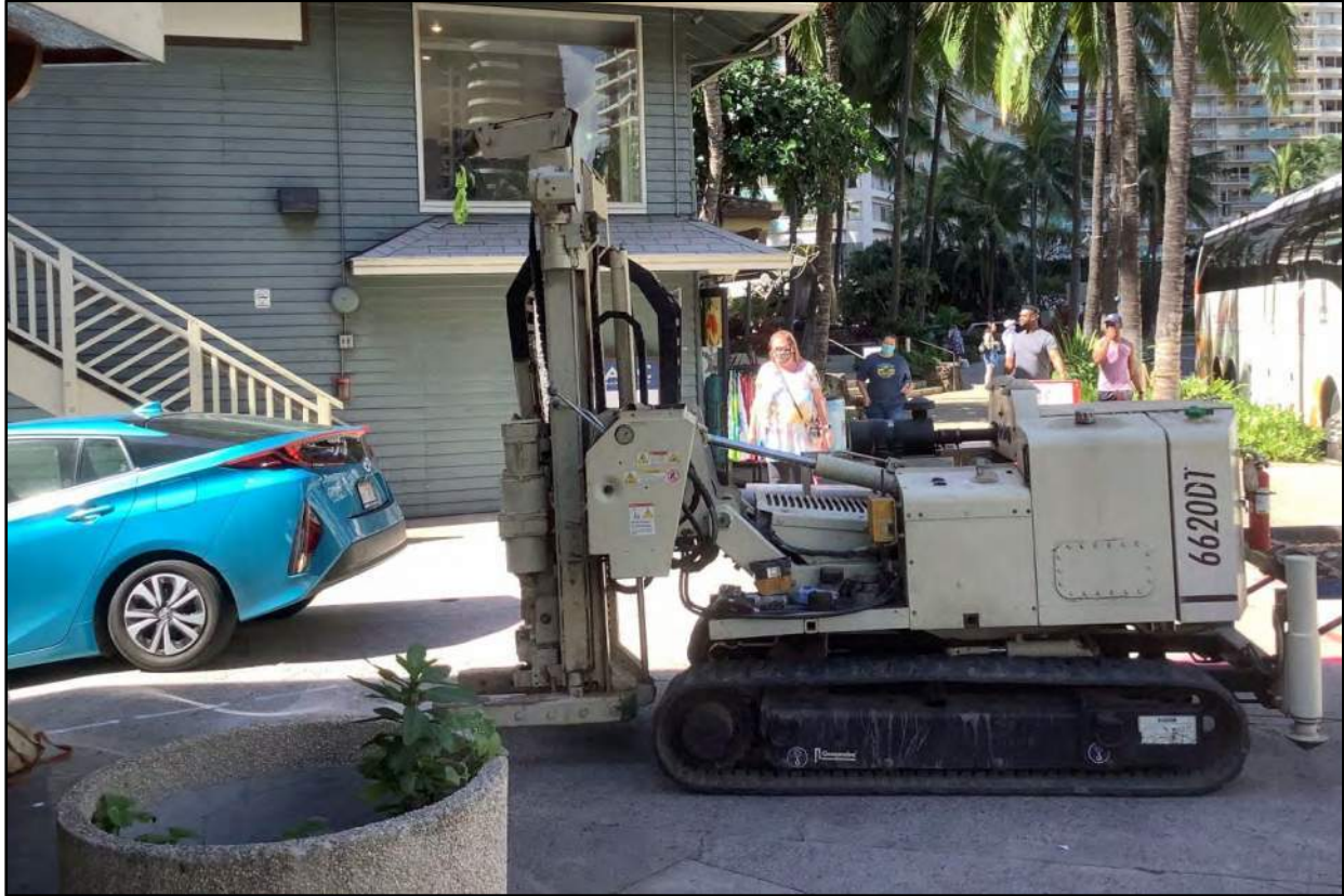
Figure 53. Boring at T-4, view to southwest; ABC store on left, Ala Moana Boulevard on right
