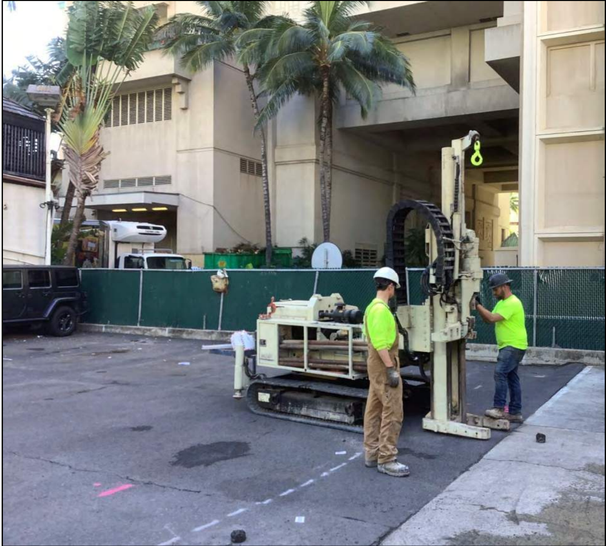
Figure 57. Boring at T-6, view to east; HHV campus in background, Kobe Steakhouse building on left
