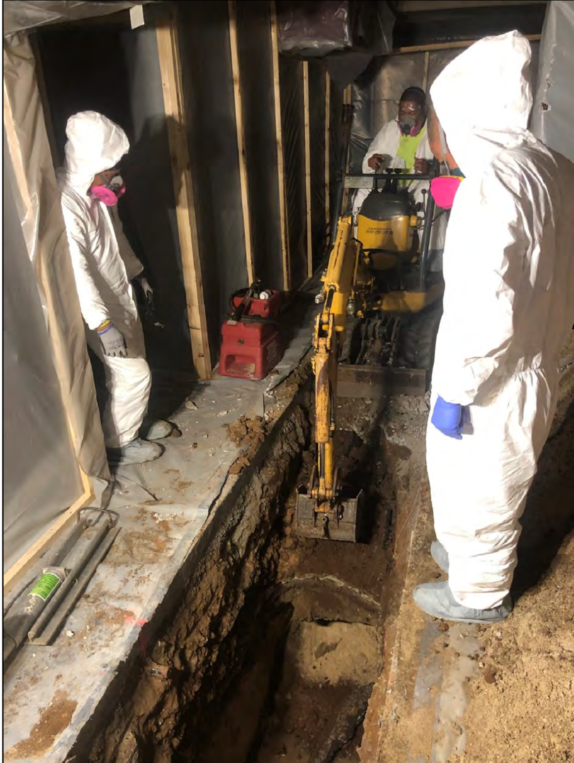
Figure 18. Excavation of T-9 inside the former Kobe Steakhouse building, showing the confined space and use of PPE, view to north; note the plastic sheeting covering the walls and floor for additional protection from mold
