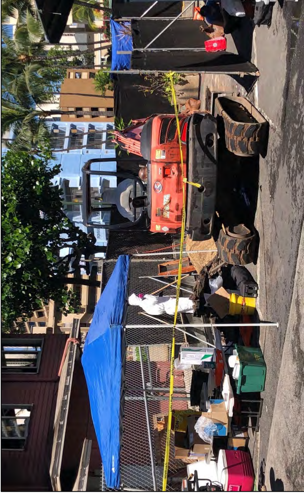
Figure 13. Overview of T-5, excavated in full PPE, view to west; note the “hot zone” where PPE is required to be worn in and around the trench and spoils pile (center), the “warm zone” where PPE was donned and doffed and in-field analysis of samples was conducted (left, under tent), and the “cool zone” where personnel could rest and rehydrate (right); fencing with black mesh provided dust control and privacy from pedestrians and vehicles along Ala Moana Boulevard (in background)
