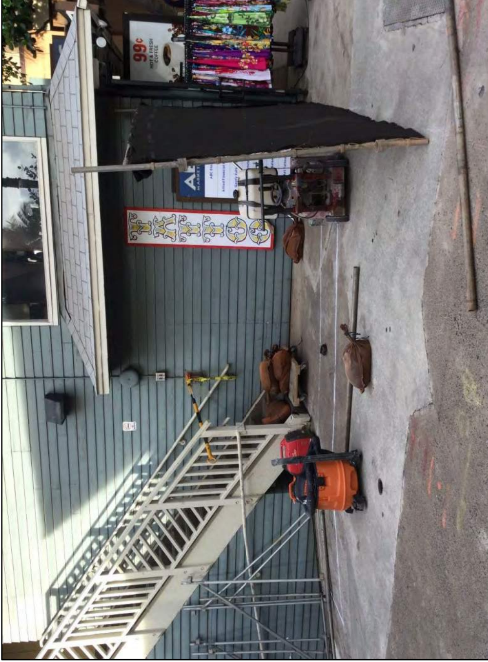
Figure 74. Location of T-3 by the ABC store (in background), with the Ala Moana Boulevard sidewalk on right, view to southwest; note the space limitations created by the existing building, pedestrian accessways, and subsurface utilities (orange and red spray paint)
