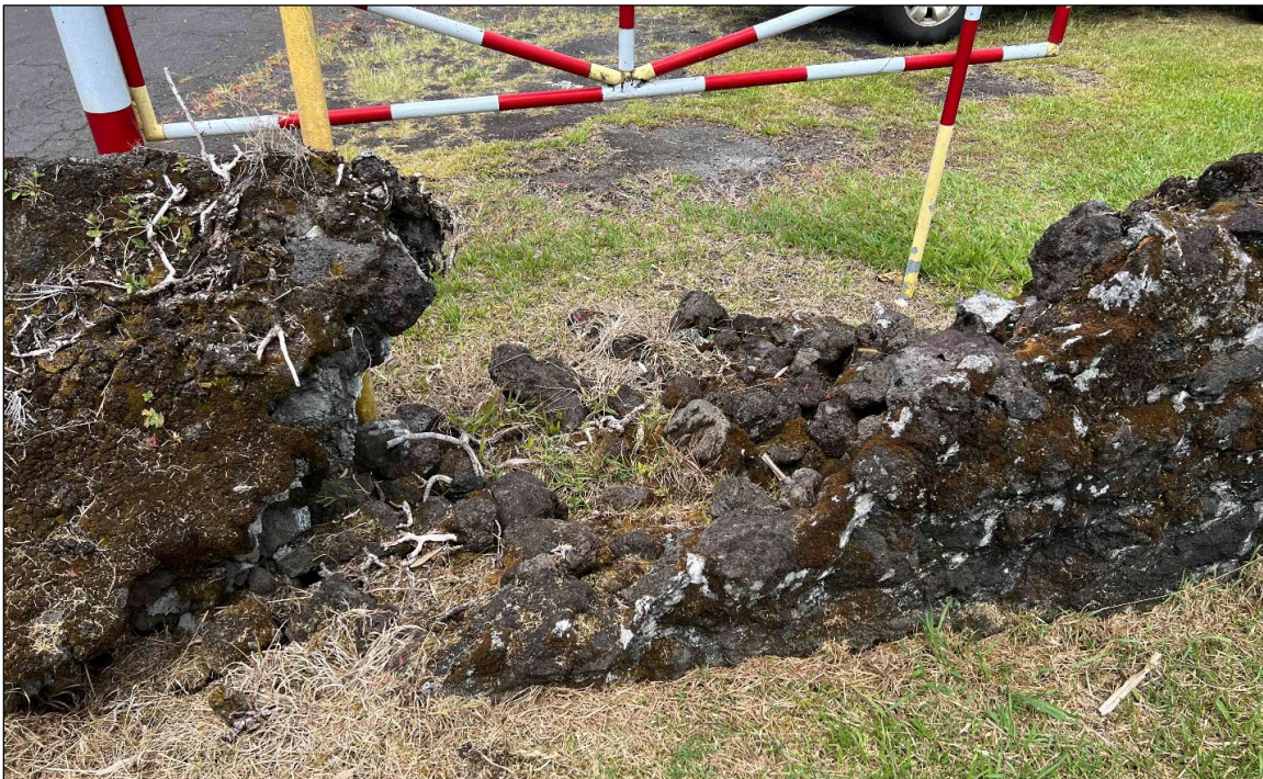
Figure 31. Another view of collapsed section of wall adjacent to entrance driveway (to the south)
