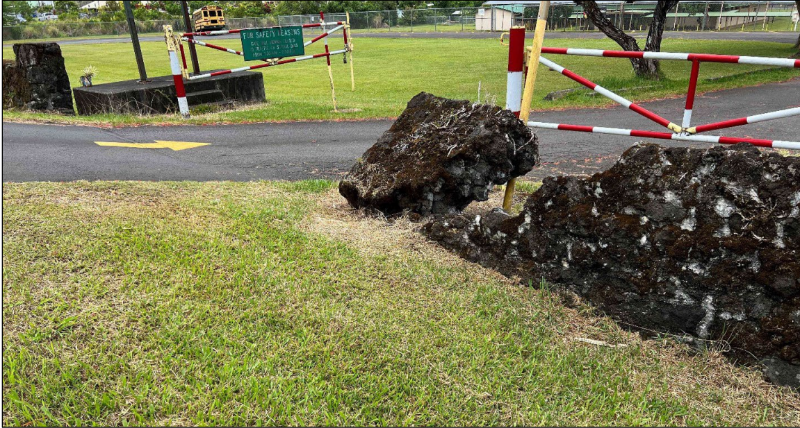
Figure 30. Detail of collapsed section of wall adjacent to the entrance driveway (to the south)
