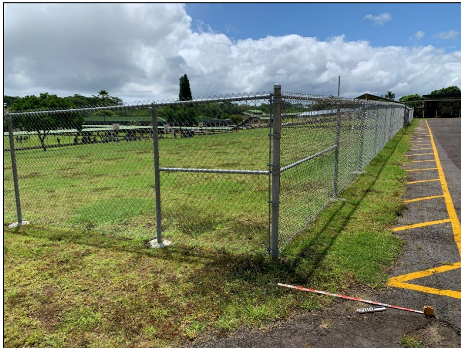
Figure 22. Overview of temporary fencing constructed near the eastern margin of the project area, view to the east
