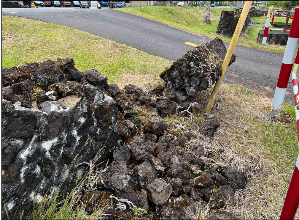
Figure 32. Another view of collapsed section of wall adjacent to entrance driveway (to the south)
