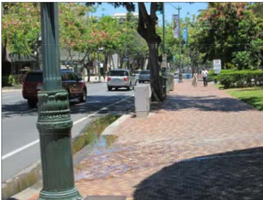
PHOTO 4: PONDING IN GUTTER.
