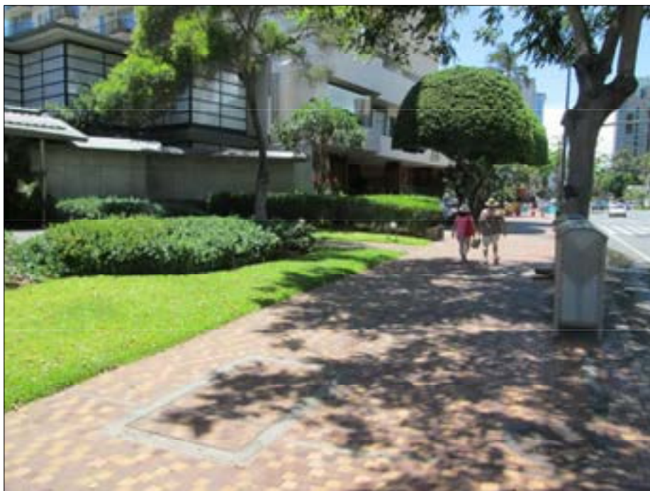
PHOTO 2: DEPRESSED SIDEWALK AREA.
