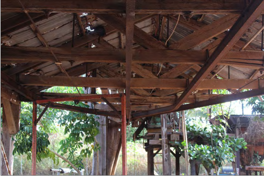
Figure 51. SIHP Site TS-02 4 track overhead I-beam rail system, view to the north.
