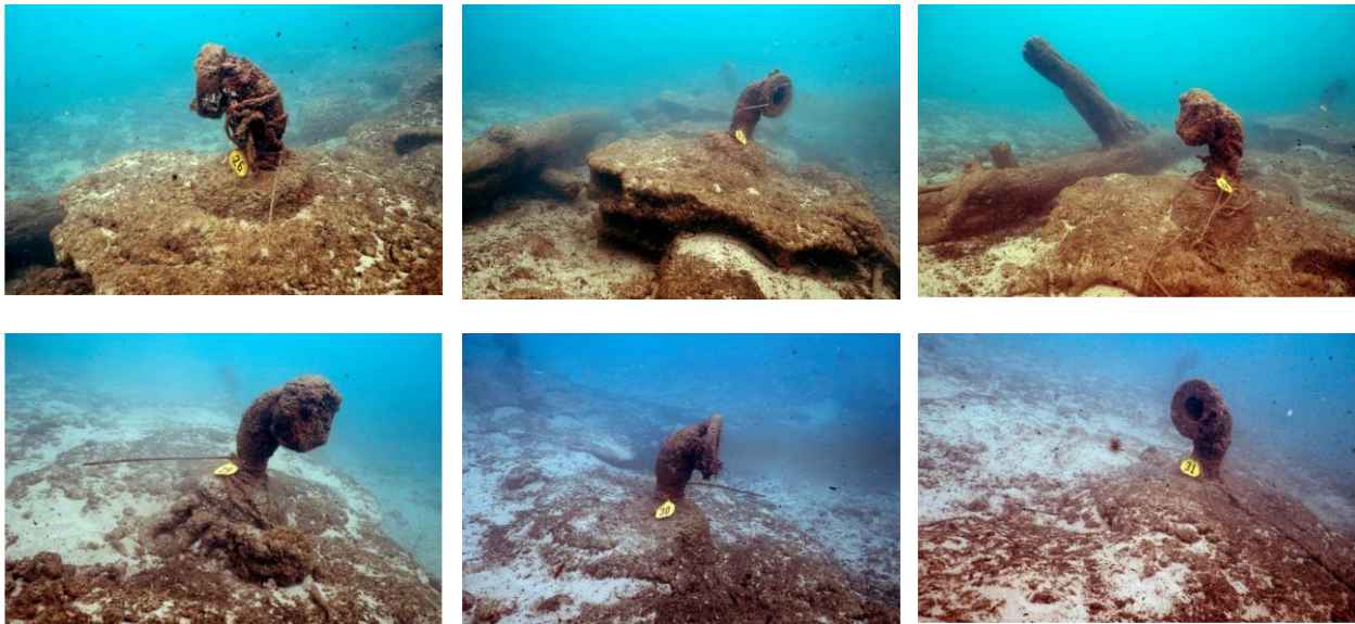
Figure 2-5: Existing Wailua WWTP Ocean Outfall Diffusers
