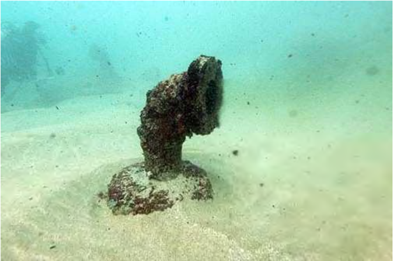
FIGURE 2. Photographs of two Wailua Wastewater Treatment Plant ocean diffuser ports discharging effluent taken on December 23, 2016. Second port can be seen faintly in the background. Note difference in sand cover around ports between Figures 4 (2012) and 3-4 (2016).
