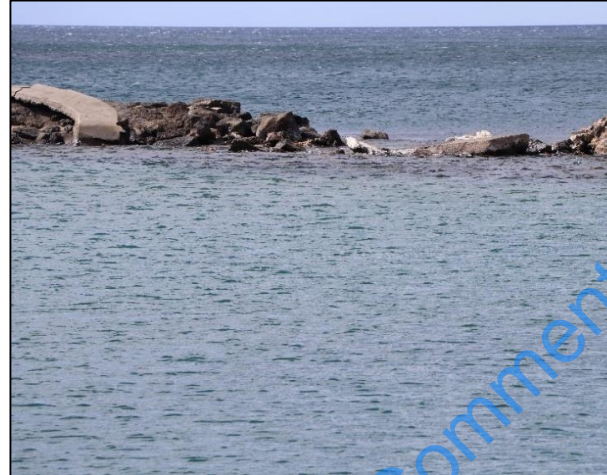
(b) January 2020. Breached section of main breakwater
