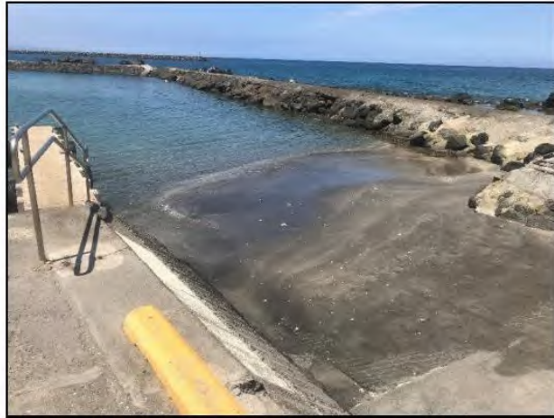
(a) May 2018. Concrete boat ramp with accreted sand.
