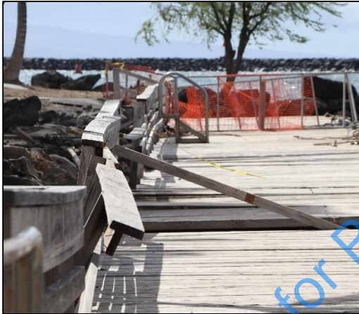
(c) January 2020. Incoming waves hit underside of marginal wooden wharf and damaged structure. Wharf was condemned.
