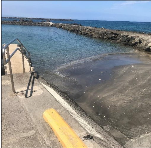
(a) May 2018. Concrete boat ramp with accreted sand.
