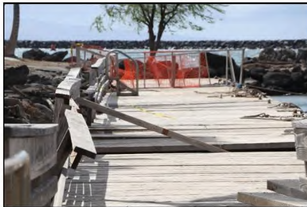
(c) January 2020. Incoming waves hit underside of marginal wooden wharf and damaged structure. Wharf was condemned.
