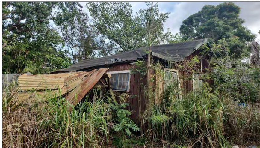
Figure 80. Uninhabitable residence on the south side of Hanapule Street.
