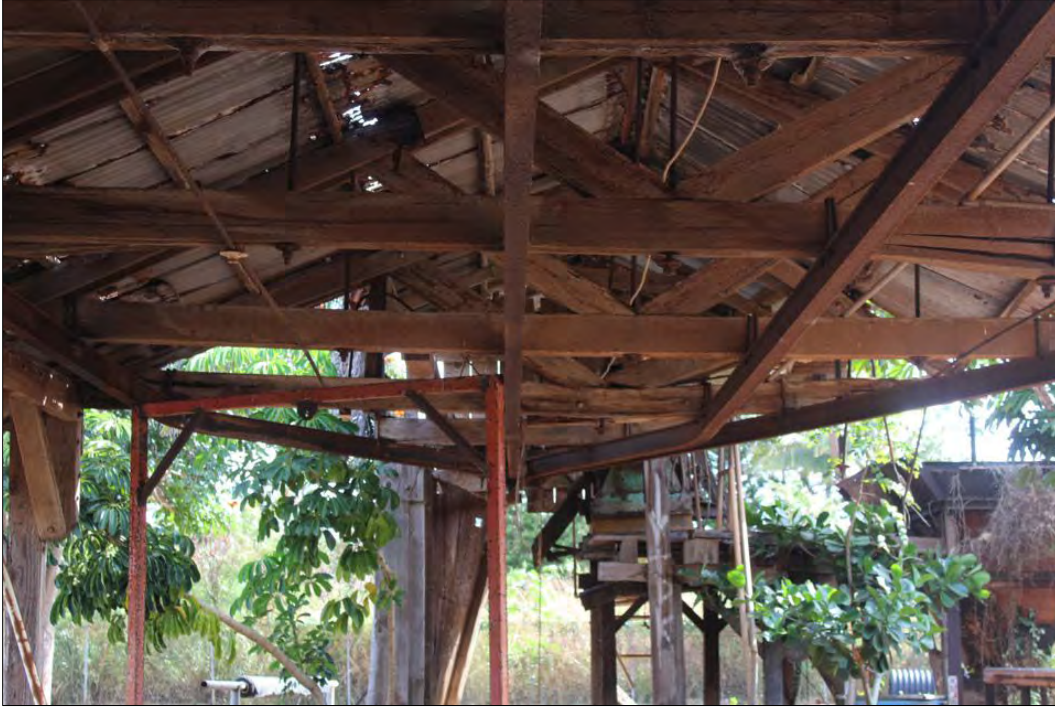
Figure 51. SIHP Site TS-02 4 track overhead I-beam rail system, view to the north.
