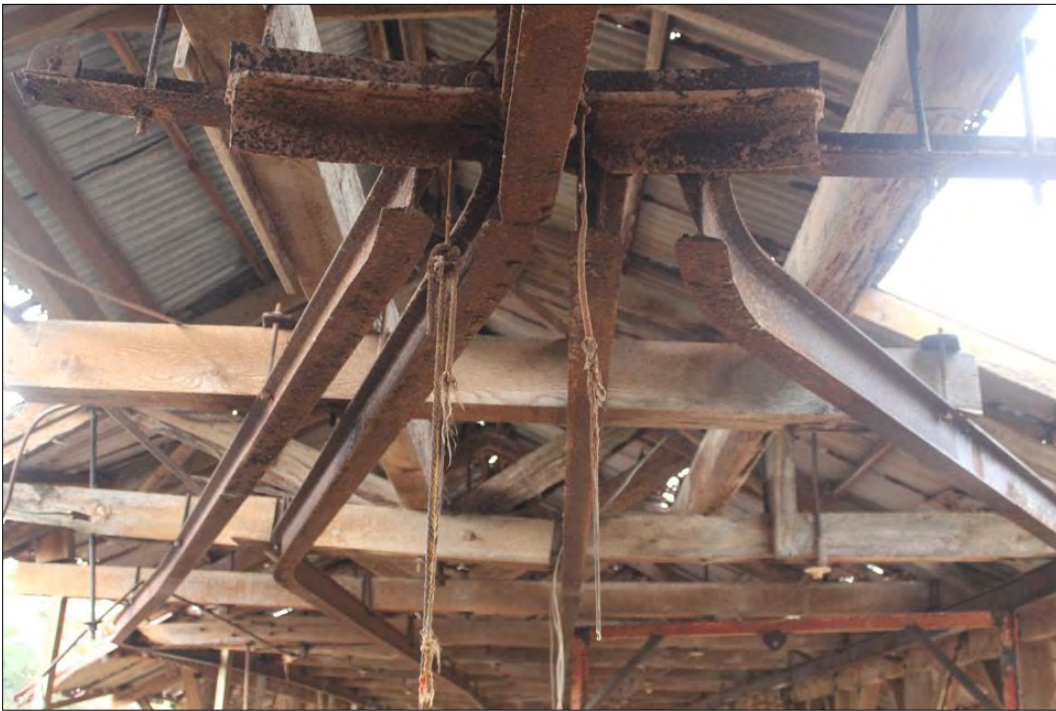
Figure 50. SIHP Site TS-02 switching section of 4 track overhead I-beam rail, view to the south.
