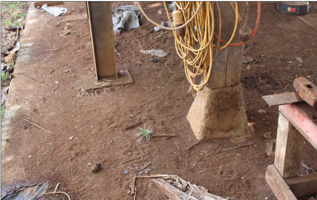
Figure 52. SIHP Site TS-02 original 6 x 8 wooden post on concrete pier block, note metal support post to left of wood post.
