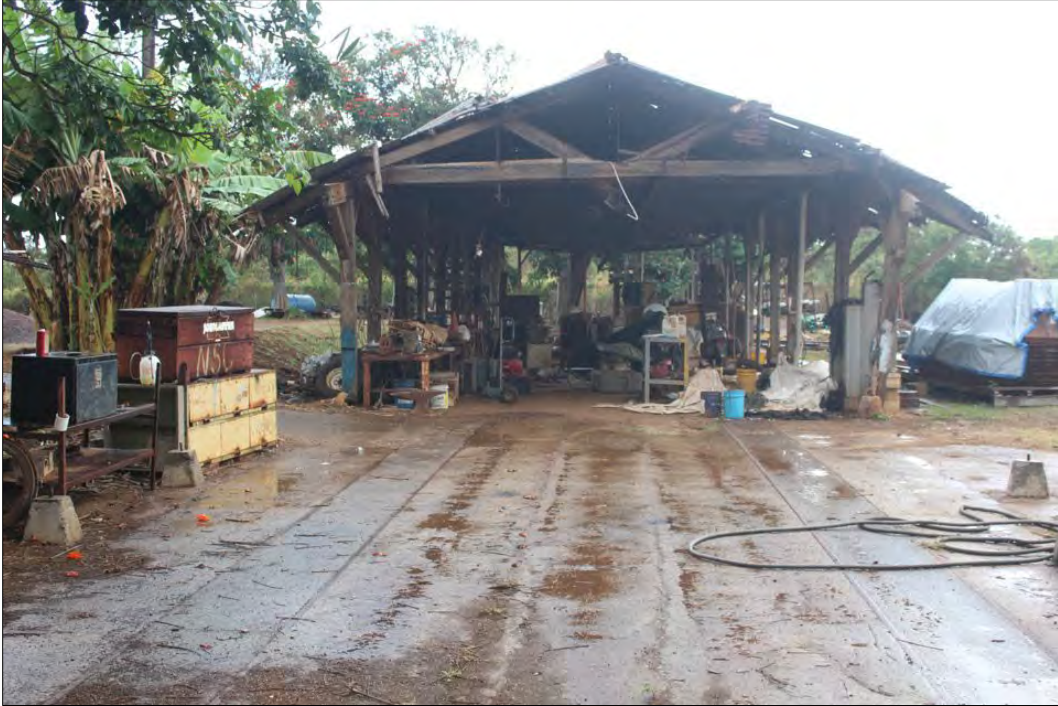
Figure 46. SIHP Site TS-02 missing portion (foreground) of main structure, view to the north.
