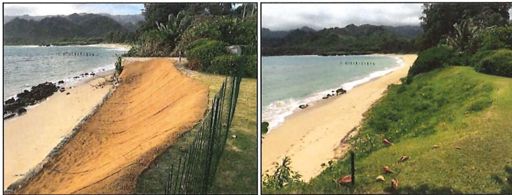
Figure 5-4 Slope stabilization with native vegetation planting on biodegradable coir providing soft shoreline protection (Lā'ie, O'ahu)
