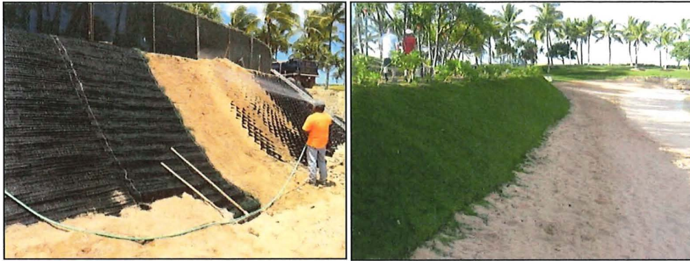
Figure 5-3 Slope stabilization with GEOCELLS and vegetation providing soft shoreline protection (Ko'olina, O'ahu)
