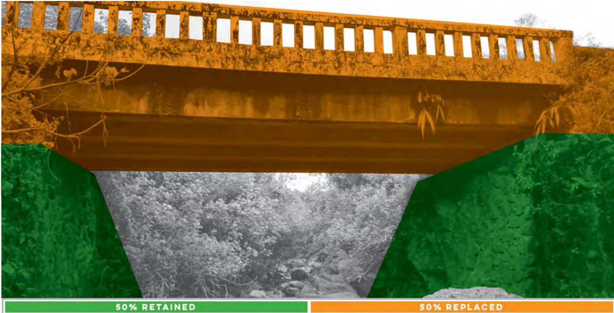
Figure 1: Kailua Stream Bridge, Overview of Effects and Rendering of the Proposed Action
