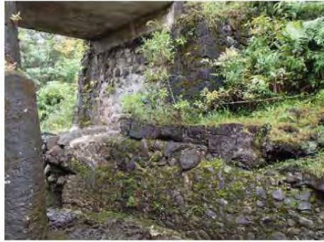
CRM abutment set on natural rock and CRM wingwall, Hana side Courtesy of NOEI
