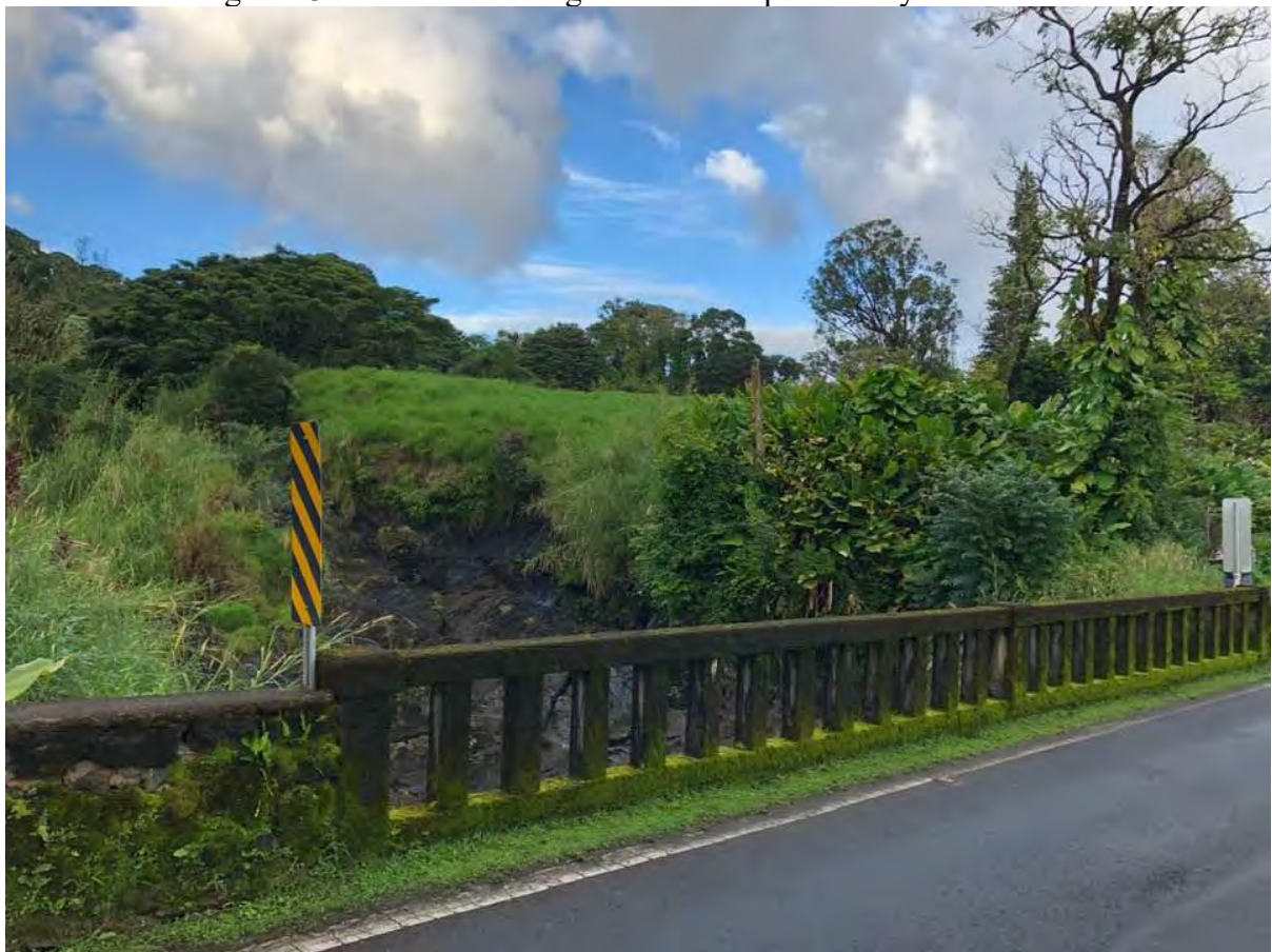
Figure 24. Mokulehua Bridge with view of upstream vegetation.
