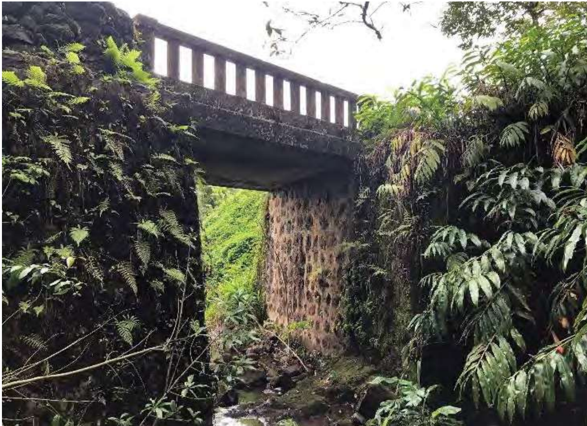
Photo 3-2. Bridge #5—Makanali Stream Bridge crossing the Makanali Stream (looking downstream from the mauka side of the bridge)
