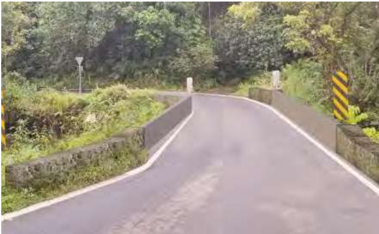
Proposed Typical Section for Bridge #40 – Mokulehua Stream Bridge. Note: Concrete Slab Bridge layout is similar to the existing concrete slab bridge section.
