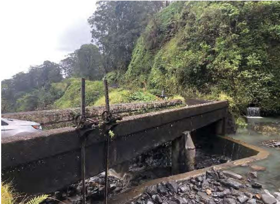
Photo 3-4. Bridge #19—Kopiliula Stream Bridge crossing the Kopiliula Stream (looking downstream from the mauka side of the bridge—Note East Maui Irrigation Co. sluice gate and weir)
