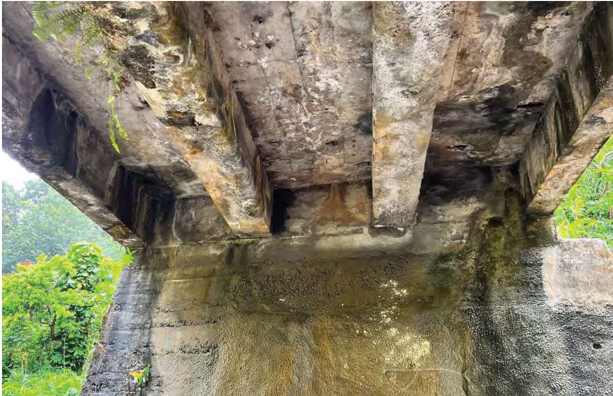
Photo 1-1. General Degradation and Condition of Structures (Bridge #8—Puohokamoa Stream Bridge)
