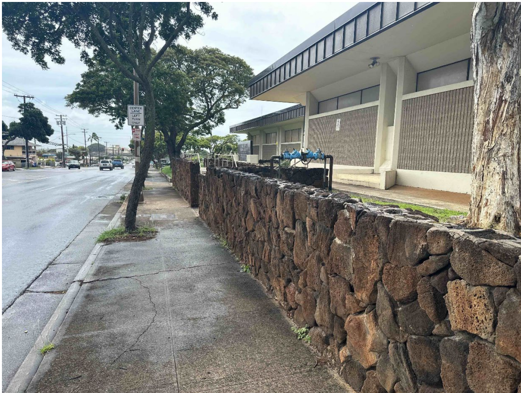
Figure 17. Eastern side of Pearl City Public Library along Waimano Home Road, view to the south.
