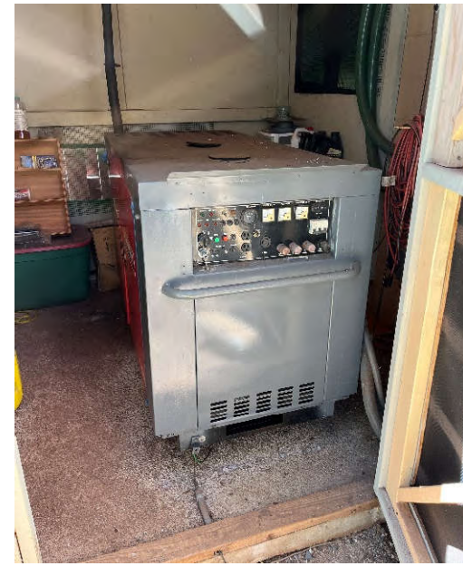
Photo 14: Emergency back-up generator inside machine room attached to Pool House.
