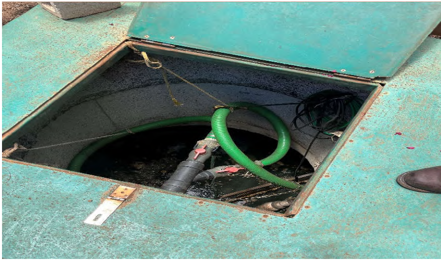
Photo 9: Interior of lift station.
