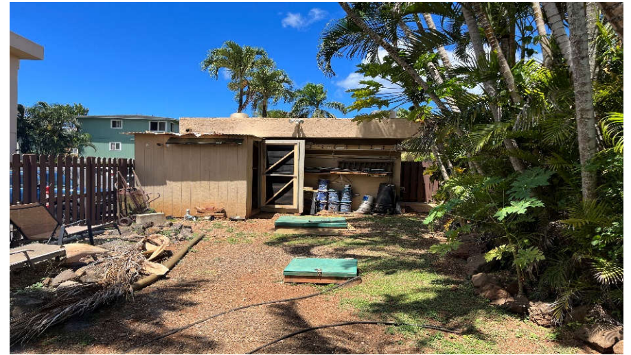
Photo 6: North portion of wastewater treatment system enclosure - facing north. Generator enclosure/machine room and Pool House in background.
