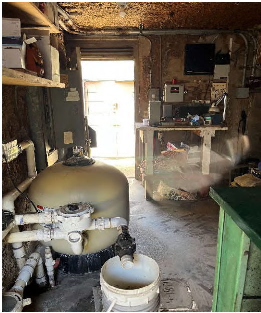
Photo 13: Interior of blower room inside Pool House.
