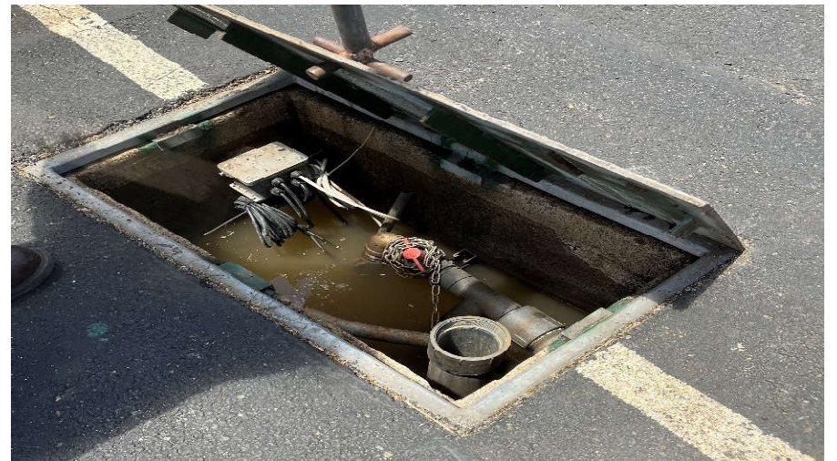
Photo 8: Pump station in parking lot.
