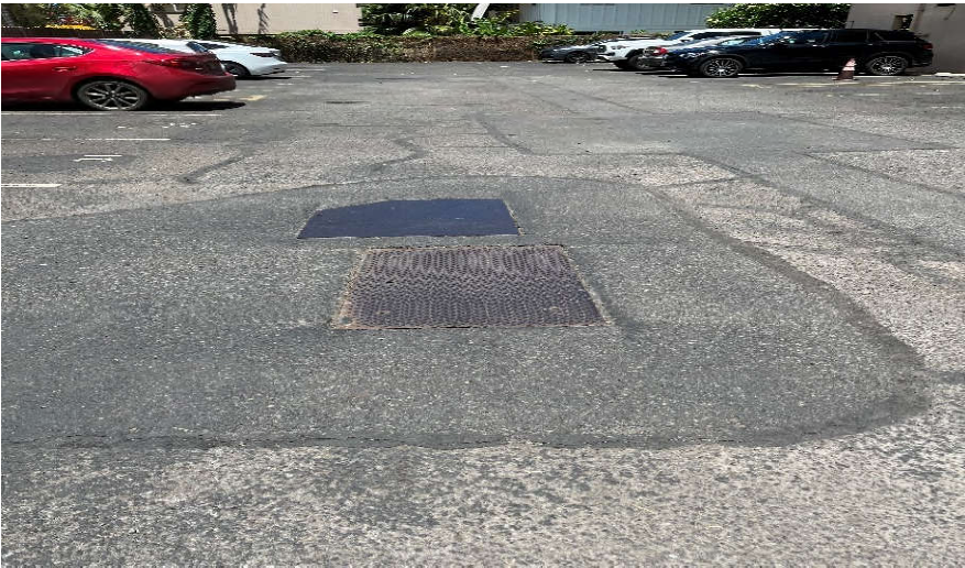
Photo 11: In parking lot, injection well #2 - facing north.
