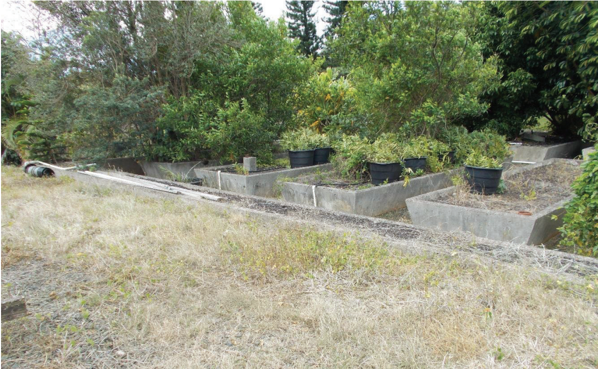
Figure 12. Concrete planters showing the perimeter planter at the southeast side. View facing northwest.
