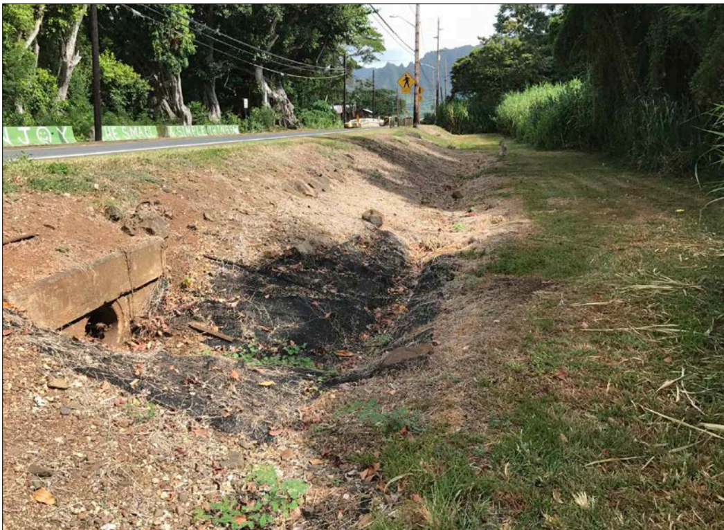
Figure 33. Recent photograph of Feature C of SIHP Site 50-80-10-5768 where it crosses beneath Kamehameha Highway.
