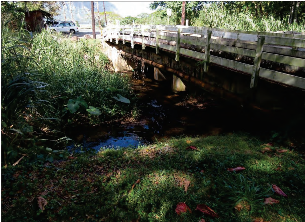
Figure 28. Mauka side of Waiāhole Bridge showing multi-column substructure and pedestrian walkway; note debris trapped beneath deck in foreground, view to the northeast,
