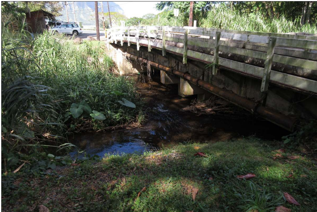
Figure 24. Mauka side of Waiāhole Bridge showing multi-column substructure and pedestrian walkway; note debris trapped beneath deck in foreground (view to the northeast)
