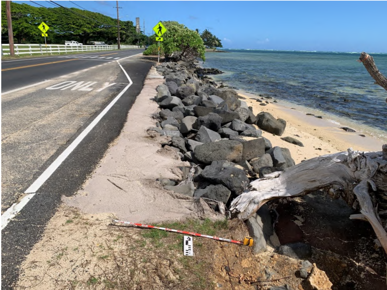
Figure 40. Retaining structures near the southern end of section 8 (Kualoa 2 Ahupua‘a); view north
