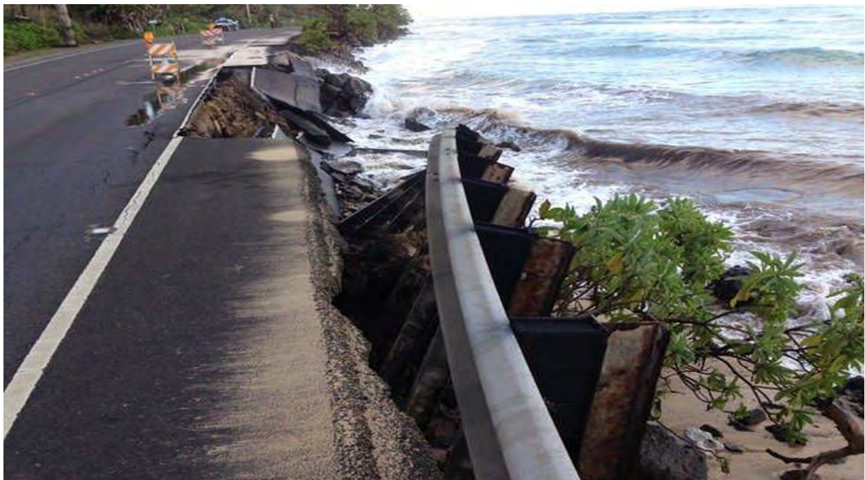
Figure 1-9. Pavement collapse along Kamehameha Hwy in Kaaawa, 2017. Note brown erosion plume, at right.
