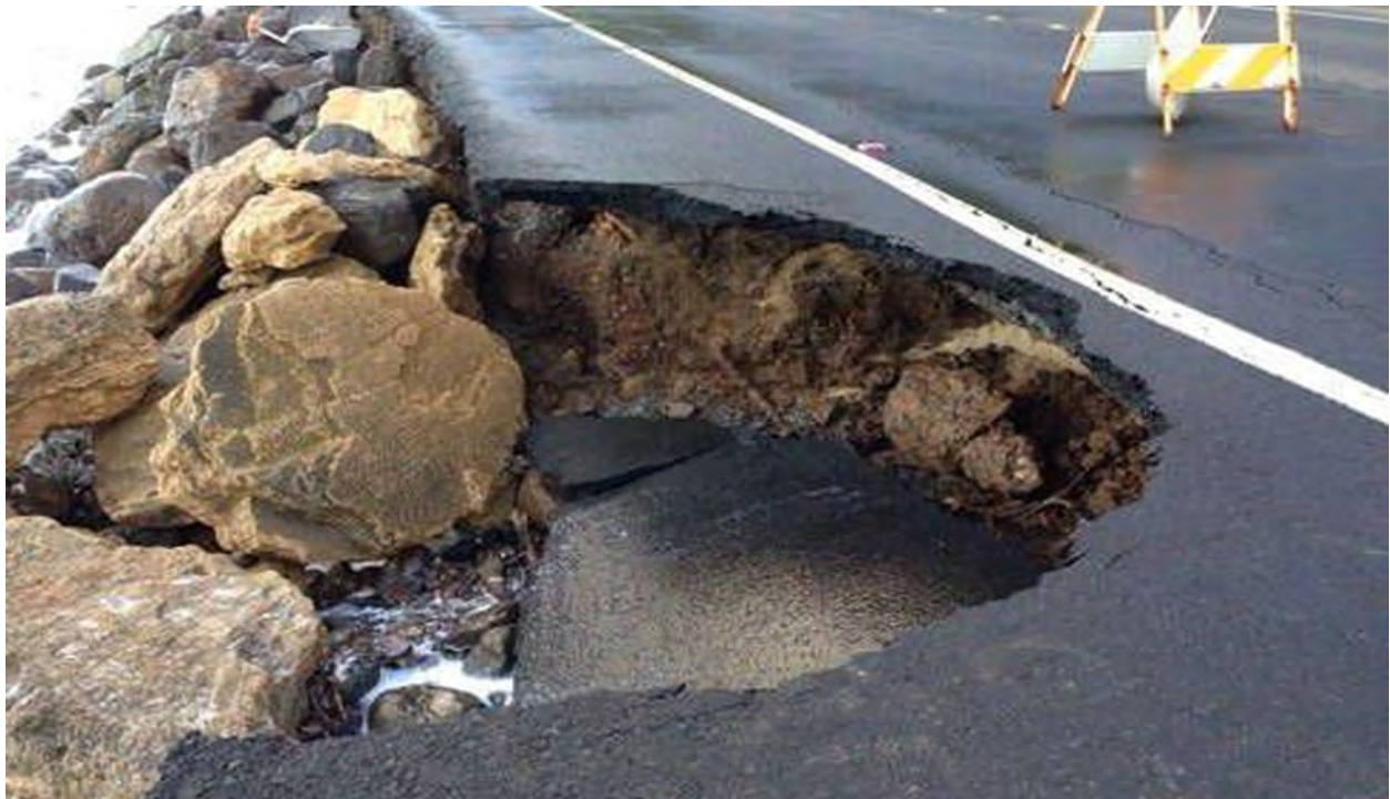
Figure 1-10. Undermining and collapse of a section of Kamehameha Hwy in Kaaawa, circa 2017.
