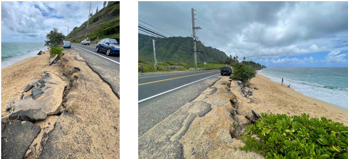
Figure 2-8. Condition of highway shoulder in vicinity of Kaoio Point, looking south ( left ) and north ( right )
