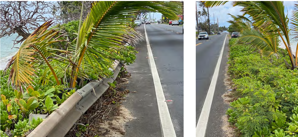
Figure 2-16. Condition of southern shoreline adjacent to highway shoulder, looking south (left) and north (right)
