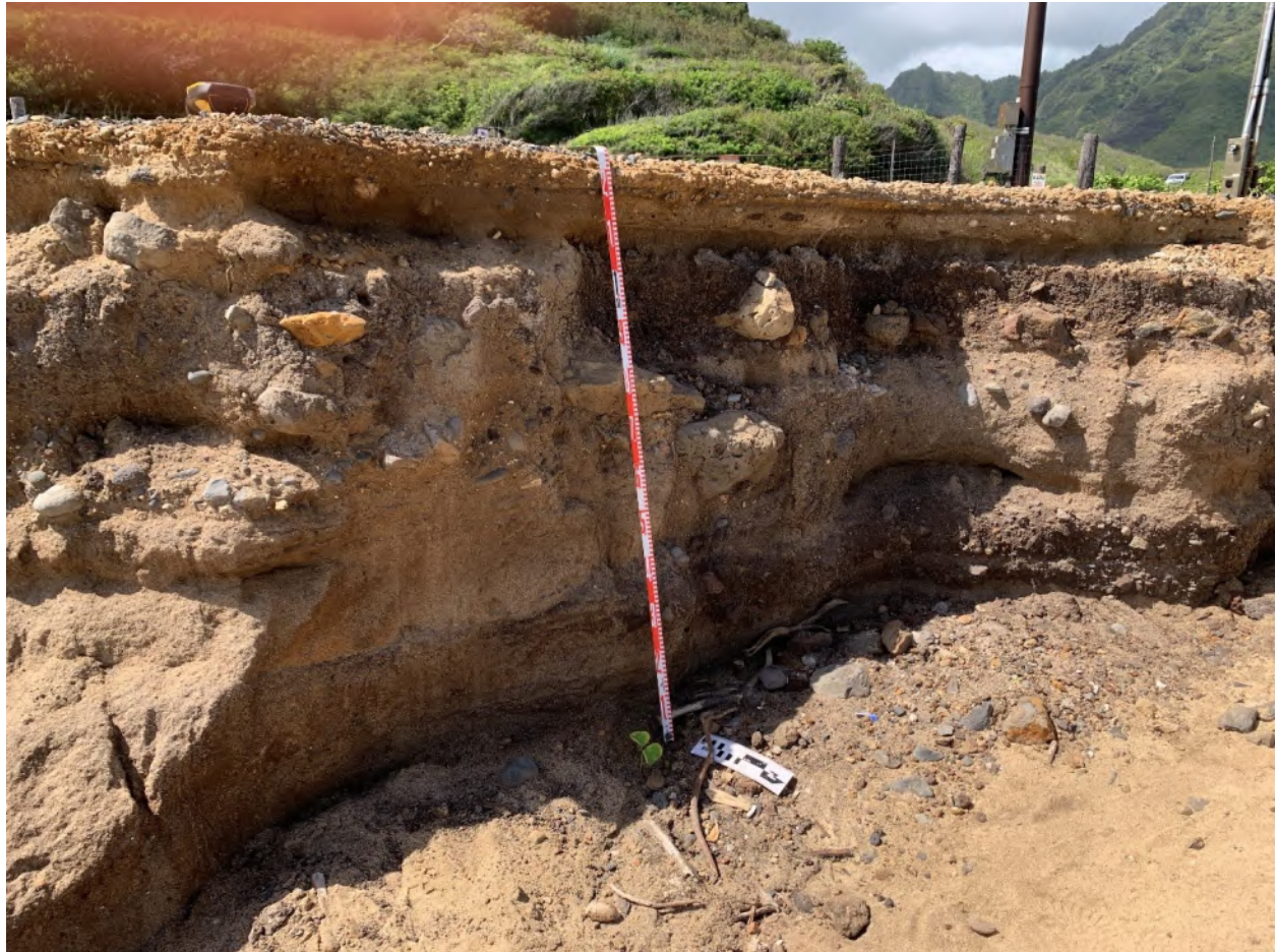
Figure 35. Severe beach-front erosion near the southern end of section 7, adjacent to Ka‘a‘awa Valley Road (near boundary of Ka‘a‘awa and Kualoa 2 Ahupua‘a); view southwest
