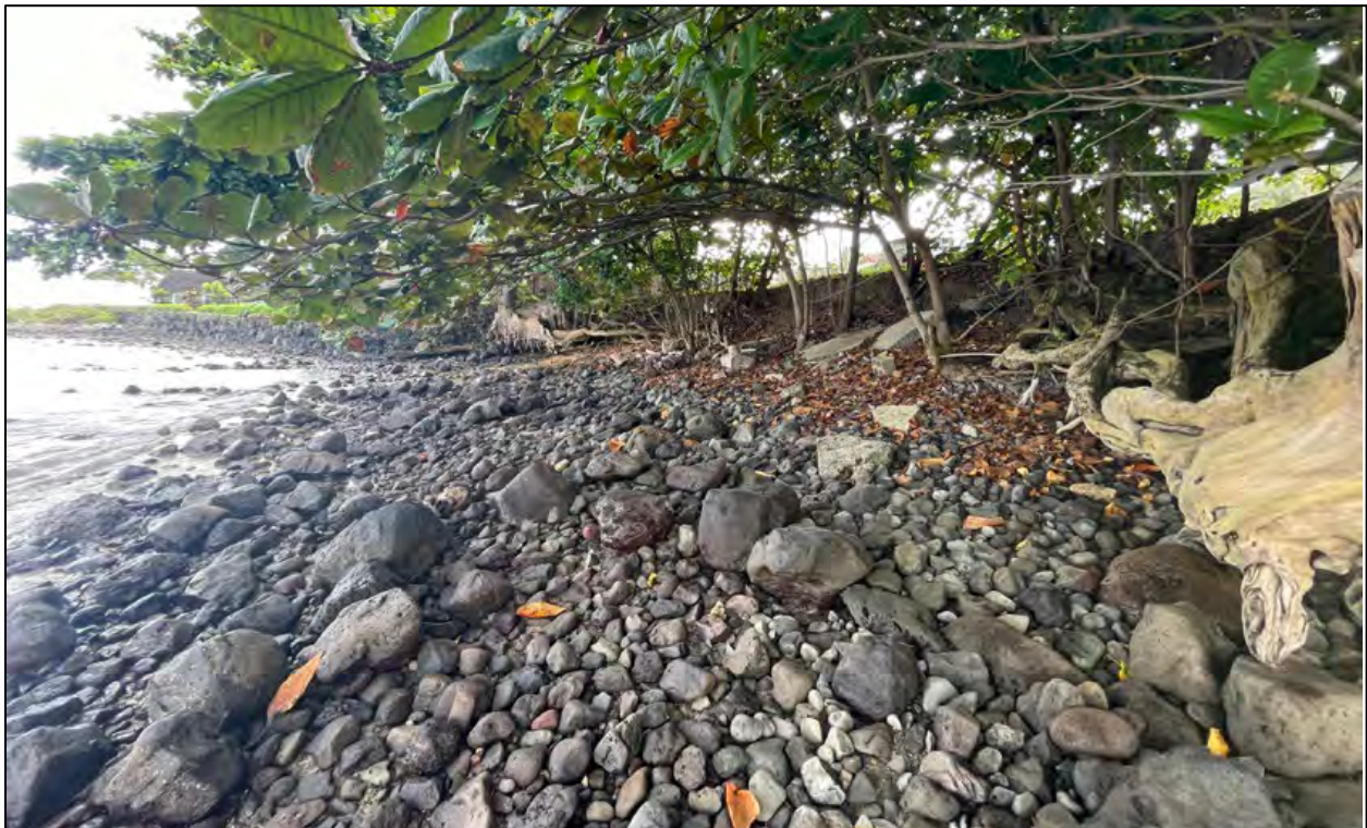
Figure 1-13. Sloped cobblestone and boulder beach and vertical erosion scarp cut into the native earthen embankment along the southern section of the Crouching Lion Project Site.
