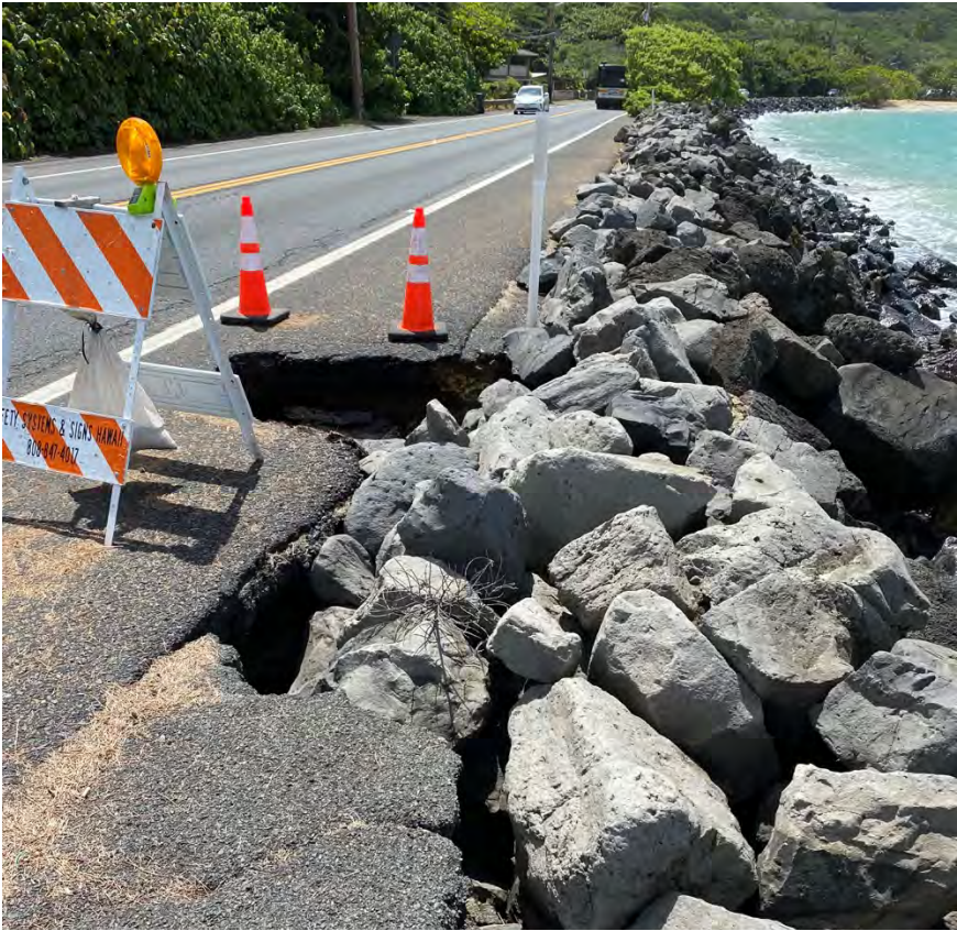
Figure 2-10. Sinkhole along the Kaoio Point to Kaaawa Stream repair site
