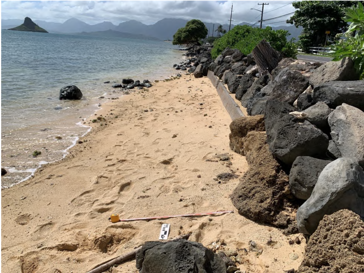
Figure 39. Retaining structures at northern end of section 8 (Kualoa 2 Ahupua‘a), makai of the old sugar mill ruins; view south
