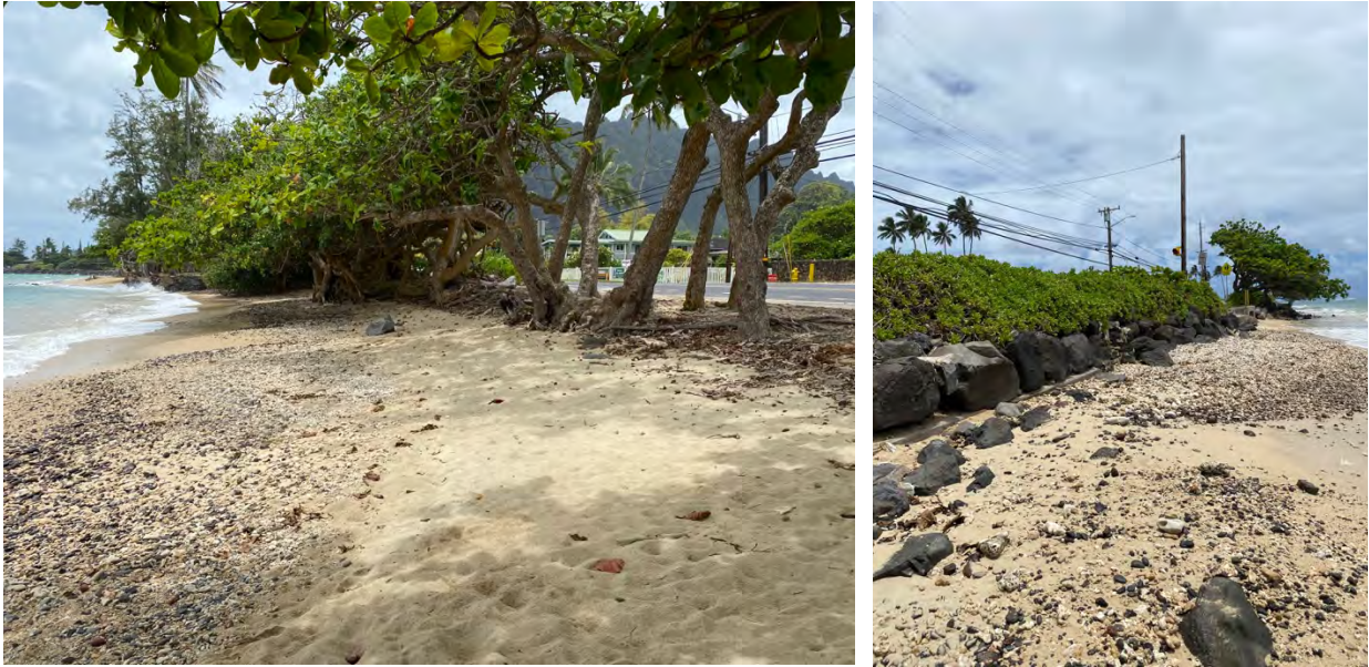
Figure 2-12. Condition of southern shoreline adjacent to highway shoulder, looking south ( left ) and north ( right )
