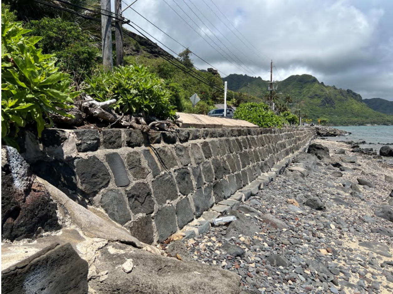
Figure 45. View of mortared rock wall (SIHP # 50-80-06-7922) dating from the original construction of the Kamehameha Highway in the late 1920s along the makai shoulder of the highway in section 4; facing north
