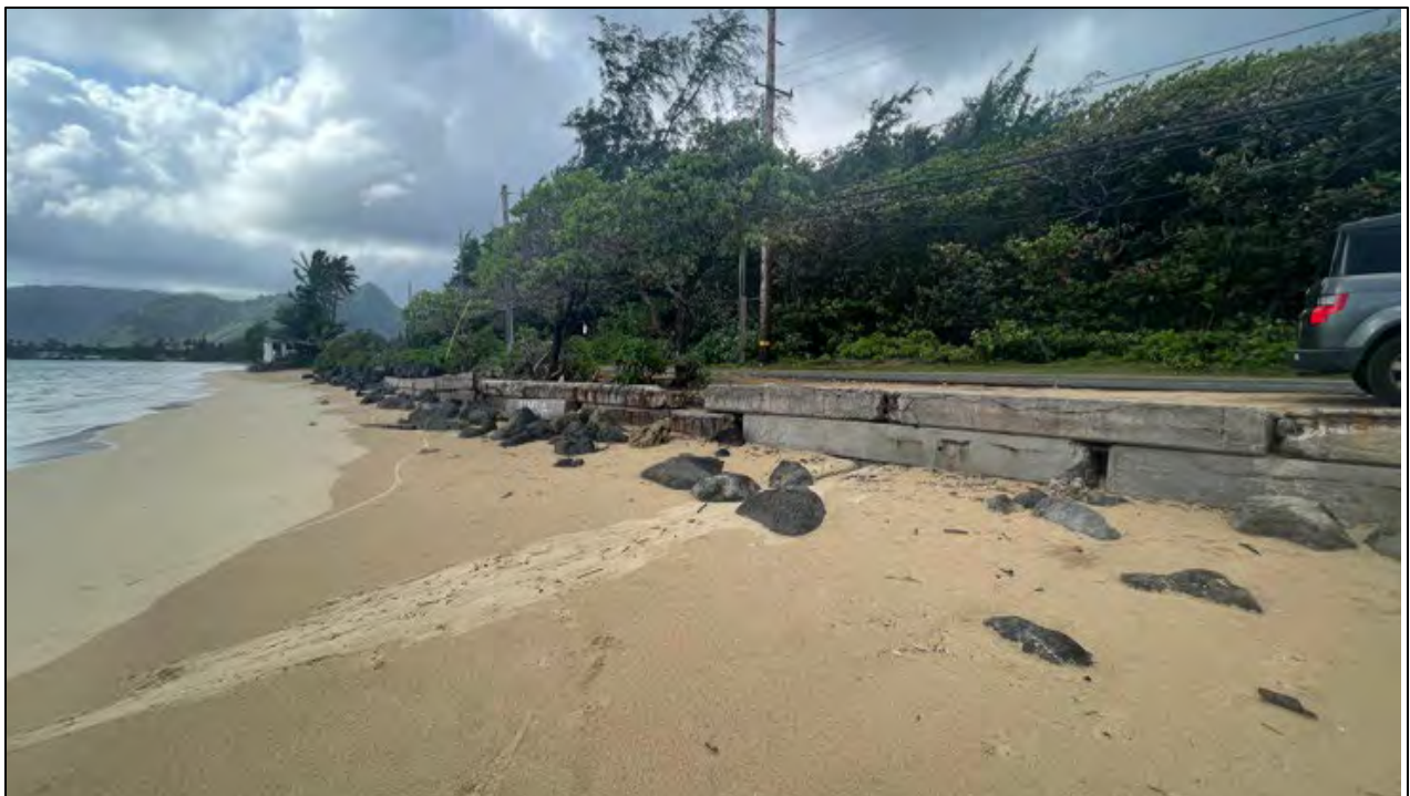
Figure 1-16. Stacked square concrete piles forming a seawall with riprap at Punalu'u North Project Site.
