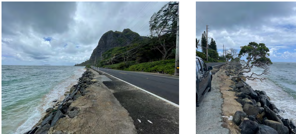
Figure 2-9. Condition of highway shoulder in vicinity of Kaaawa Valley, looking south ( left ) and north ( right )
