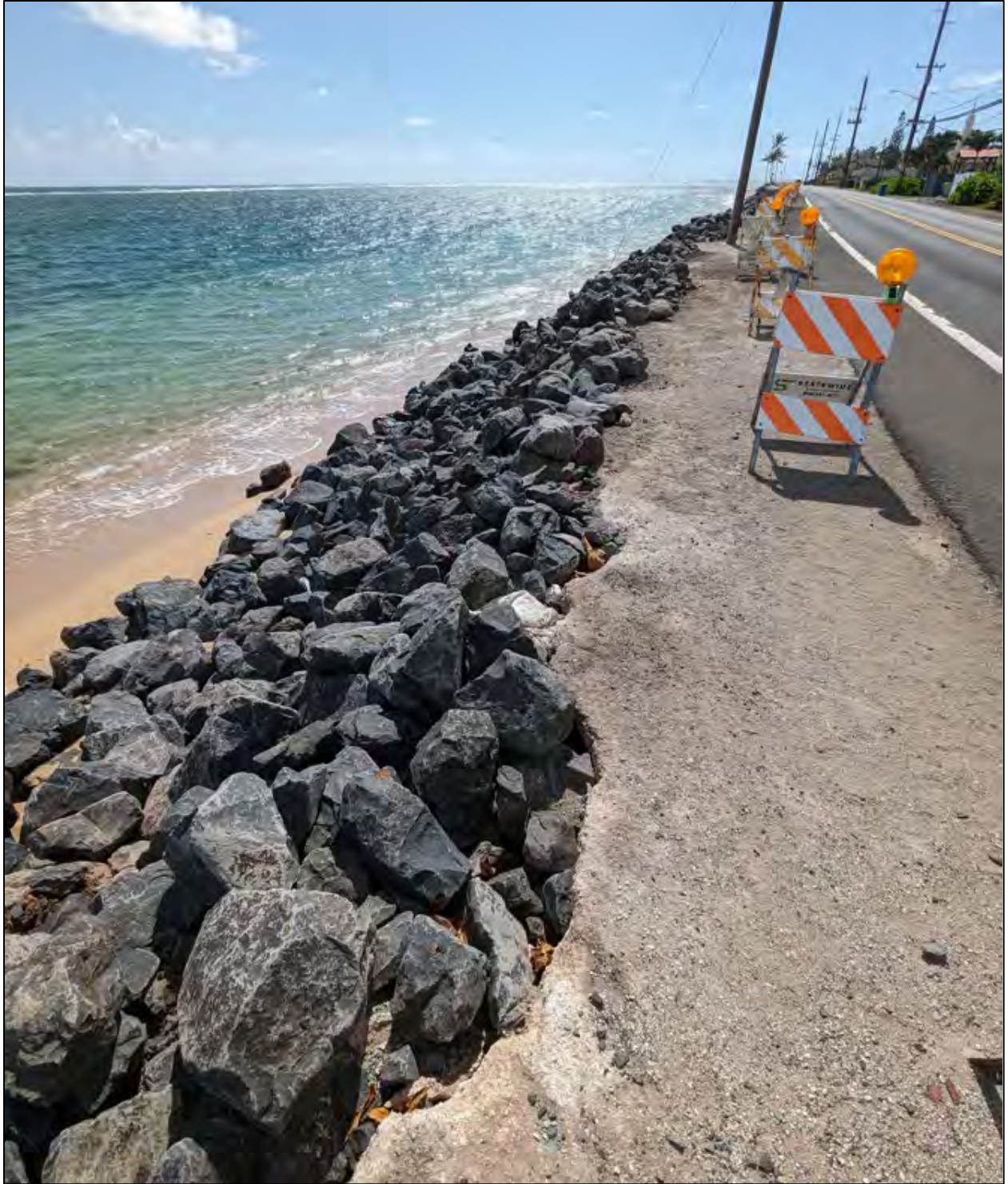
Figure 1-18. Non-engineered rock revetment at the Hau 'ula Project Site.
