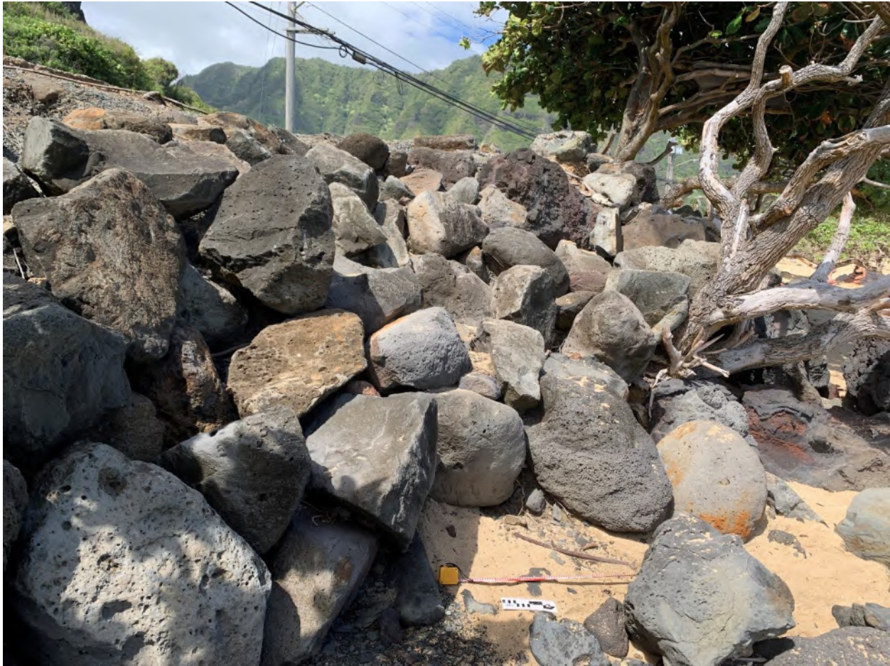
Figure 37. View of mitigation effort to combat severe beach-front erosion near the southern end of section 7, adjacent to Ka‘a‘awa Valley Road (near boundary of Ka‘a‘awa and Kualoa 2 Ahupua‘a); view west
