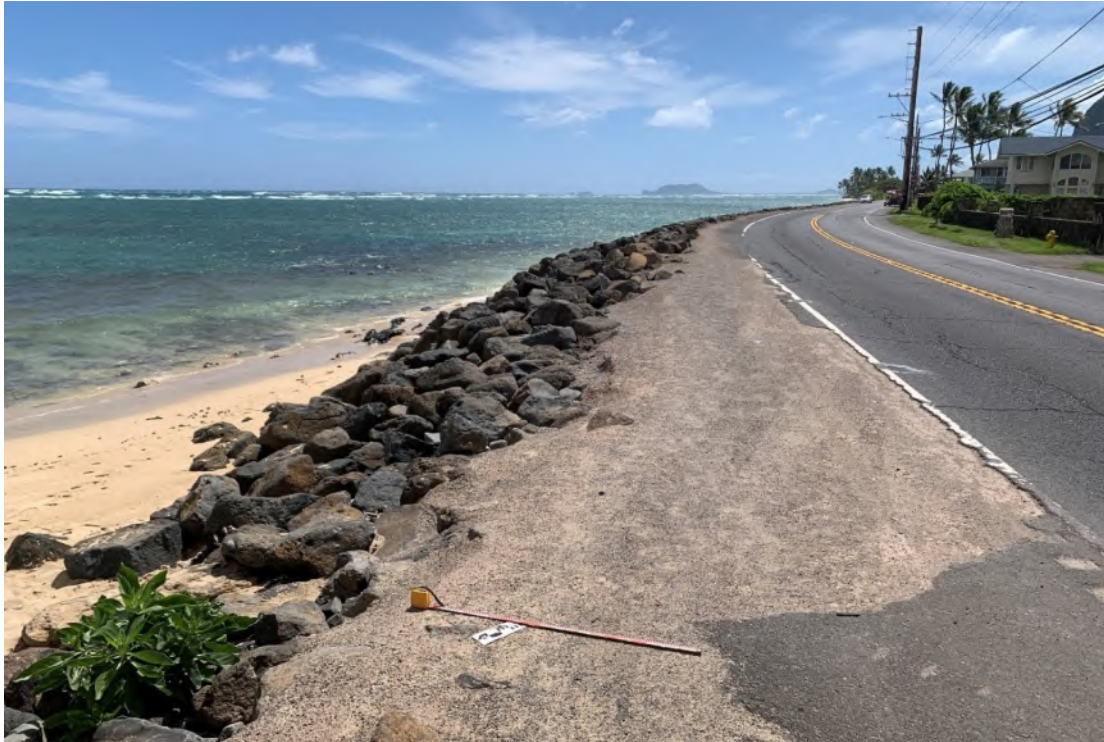
Existing boulder revetment just south of Swanzy Beach Park, Ka‘a‘awa; view southeast
