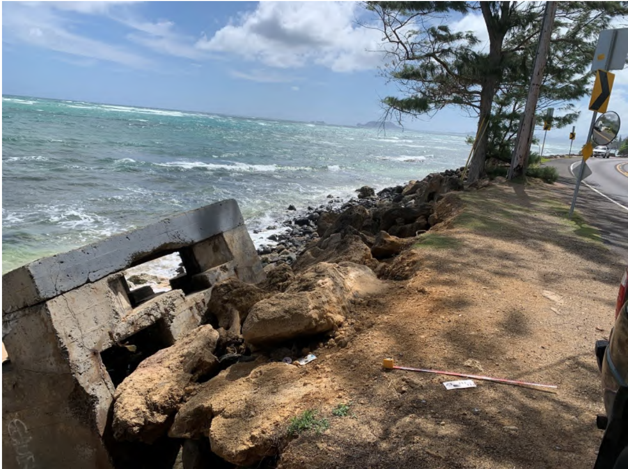
Figure 34. Failing retaining-wall structure at the southern end of Ka'a'awa Bay (Ka'a'awa Ahupua'a), middle of section 7; view east-southeast
