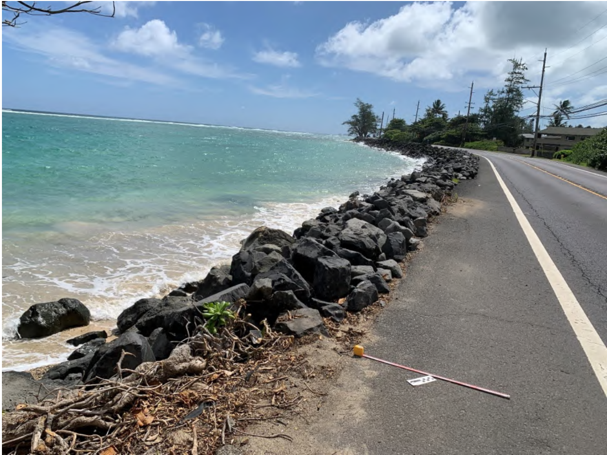
Figure 33. Boulder sea-wall structure at the southern end of Kalae‘ō‘io Beach Park (near northern end of section 7), Ka‘a‘awa Ahupua‘a; view southeast
