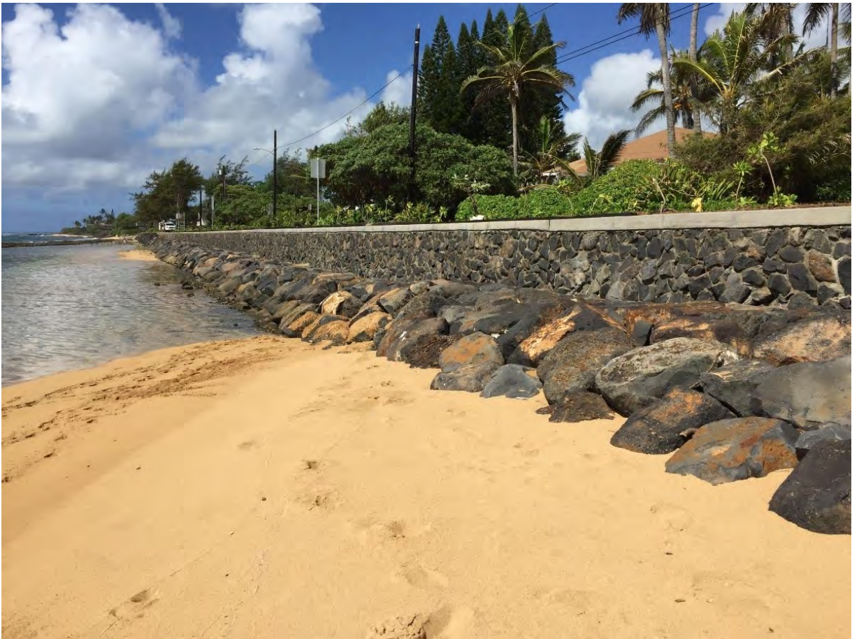
Figure 6-2. Example of existing hybrid seawall with rock apron (armored toe), Kapaa, Kauai
