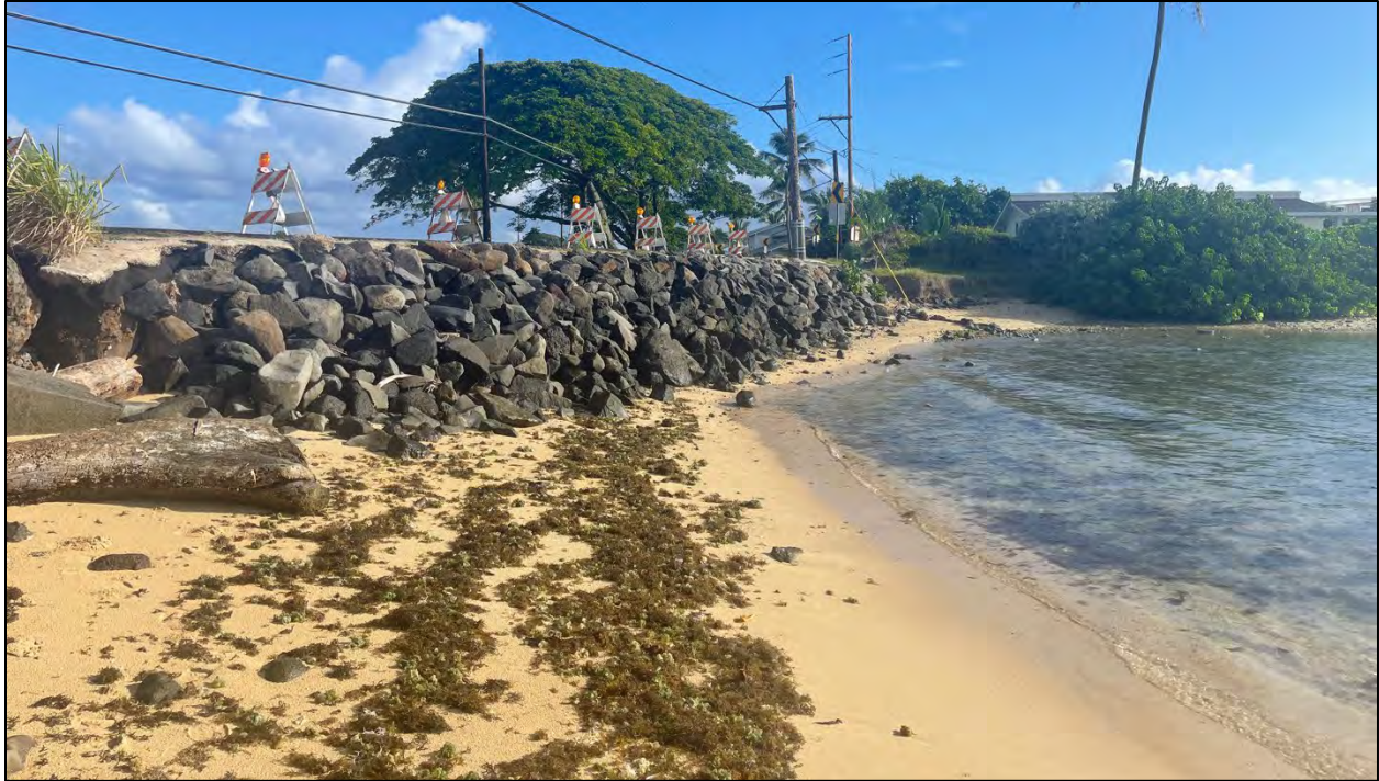
Figure 1-6. Kualoa Park Project Site. Erosion under the highway and non-engineered emergency riprap protection.
