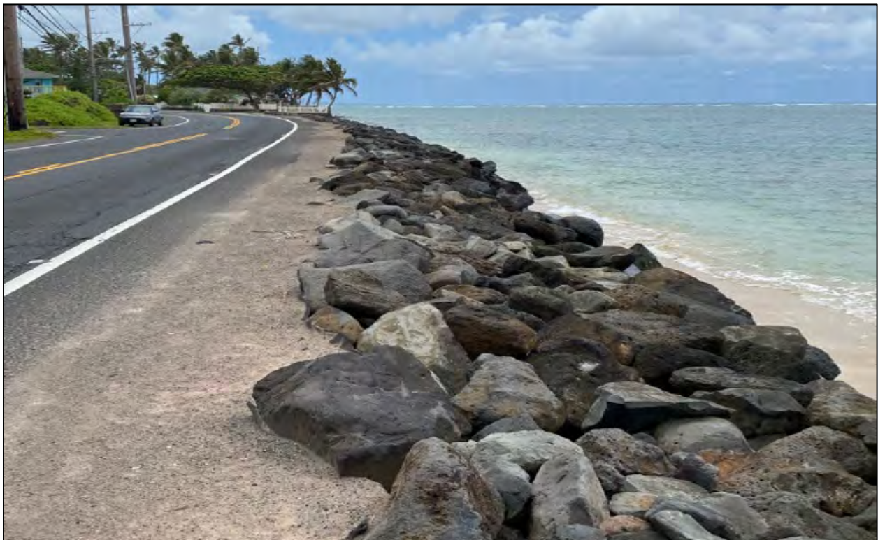
Figure 1-12. Riprap directly abutting paved roadway shoulder in the northern portion of the Puakenikeni Road Project Site.
