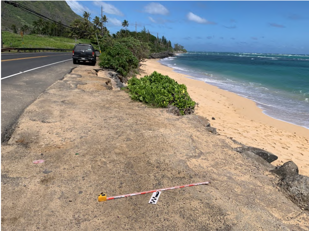
Figure 36. View from the roadway of severe beach-front erosion near the southern end of section 7, adjacent to Ka‘a‘awa Valley Road (near boundary of Ka‘a‘awa and Kualoa 2 Ahupua‘a); view north
