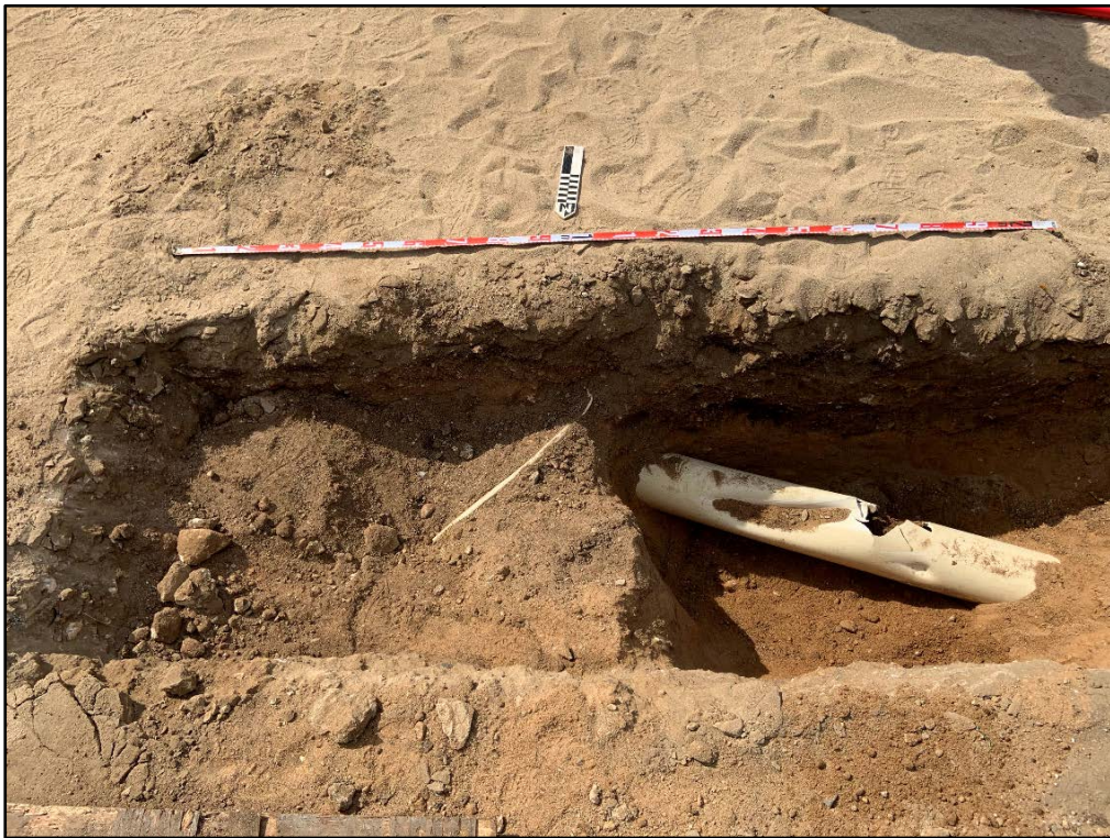
Figure 54. Plan view of T-11 showing broken PVC sewer drain pipe; view to south
