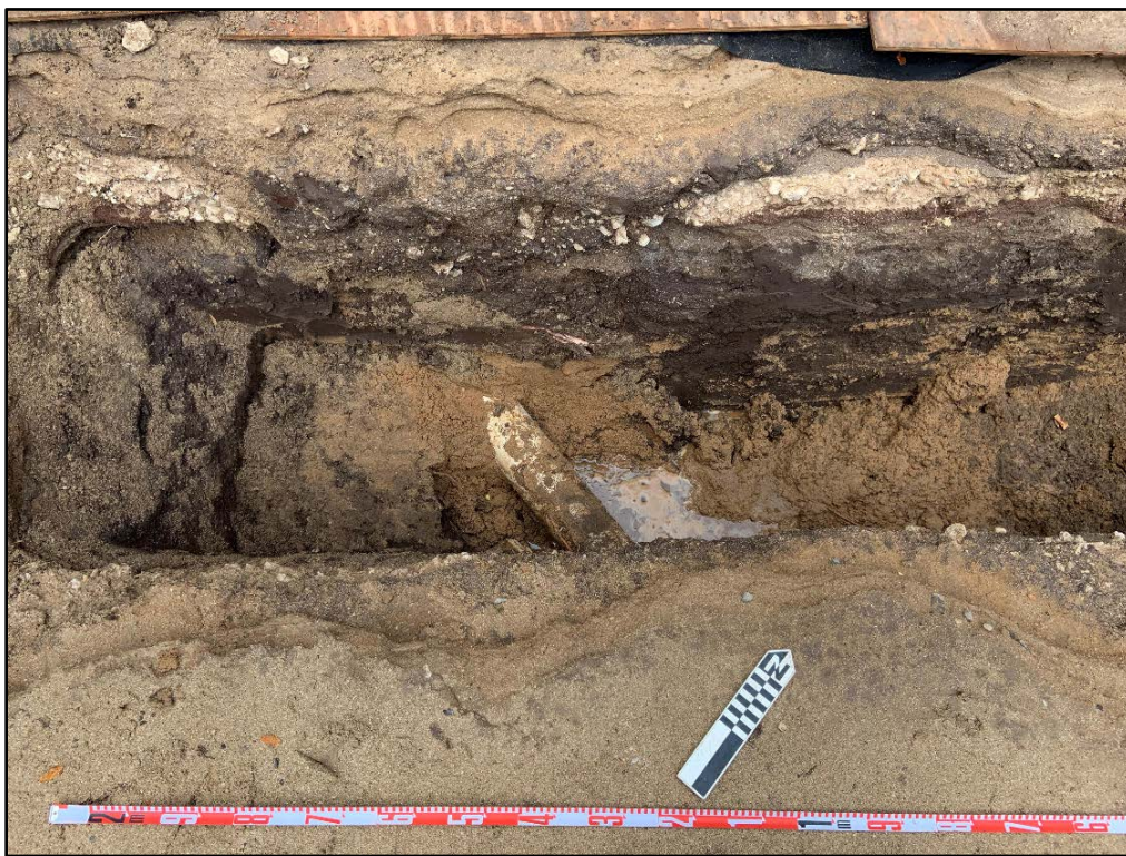
Figure 60. Southwest end of T-13 showing broken PVC fire sprinkler line at 1.13 mbs
