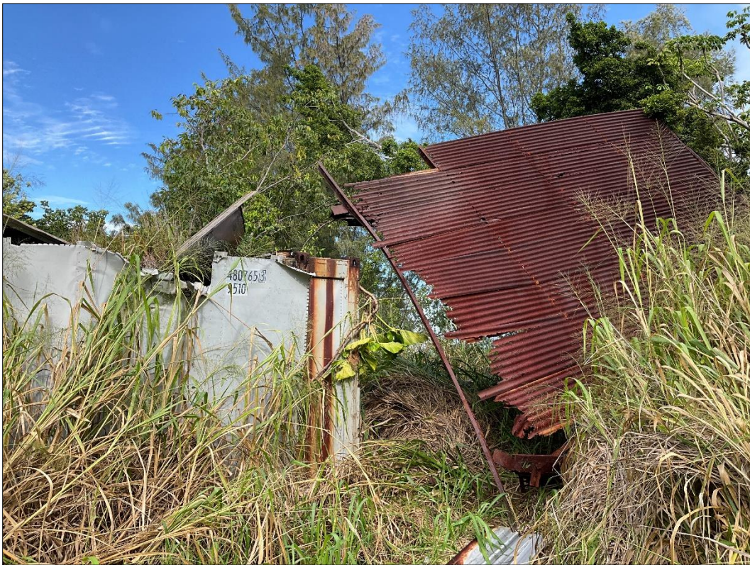
Figure 63. Feature B, collapsed building, view to the northwest.
