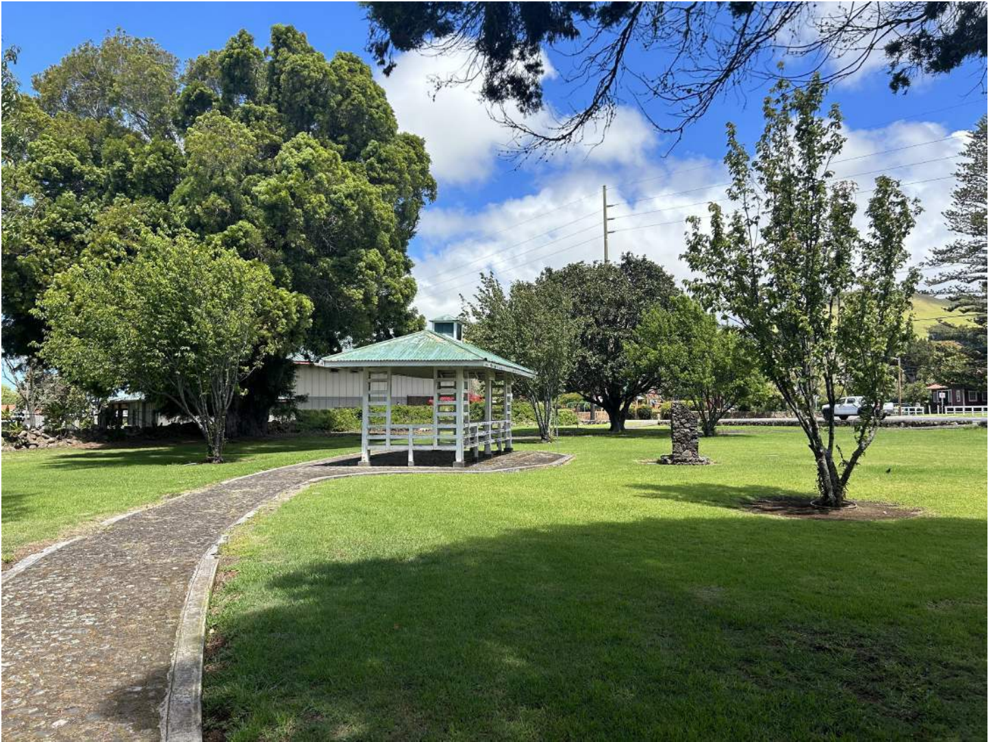
Photo 4: Corner of southeast and northeast elevations of gazebo, viewed from southeast walkway.
