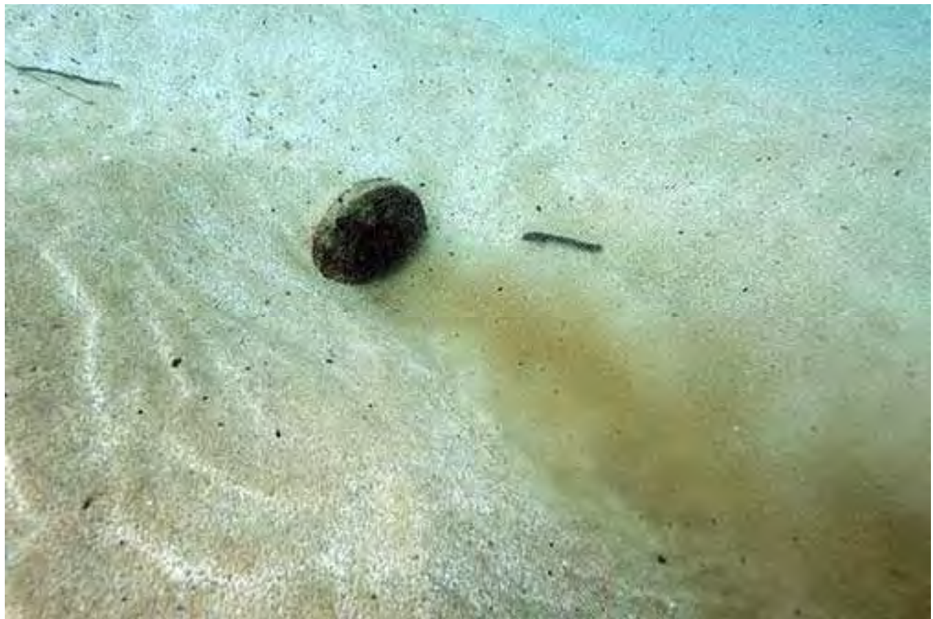
FIGURE 3. Photographs of partially buried Wailua Wastewater Treatment Plant ocean diffuser ports discharging effluent on December 23, 2016.
