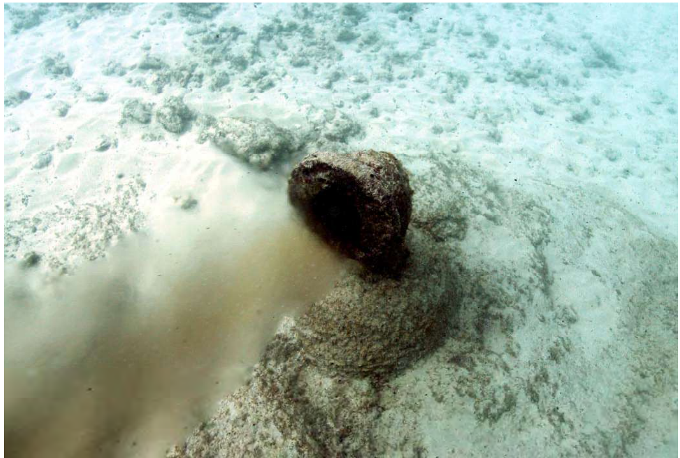
FIGURE 4. Photographs of two Wailua Wastewater Treatment Plant ocean diffuser ports discharging effluent taken on September 21, 2012. Note difference in sand cover of the area compared to photos taken in 2016 (Figures 2 and 3).
