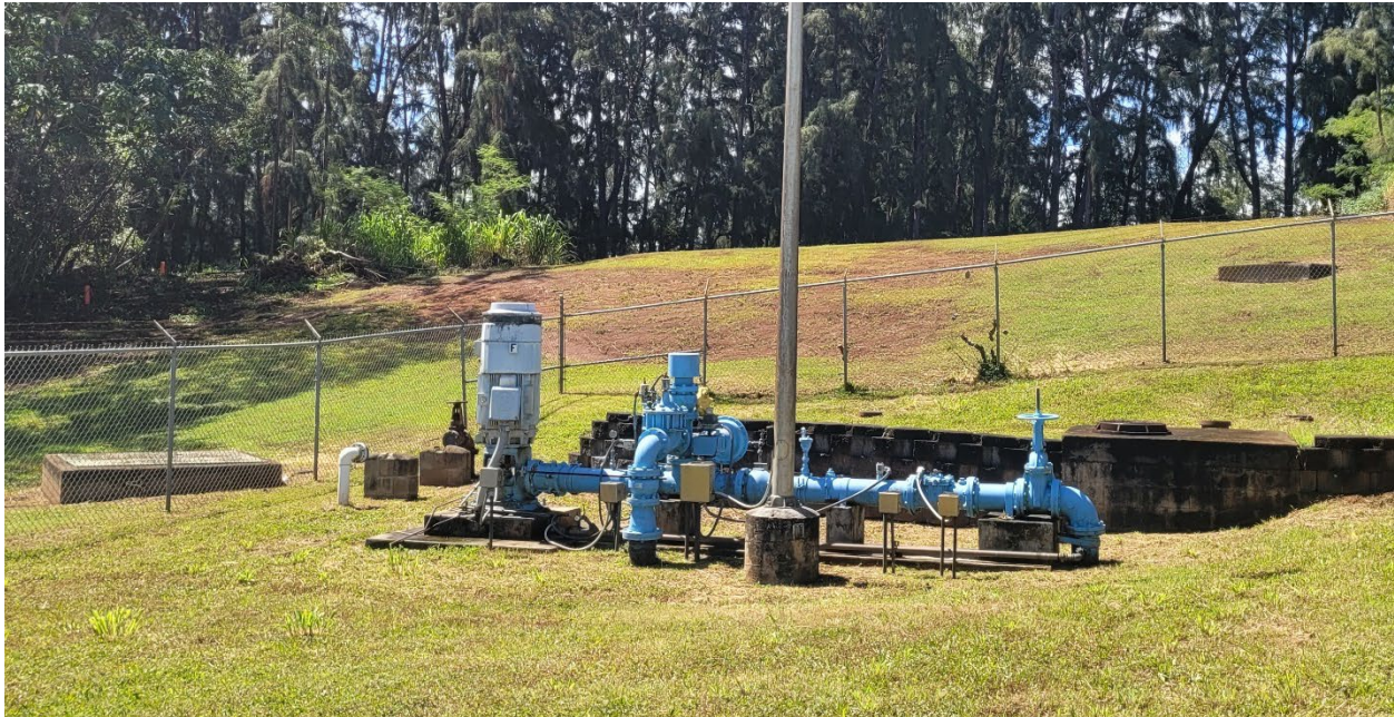
Figure 2-6: Example of Production Well
