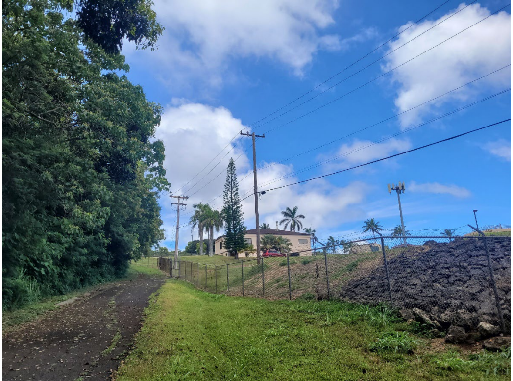
f. View of existing Hawaiian Electric power lines and poles in vicinity of proposed tap.
