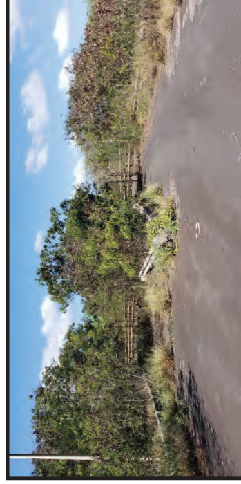
Figure 20. Overview of the split in the paved loop road in the northeastern portion of the facility for two weigh stations, looking northwest
