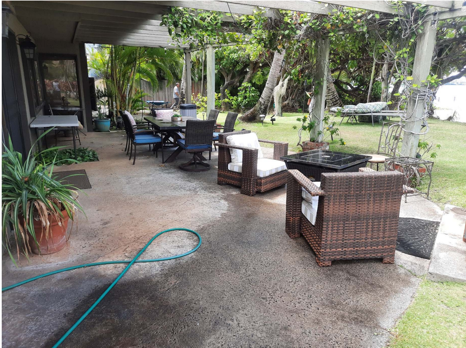
Figure 13: Milled-wood pergola attached to the two-story, masonry framed structure covering the concrete patio (view to south)
