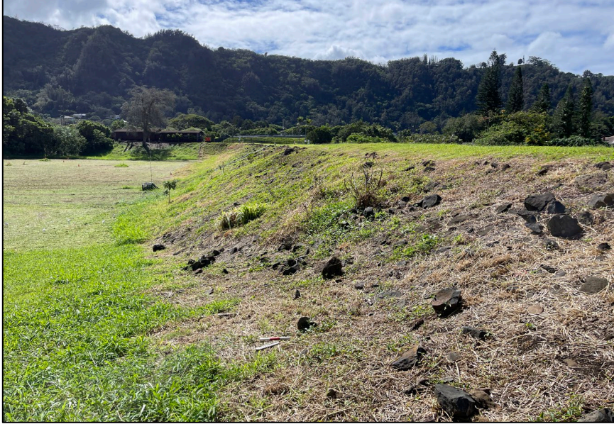
Figure 19. Feature 6 Nu‘uanu Reservoir No. 1 (reservoir on the left and embankment on the right), facing southeast.
