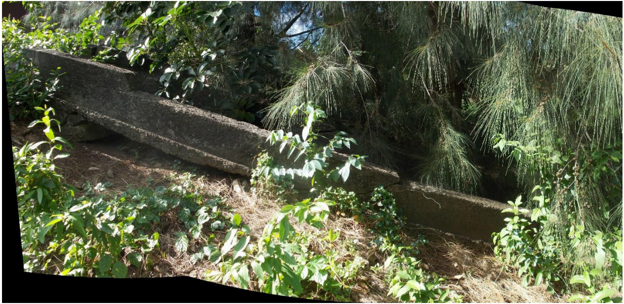
Figure 13. Concrete sluice on the southeast side of the reservoir. View facing southwest.
