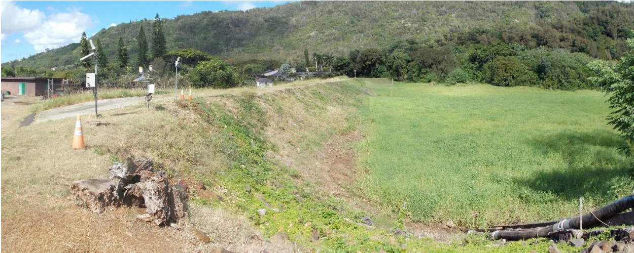
Figure 3. Overview of the Nuuanu Reservoir No. 1 Dam with a view of the upstream slope. Impoundment is on the right. View facing northwest.
