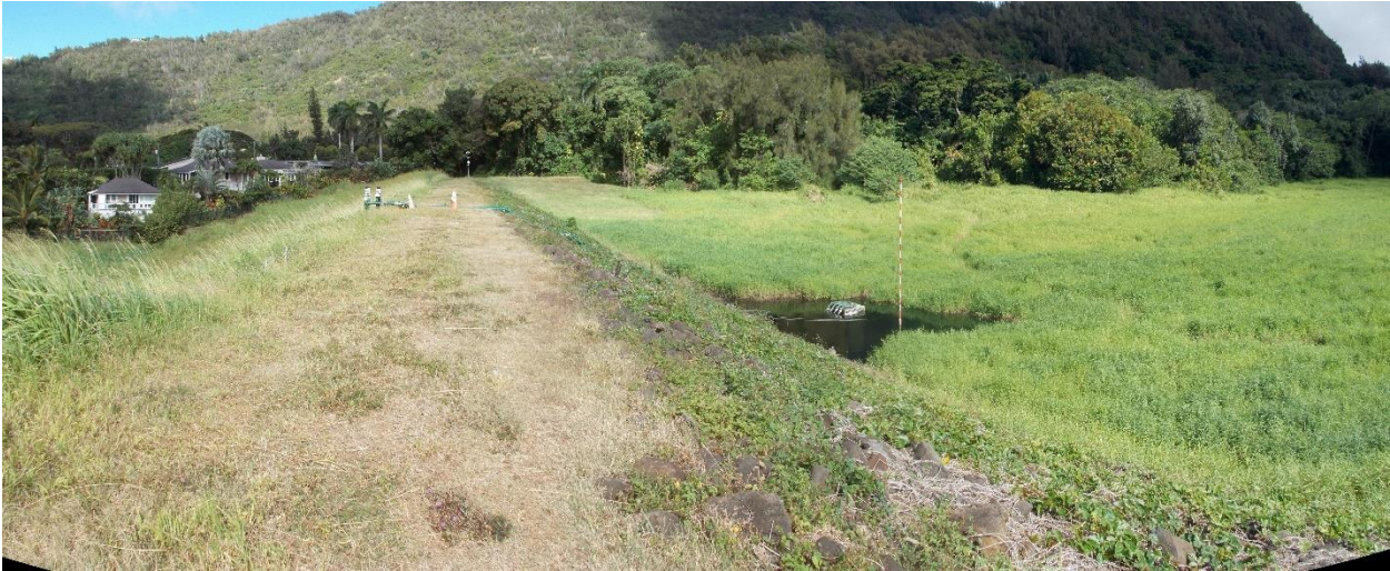
Figure 4. The crest of the dam. Note the open water of the sump and the impoundment on the right. View facing northwest.
