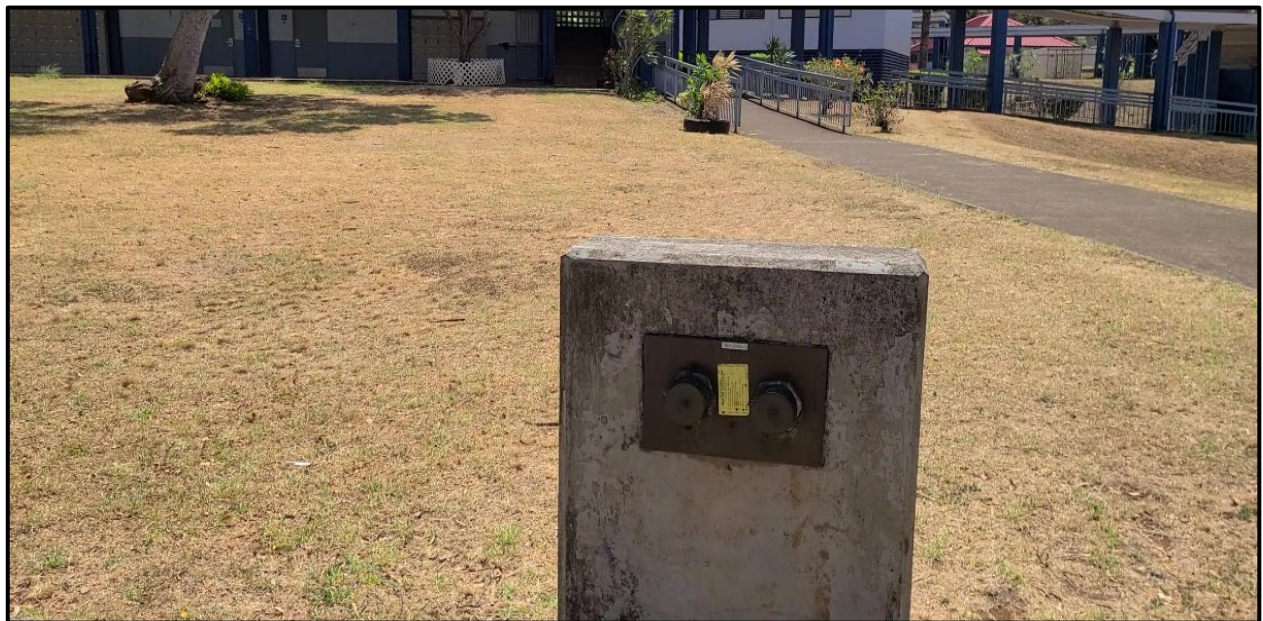
Figure 12. Dry standpipe monument near southwest corner of project area, view to the southeast.
