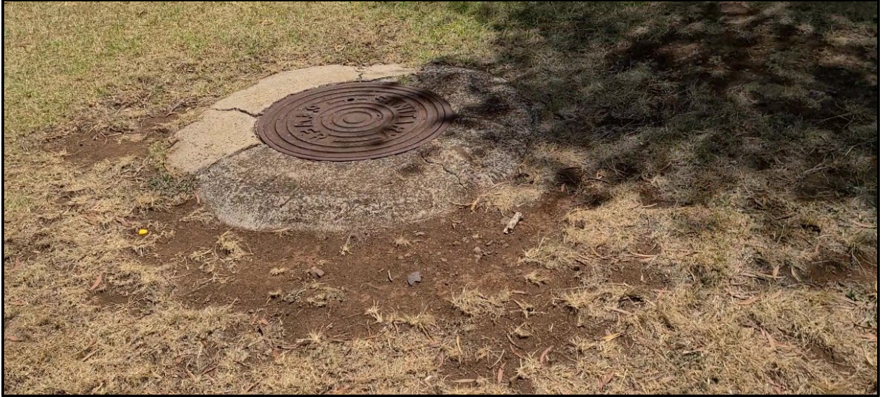
Figure 13. Sanitary sewer manhole in central portion of project area, view to the west.
