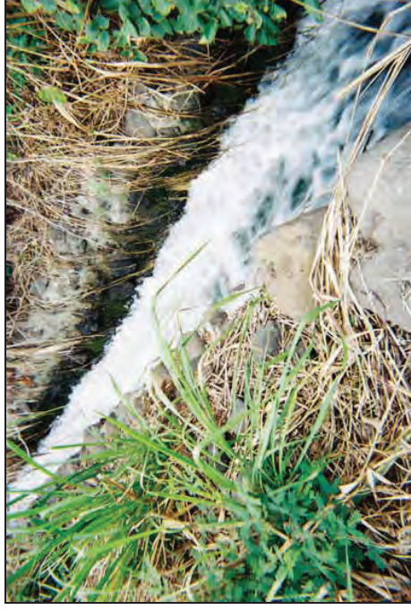
Figure 14: Site 50-50-04-5729 Ditch, Showing Rock and Mortar Construction of Side Walls. View to Northwest.
