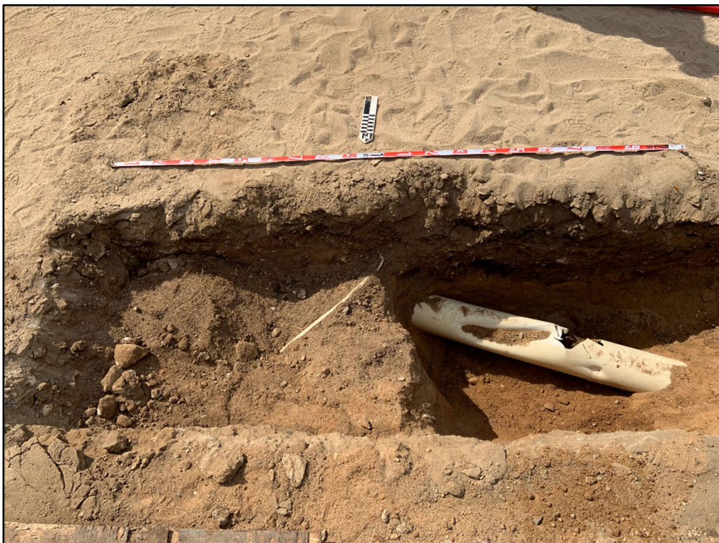
Figure 54. Plan view of T-11 showing broken PVC sewer drain pipe; view to south
