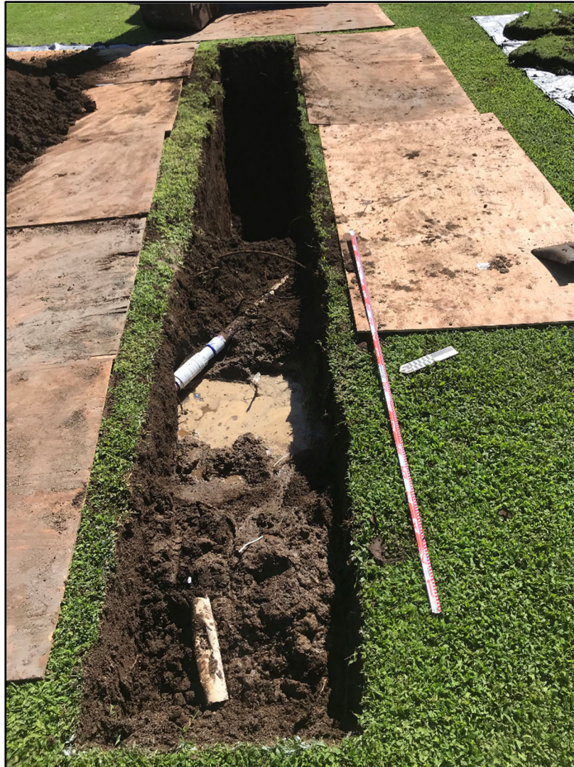
Figure 37. Profile of T-4 overview at BOE depicting water line and unexcavated area; view to east
