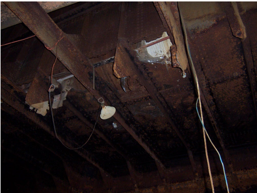
Wasted deck and scantlings below boiler flat, Tank #1 starboard.
