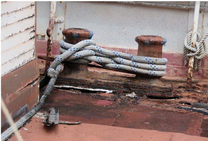
Wasted double bitts, fir foundation and deck badly corroded and rotted. Unsafe, yet still securing vessel under load.
