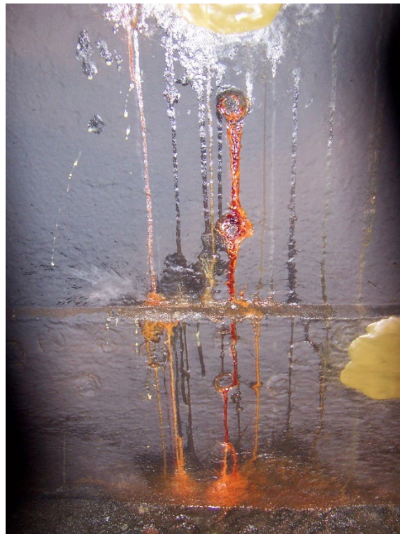
Leaking rivets and patches in Tank #4 starboard.
