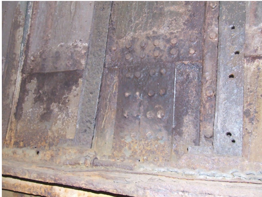
Wasted or non-existent rivets on transverse framing in Pump Room, port side looking aft.
