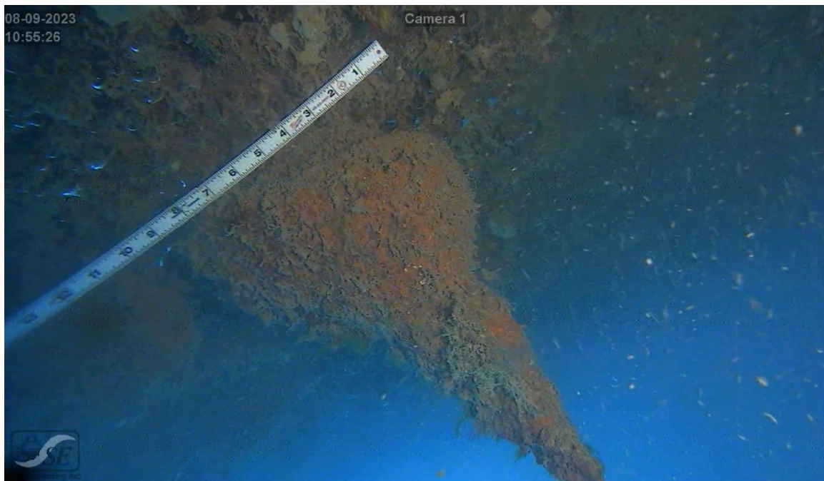
Figure 2: Cone shaped corrosion stalactite varied in size, up to 12 inch in diameter and 18 inch in length.
