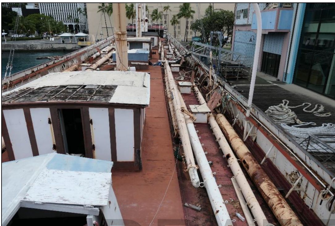
Figure 7: The corroding, dry-rotted and crowded decks of the ship are in danger of collapse, March 2023 (Joseph Lombardi), source: Delgado, “The Four-Masted Ship Falls of Clyde.”
