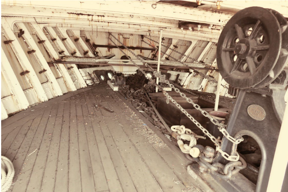
Chains installed in 2008 to support forward collision bulkhead. Transverse steel beams welded across space to pull side shell plating in.
