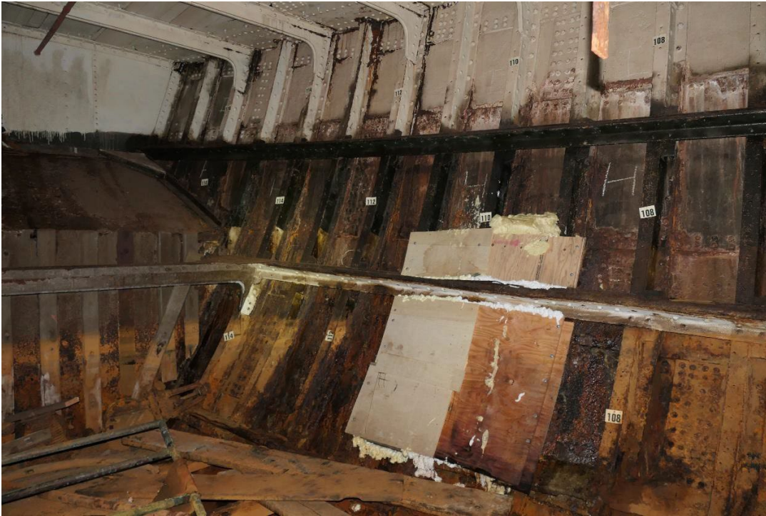
Figure 5: Patches cover more substantial leaks, but water infiltration is also resulting from loss of up to fifty percent of hull plating thickness in many areas, lost rivets, and rainwater entering through the decks (Joseph Lombardi), source: Delgado, “The Four-Masted Ship Falls of Clyde.”
