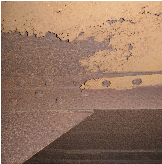
Overhead plate scaling in Tank #3 starboard..
