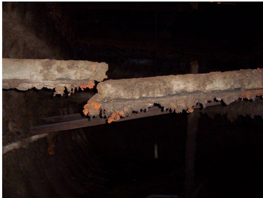
Tripped or broken horizontal support in Tank #3 starboard.
