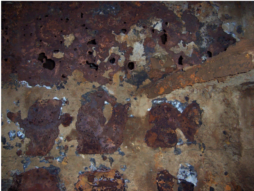
Wasted bulkhead in Tank #1.
