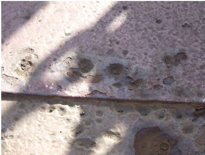
Typical pitting action on maindeck, showing failed paint system.
