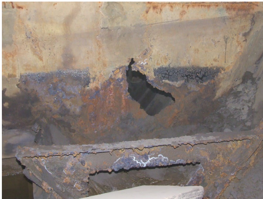
Holed main aft bulkhead into Tank #1 port.
