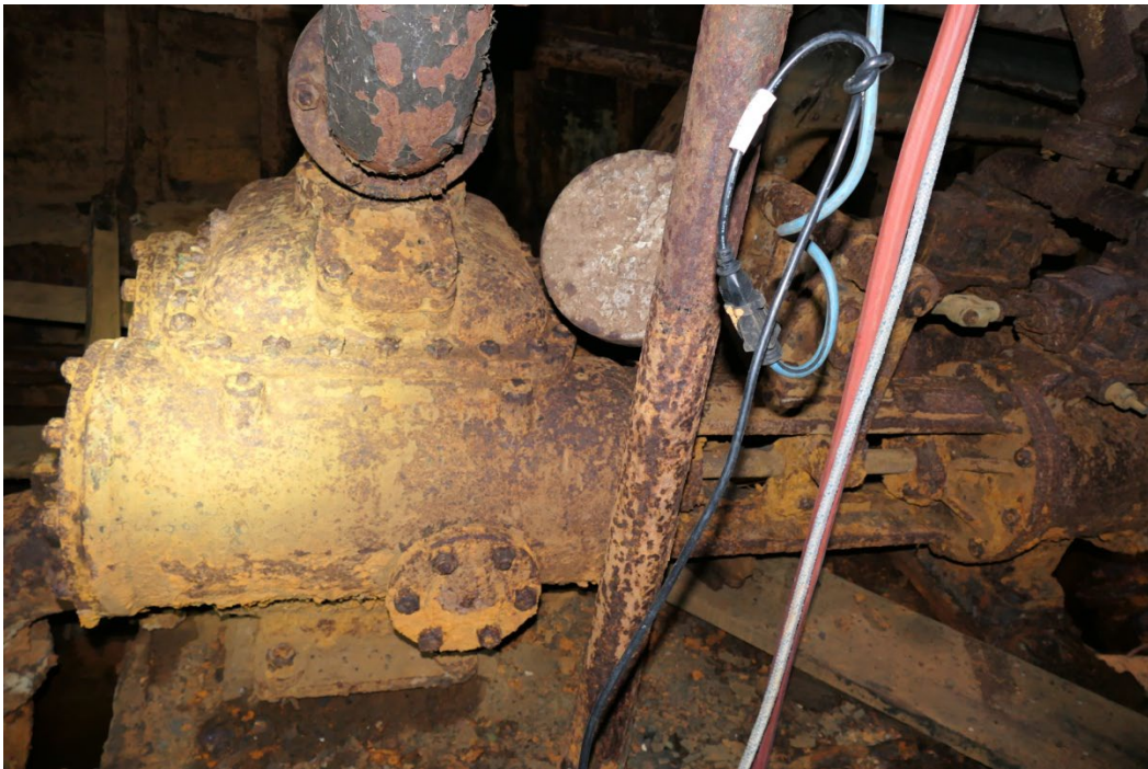
Main steam pump, totally wasted with rust/scale.
