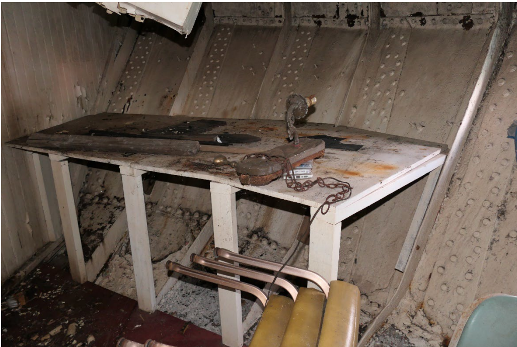
Small cabin to port at the counter showing overhead sagging down at top of photo and poorly maintained inner hull facing.
