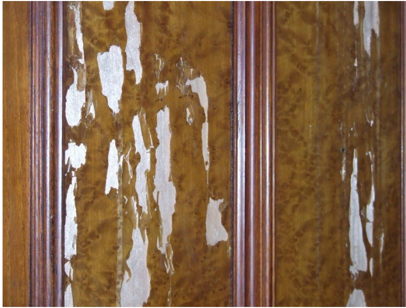
Delaminated veneer in main salon.
