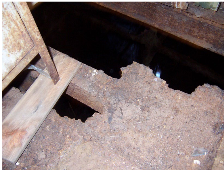
Wasted intermediate platform in Tank #2 port.
