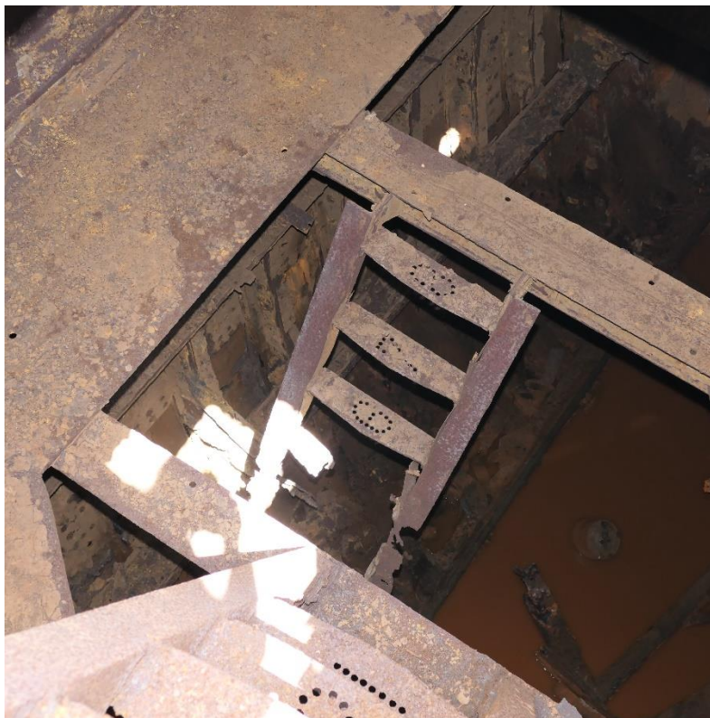
Figure 15: Corroded and partially flooded tank (Joseph Lombardi).
