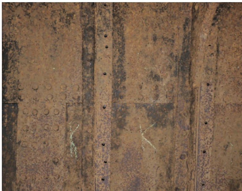
Tank #4 starboard showing wasted side shell plating and non-existent rivets.
