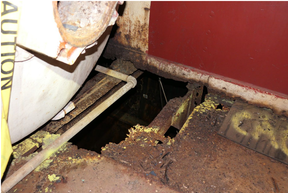
Boiler-room, holed plating to port under boiler.
