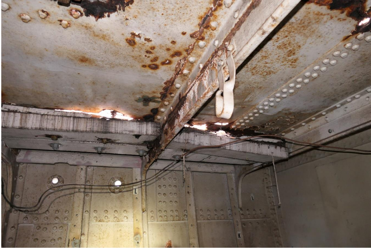
Figure 12: Corrosion has opened holes that have accelerated corrosion inside the ship as well as outside of the vessel (Joseph Lombardi).
