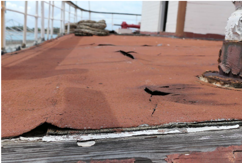
De-laminated sheathing on poop deck.
