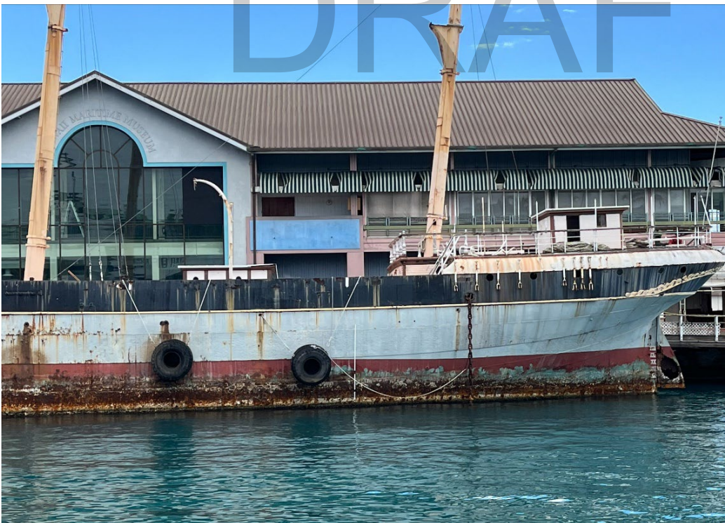
Figure 2: Condition of the hull, rudder, and standing rigging on mizzen and jigger masts, February 20, 2024 (Melia Lane-Kamahele, NPS)
