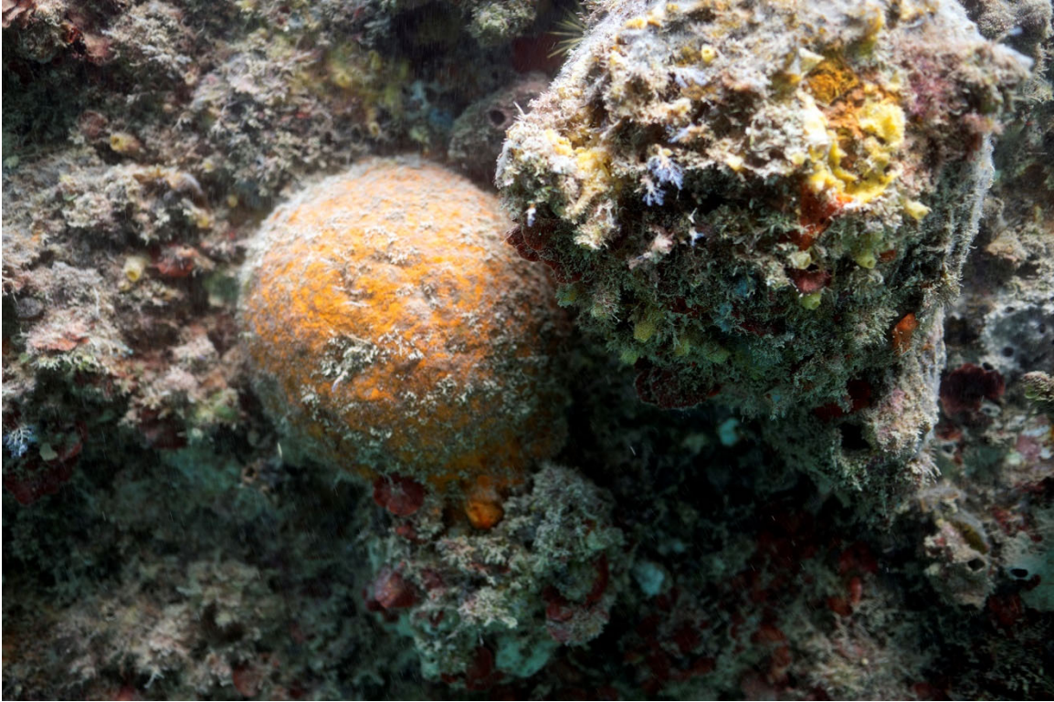
Figure 4 Spherical Protrusion Consisting of Rust on the Hull of the Falls of Clyde.
