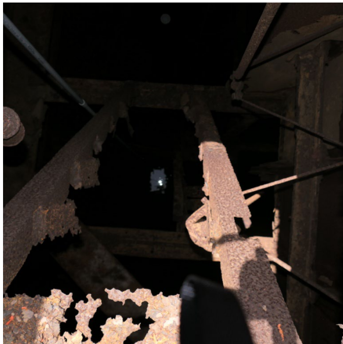
Wasted ladder entering #3 Tank to starboard.
