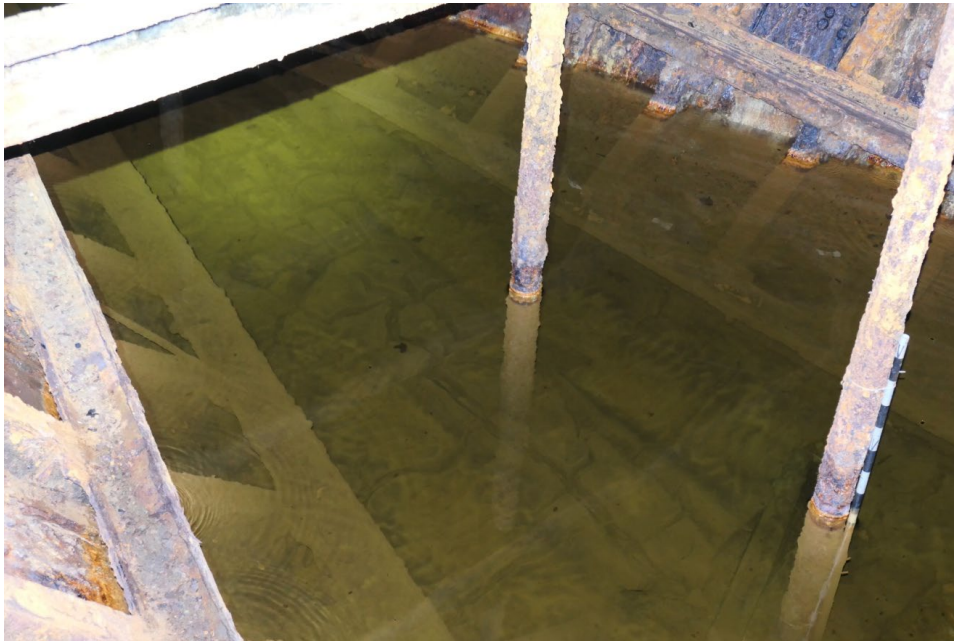
Flooded lower flat of Aft Peak Tank.
