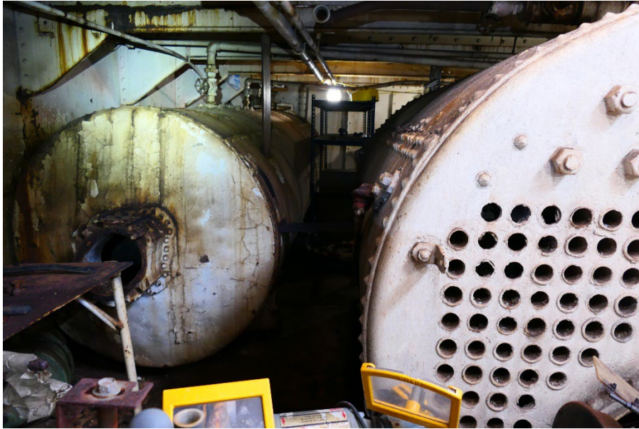
Boiler-room, looking aft to port.
