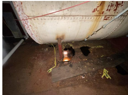
Photo #4, below deck wastage
