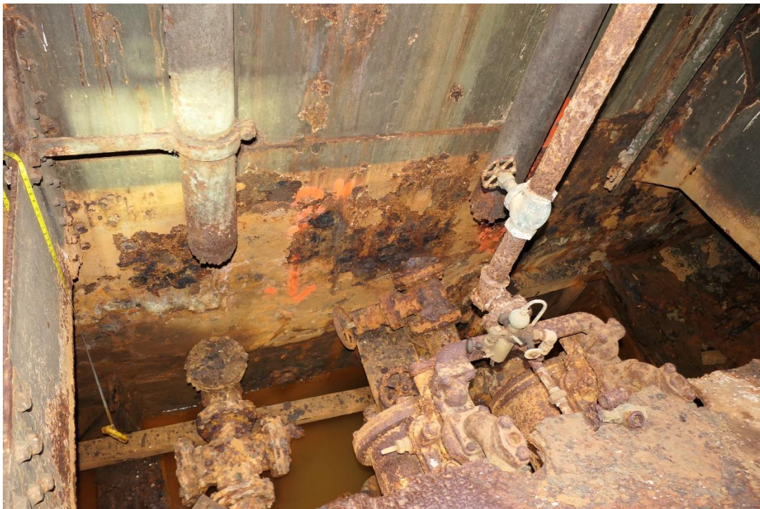
Figure 14: Corroded machinery and piping in 2023 (Joseph Lombardi).
