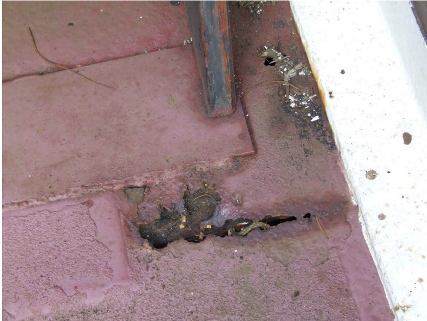
Wasted deck at foot of ladder aft to starboard.
