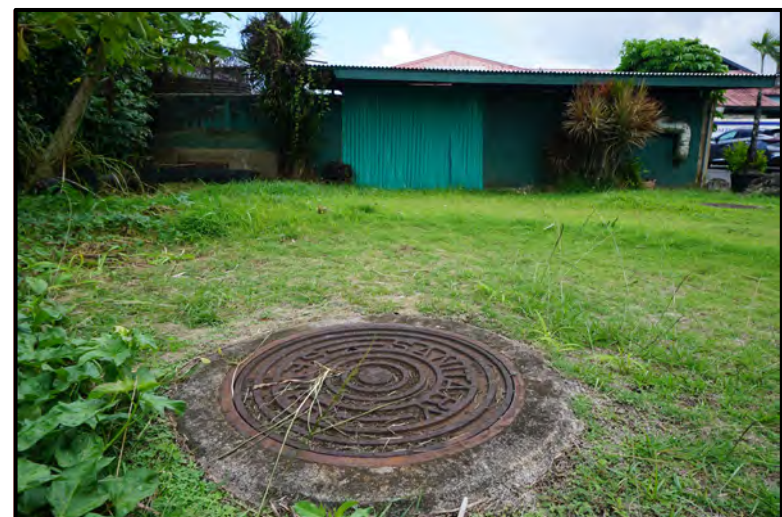
Photo 4: View of existing backup injection wells and existing WWTP enclosure. Facing east
