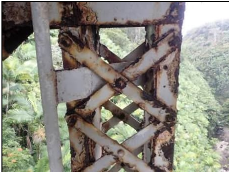
Photograph 44. Bent 3 Level 1, Column D Vertical near top - Corrosion, typical laminar at upper levels (CS 3)
