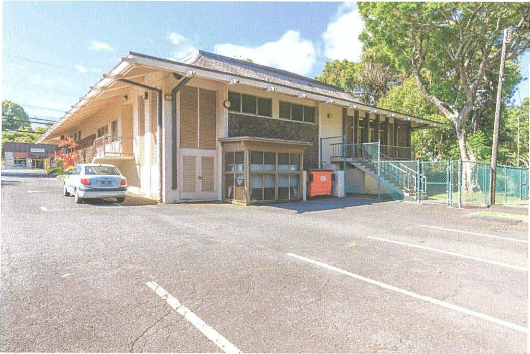
Photograph 2. West View of Building Corner. Four Parallel Parking Stalls on Left of Building to be Removed.
