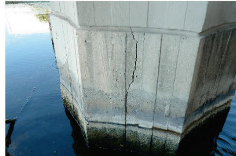
Photo 5: Example of structural damage from corrosion to Capitol column. (AHL, 2015)
