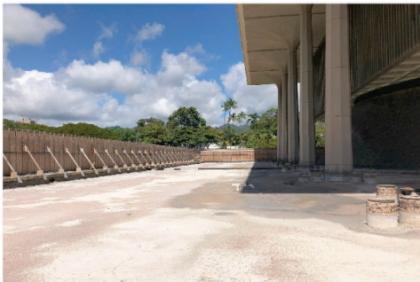
Photo 6: Existing condition of the Ewa Capitol pool, looking mauka. Repairs to basin surface not started. (HHF Planners, 2024)
