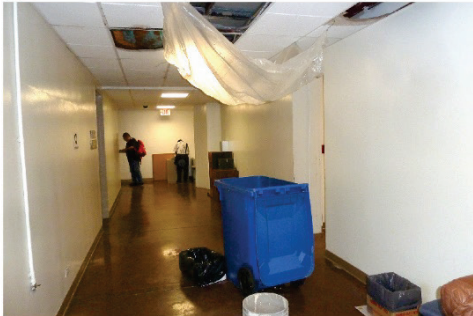
Photo 4: Example of leak within Capitol office hallway. (AHL, 2015)
